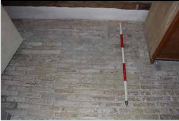
7 Brick paviour floor (eastern service-wing) recorded during the third phase of monitoring, facing south
