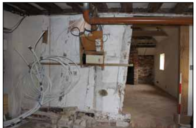
12 North side of the south bay (eastern service-wing) showing studwork with aperture marking the position of a lost stud and truncated sole-plate, facing north
