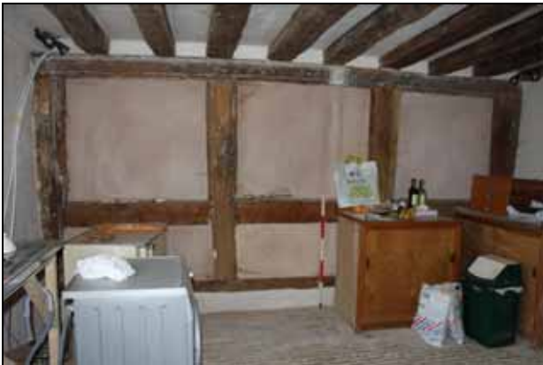
9 South wall of the eastern service-wing showing full extent of frieze windows following the removal of modern fabric, facing south
