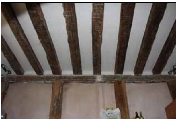
11 Detail of the south wall showing ceiling joists and jetty plate with evidence for diamond mullion windows, facing south
