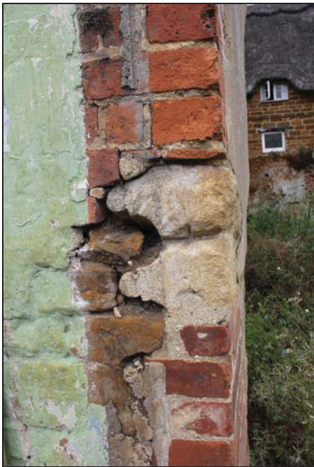
DP 21 Detail of the north-east corner of the house showing reused moulded stone elements, taken from the east
