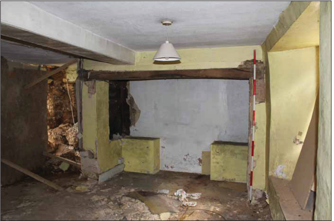
Plate 3 Inglenook fireplace on the east side of Room GF02, taken from the west (DP27)
