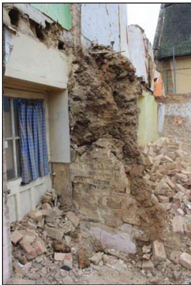
DP 101 Area adjoining the south doorway showing original cob walling with areas of brick repair below, taken during demolition from the east
