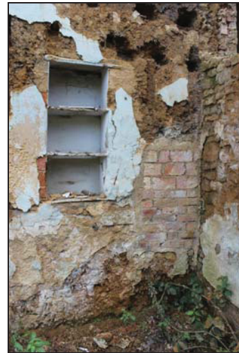
DP 100 Detail of the north elevation (west end) in the area of the former lean-to, taken during demolition from the north
