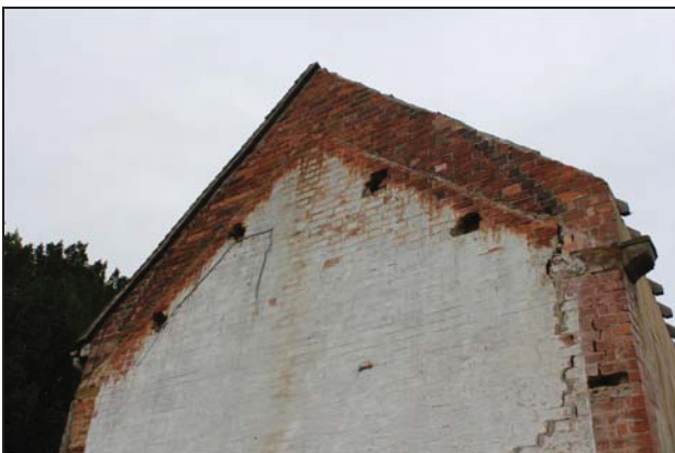
DP 23 View of the east gable of the house at upper level, taken from the east
