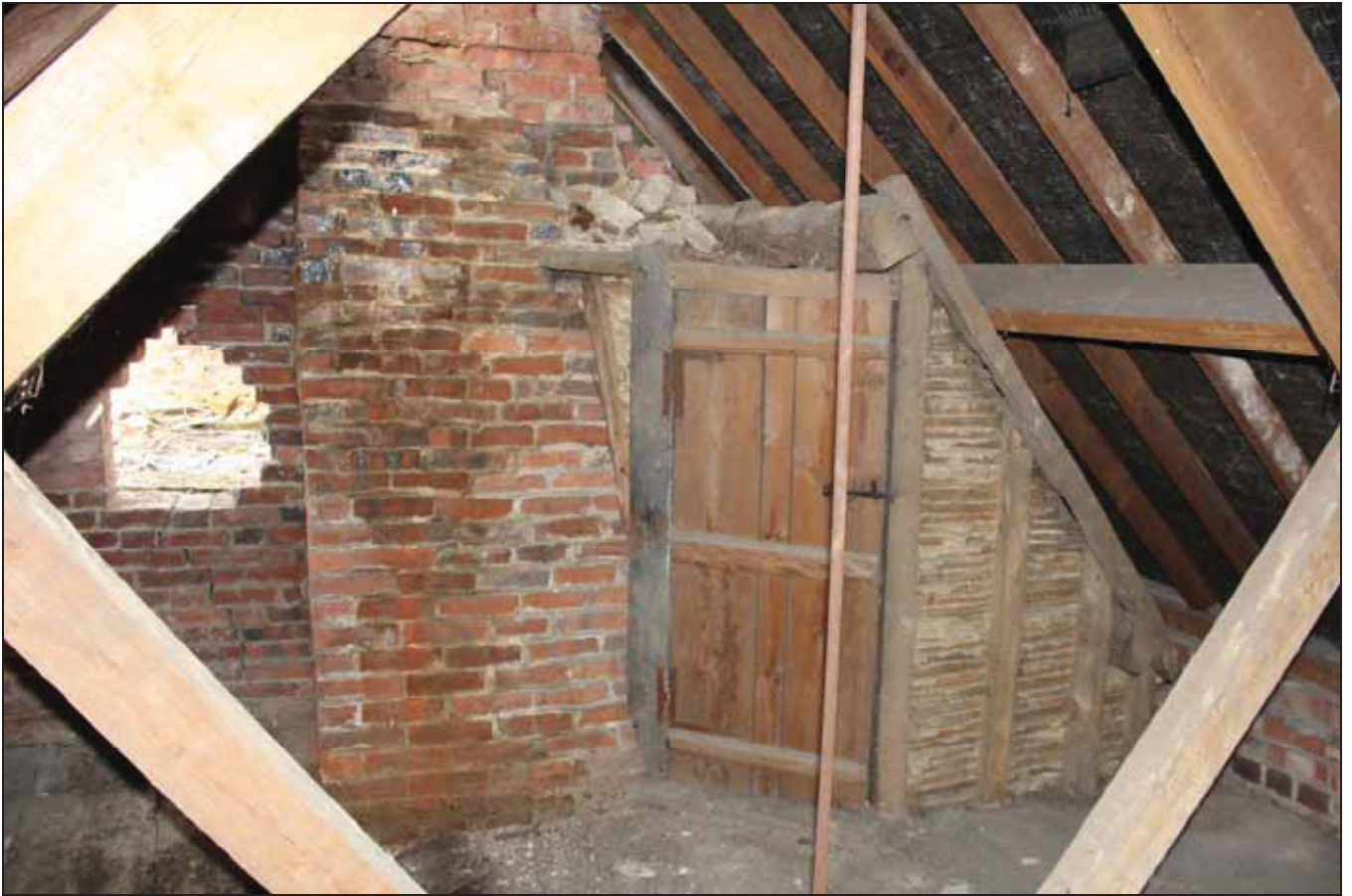
Plate 11 View of the south side of the building at roof level in the centre, taken from the west (DP84)
