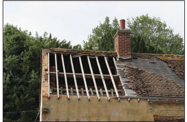
DP 20 North roof pitch of the house showing area of removed tiles, taken from the north
