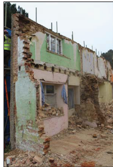
DP 102 South wall exposing mixed cob and stonework construction with later brickwork, taken during demolition from the north-east
