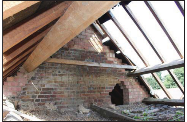
DP 98 View of the east side of the principal chimney stack at roof level, taken during demolition from the east
