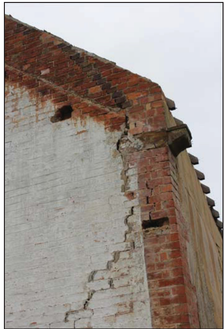
DP 22 Detail of the north-east corner of the house showing reused moulded stone as a projecting corbel, taken from the east
