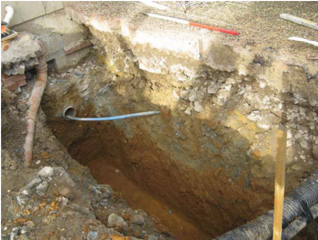
DP 3. Northern part of the foundation trench with Sample section 1. Looking north-west.
