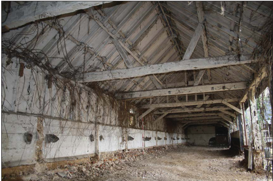
Plate 7 View of Range 3 after the removal of the concrete stall partitions, taken from the west (DP 47)
