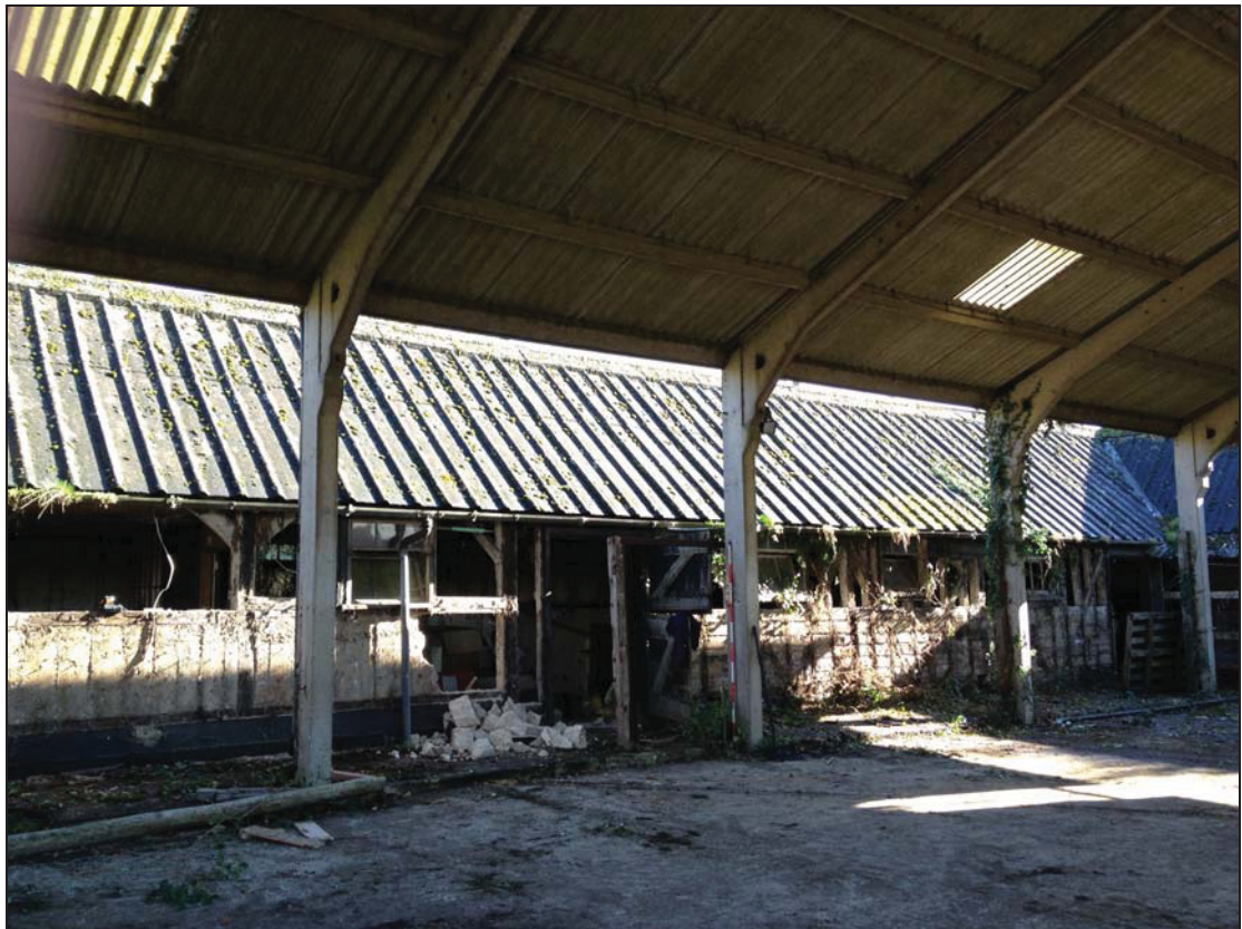
Plate 6 South elevation of Range 3 from within Range 6, taken from the south (DP 10)
