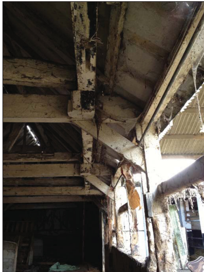
Plate 10 West side of Bays 1 and 2 (Range 4) showing the widening of the range, taken from the north (DP 25)
