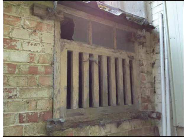
DP 26 Window on the west side of Bay 5 (Range 4), taken from the north-west
