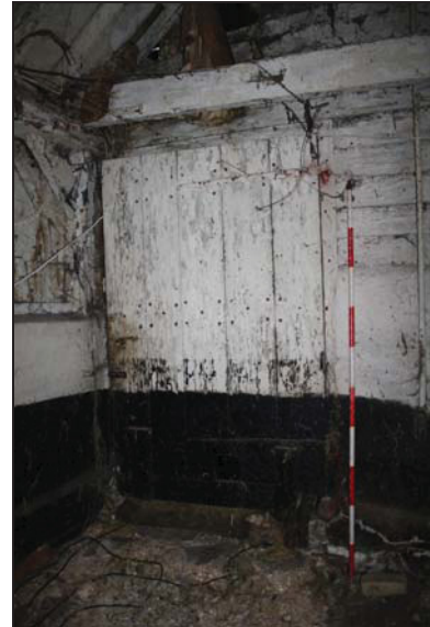
DP 46 18 th century door on the east wall of the barn (Range 1), taken from the east
