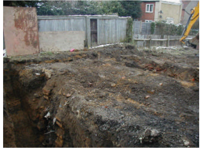
DP 2. Foundation trenches in the western part of the site. Looking north-east.
