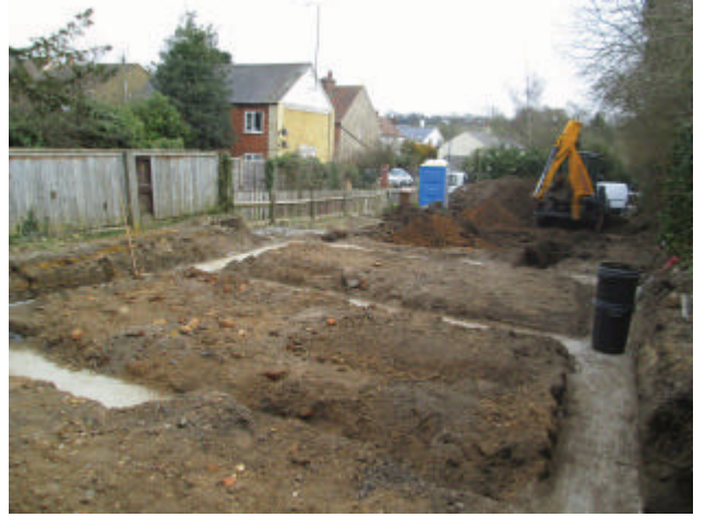
DP 8. Excavation of trenches in the eastern part of the site. Looking east.
