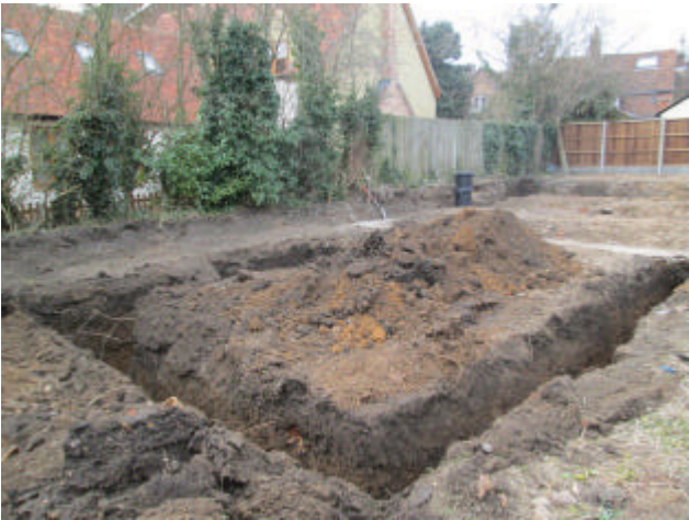
DP 9. Foundation trenches in the eastern part of the site. Looking west-south-west.
