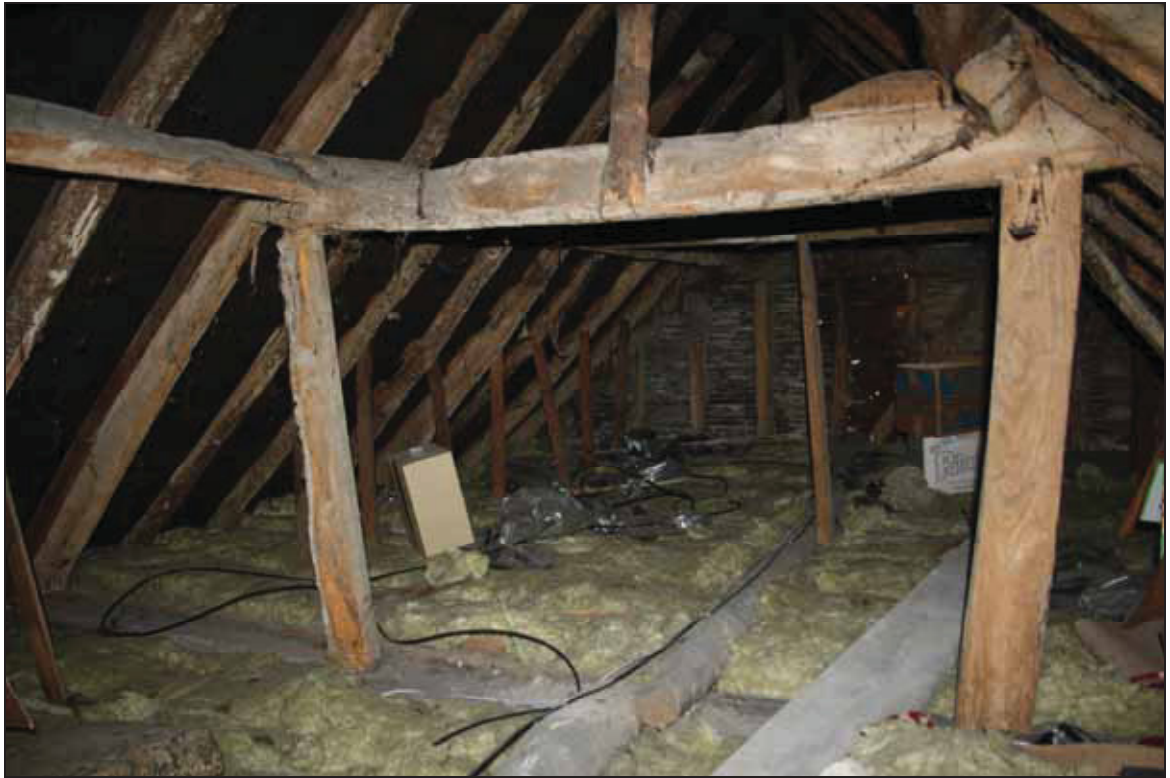
Plate 7 View of the roof structure over the main range, taken from the south (DP 01)
