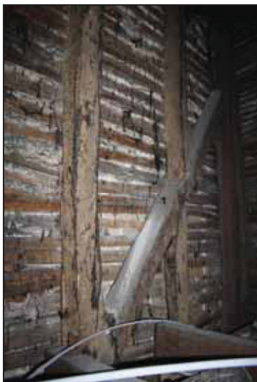
DP 5 East side of the main range showing primary- braced timber-framing, taken from the south-east
