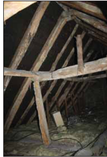
DP 2 View of the roof structure over the main range, taken from the south-east
