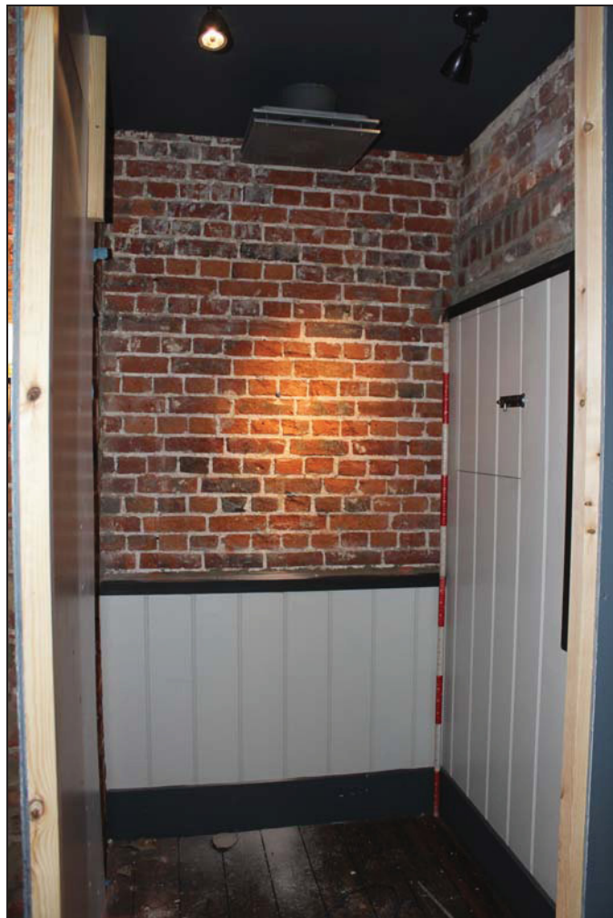
Plate 4 Full-height niche to the east of the chimney stack (GF01, No. 22) showing location of new doorway, taken from the south (DP 2)
