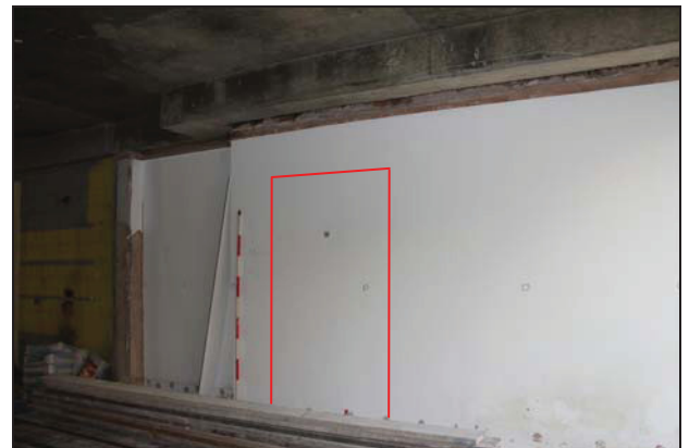
DP 6 South wall of Room GF02 (No. 24) with position of new doorway outlined, taken from the south-west
