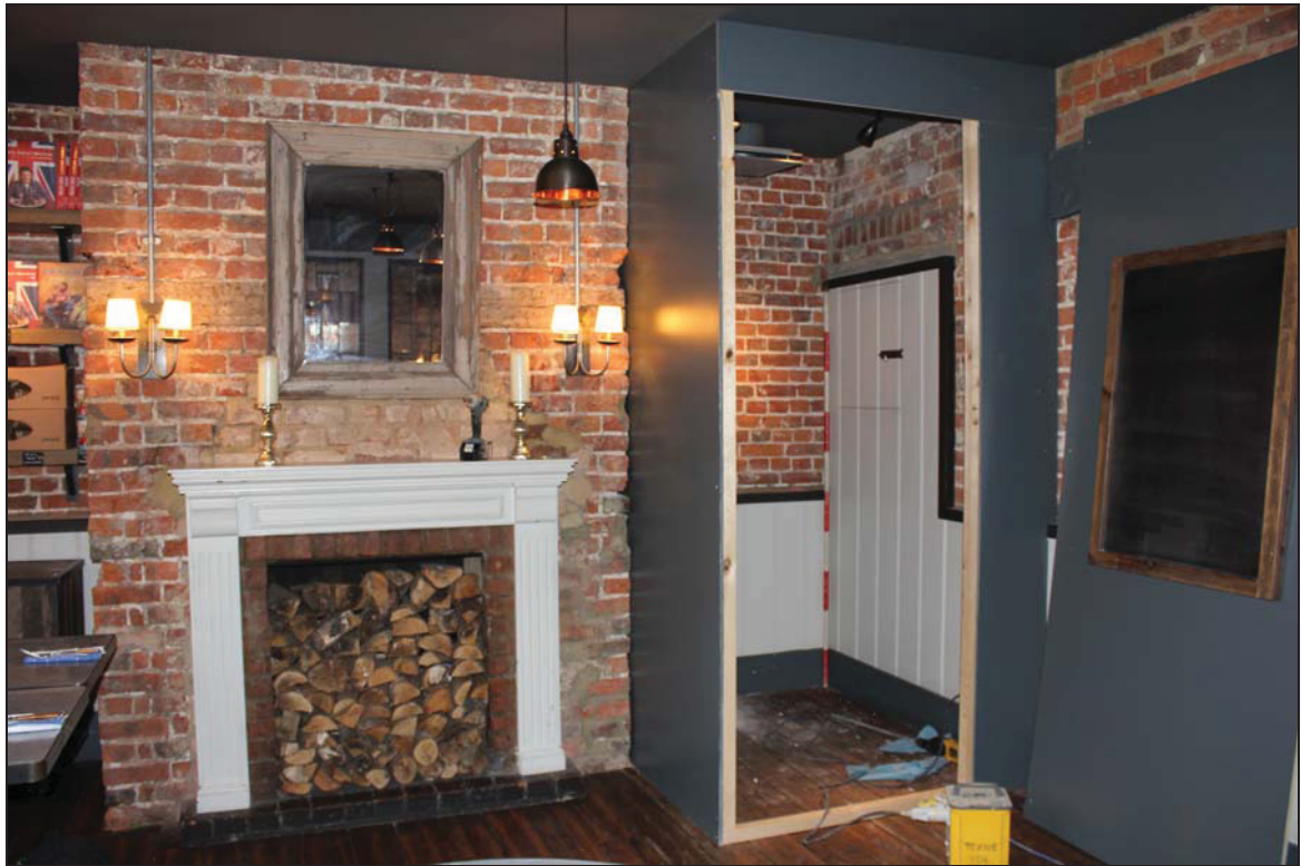
Plate 3 Chimney stack on the north side of Room GF01 (No. 22) with full-height niche to the east where the new doorway is to be located, taken from the south-west (DP 1)
