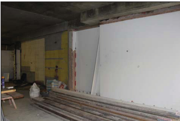
DP 5 South wall of Room GF02 (No. 24) showing modern ceiling and wall cladding, taken from the south
