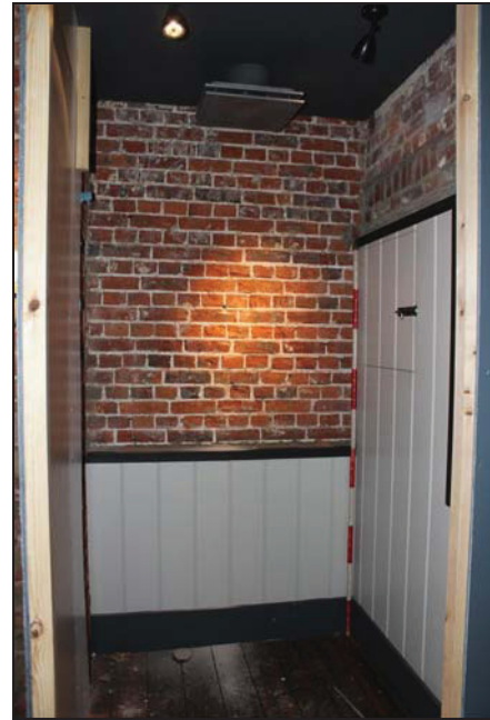
DP 2 Full-height niche to the east of the chimney stack (GF01, No. 22) showing location of new doorway, taken from the south
