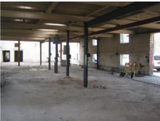
DP 5. Interior of the building before removal of the floor. Looking east-south-east.
