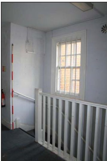
DP 41 First floor landing of the northern staircase (Room FF01), taken from the north
