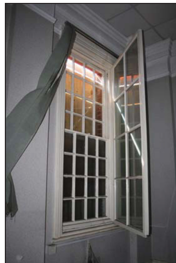
DP 22 Double window system on the south-east side of Room GF07, taken from the north
