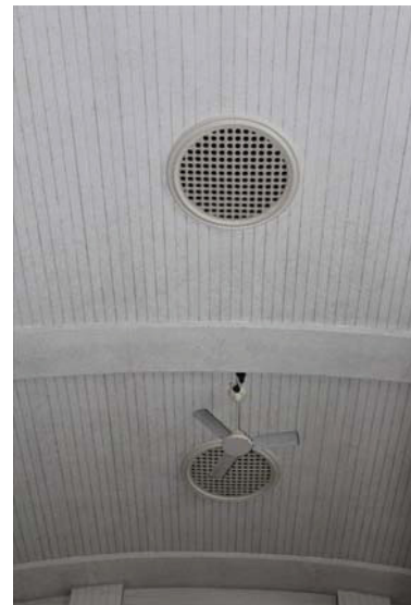
DP 60 Ventilation apertures and fan in the ceiling of Court 1 (GF06), taken from the south-east
