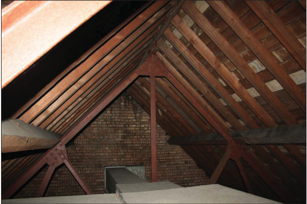
Plate 13 View of the timber and metal roof structure over Court 1, taken from the north (DP 47)
