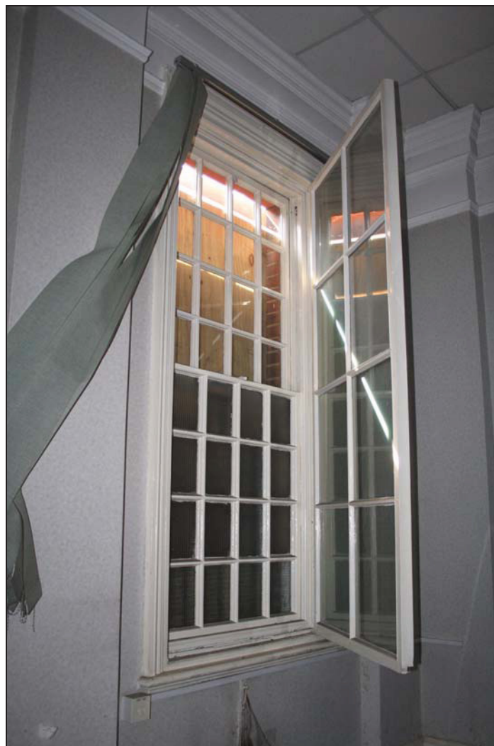
Plate 6 Double window system on the south-east side of Room GF07, taken from the north (DP 22)
