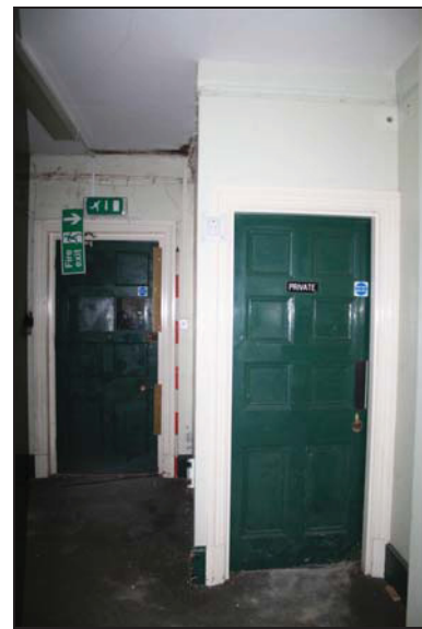
DP 24 Doorways at the southern end of Corridor GF08, taken from the north-west
