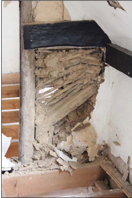
Plate 15 Wattle and daub infill around a brace, north gable, FF02, taken from the south-west (DP 85)
