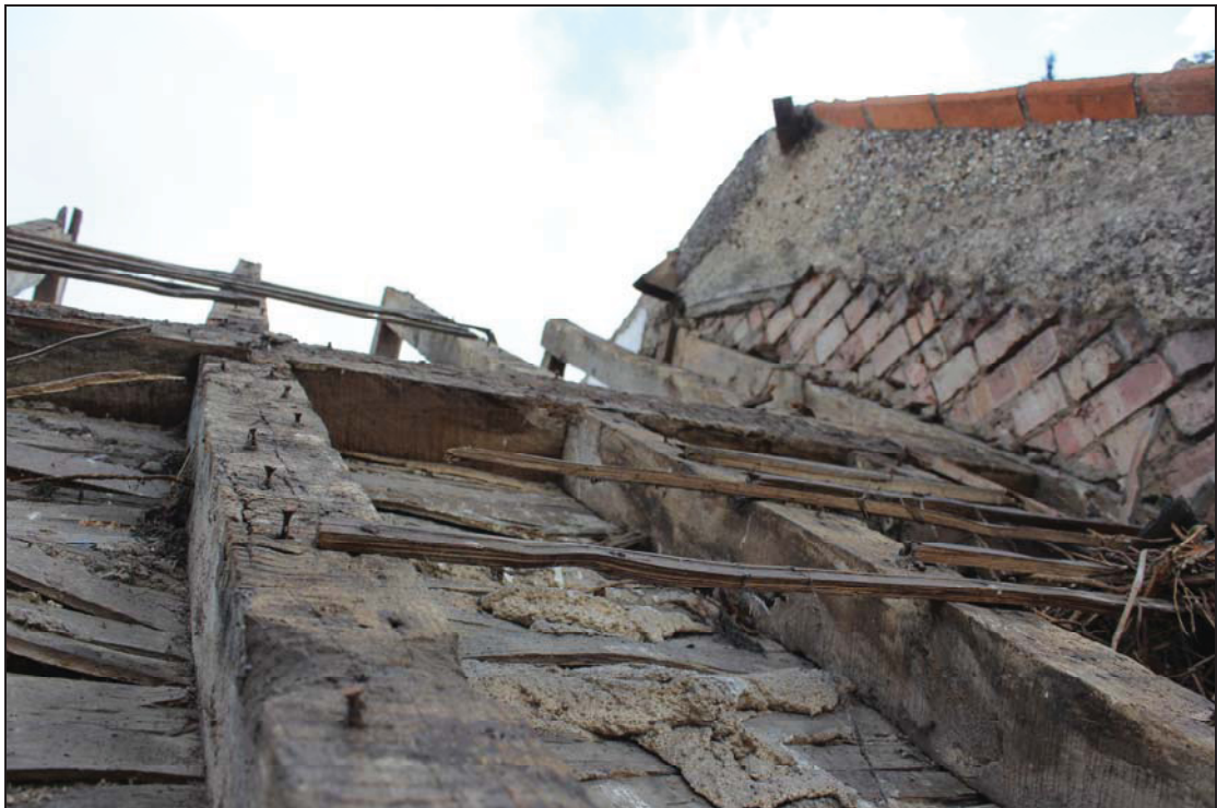
Plate 20 Common-rafters rising above and below the purlin, north-west pitch, taken from the north-west (DP 92)
