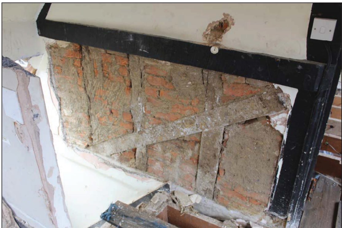
Plate 14 Timber-framing infilled with brick at the bay division, FF01, taken from the south-east (DP 93)
