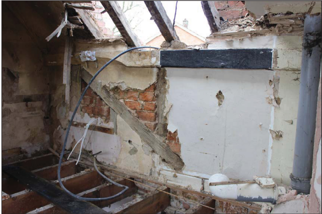
Plate 13 Primary braced studwork with brick infill to north-west elevation, FF01, taken from the north-east (DP 83)
