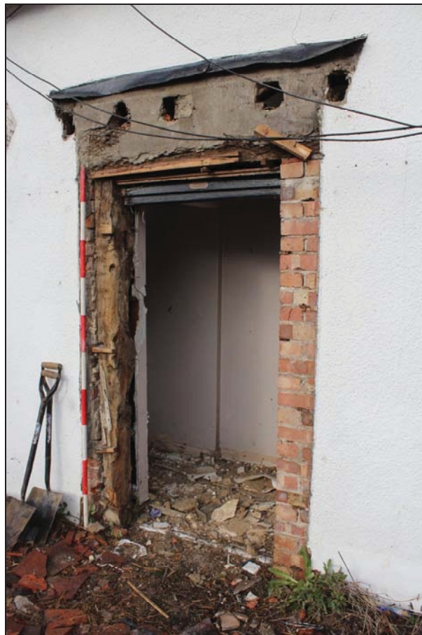
Plate 4 Original timber at the bay division acting as door jamb, south-east elevation, taken from the east (DP 68)
