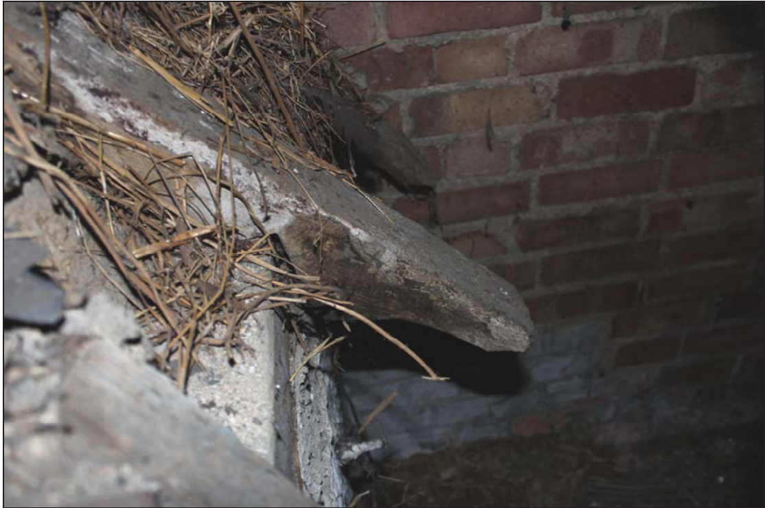
Plate 19 Original rafter feet preserved within pent-roofed extension seen from FF05, taken from the north-east (DP 55)
