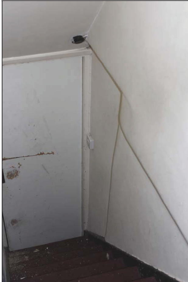
Plate 11 Stair vestibule, the junction between historic core and rear pent-roofed extension visible in the wall, FF01, taken from the south-east (DP 43)
