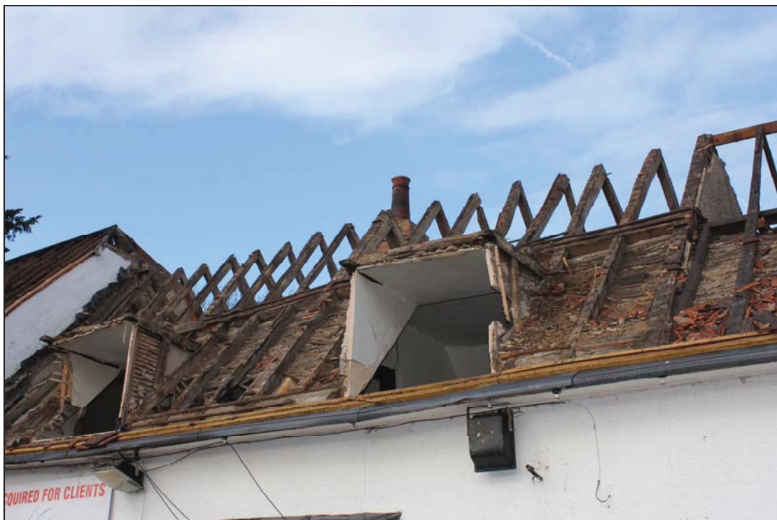
Plate 18 Roof structure above two-bay historic core of the building, south-east pitch, taken from the east (DP 67)
