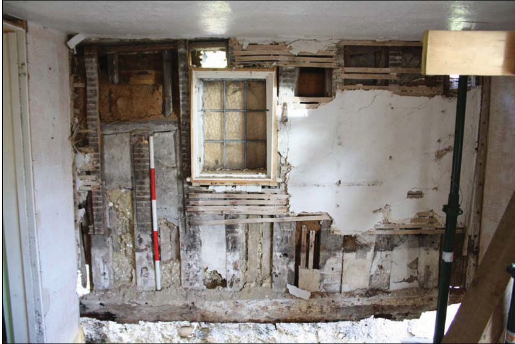
Plate 7 Soft stripping of the walls in Room 3, revealing early 17 th century window and timber-framing, taken from the south-east (DP 21)
