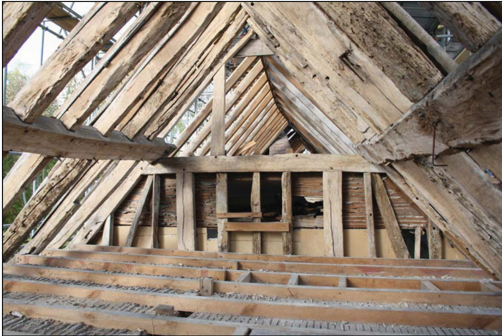
Plate 15 Internal roof space above the kitchen range, taken from the south-east (DP 68)
