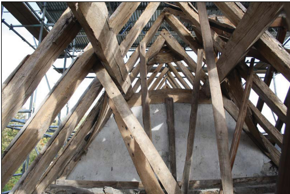
Plate 6 Internal view of the roof above the cross-wing, south bay, taken from the south-west (DP 75)
