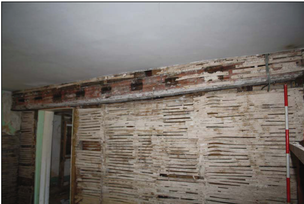
Plate 8 Central joist between Rooms 3 and 4 covered in red pigment with redundant mortices for common-joists, Room 4, taken from the south (DP 18)
