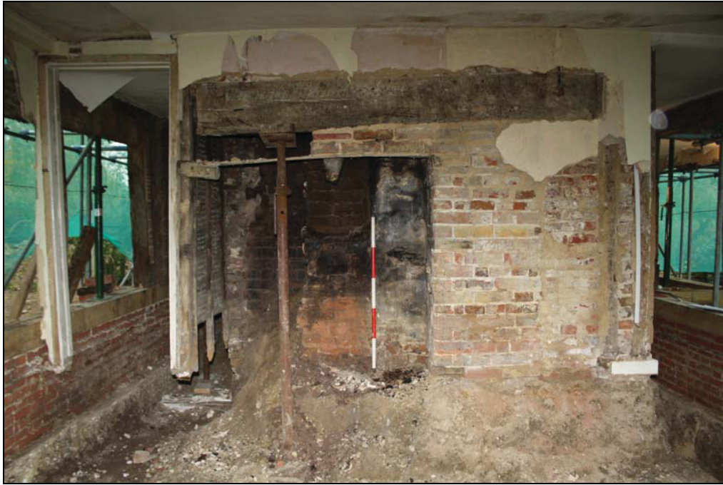
Plate 11 Chimney stack, fully exposed, ground floor, Room 1, taken from the south-east (DP 90)
