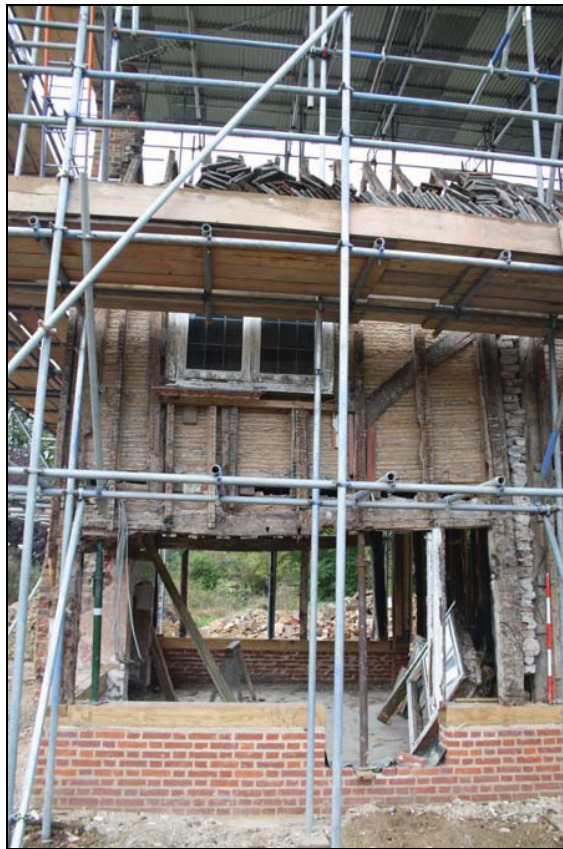
Plate 14 The kitchen bay, north elevation, fully exposed, taken from the north-east (DP 34)
