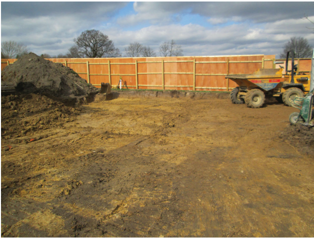
DP 9. Car par extension area to the north of the site. Looking north.
