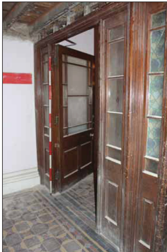
Plate 20 Glazed and panelled partition to a small lobby and external access, GF09, taken from the south-east (DP 170)
