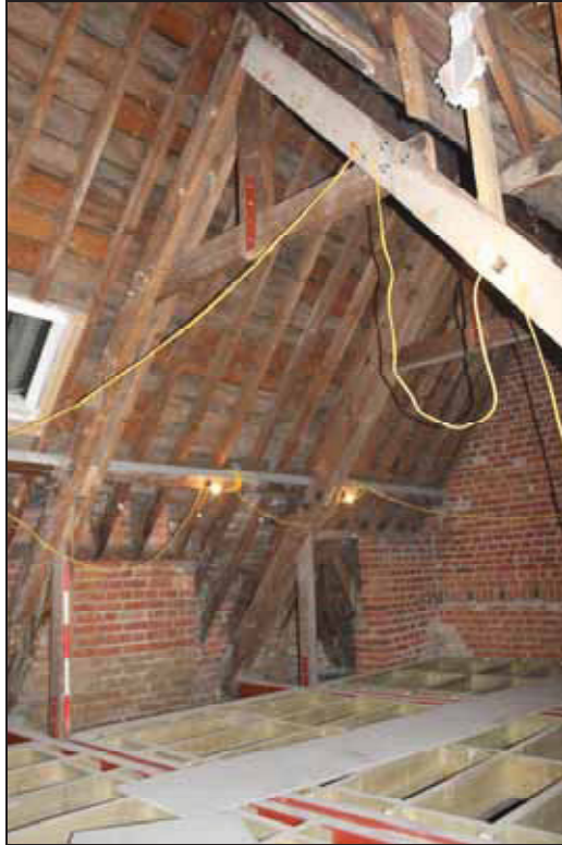
Plate 27 Roof space above the east gable of the main house, SF09, taken from the west (DP 322)
