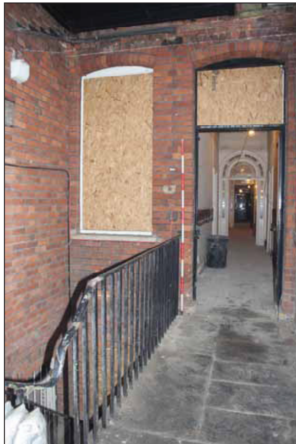
Plate 8 Side entrance to the service range, north-east elevation, taken from the north-east (DP 96)
