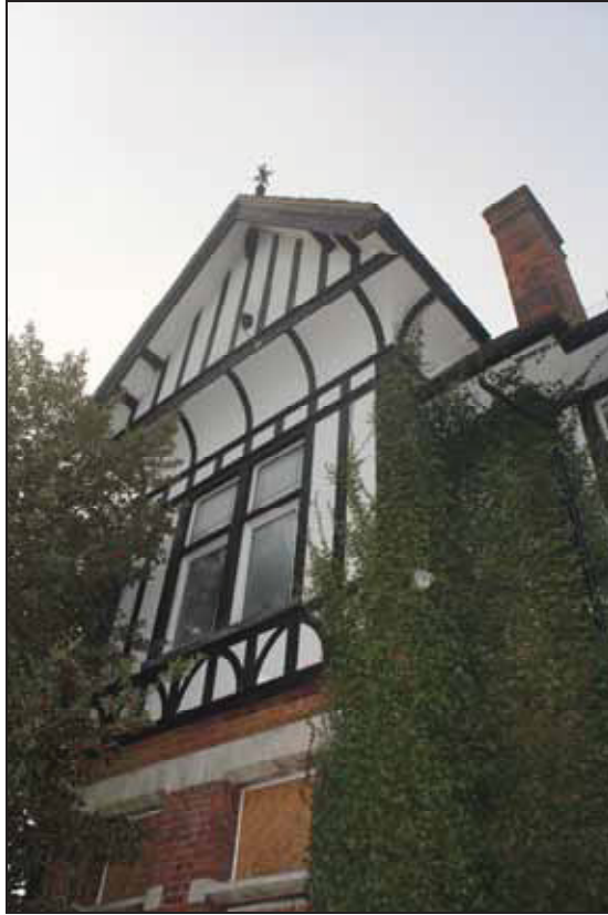
Plate 3 Upper decorative timber framing with jettied gable to south-east elevation, taken from the east (DP 74)
