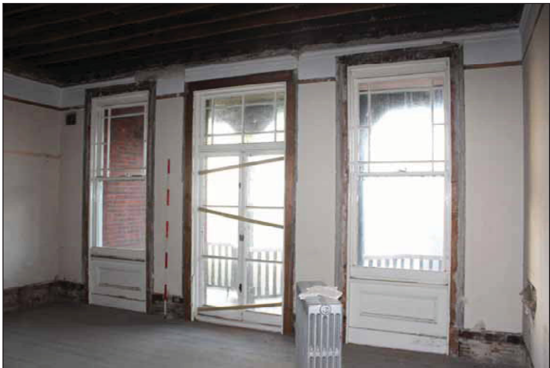
Plate 24 Central glazed access to the balcony, FF04, taken from the north-east (DP 248)
