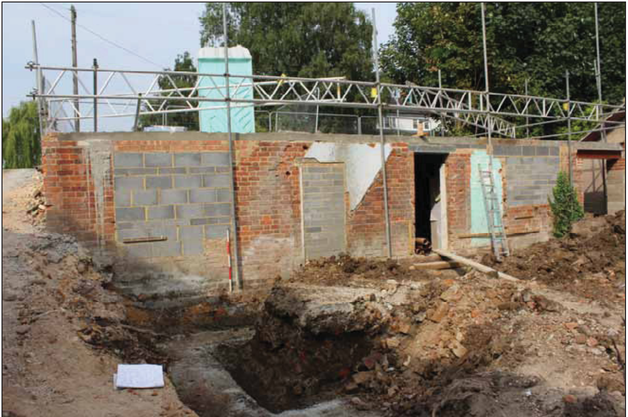
Plate 4: East elevation of the surviving lower ground floor level, taken from the east (DP 13)
