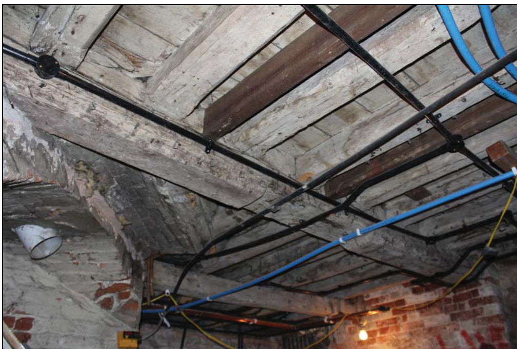
Plate 8 Ceiling to the basement formed of large chamfered central joist and chamfered common-joists with lamb tongue chamfer stops, BF01, taken from the west (DP103)
