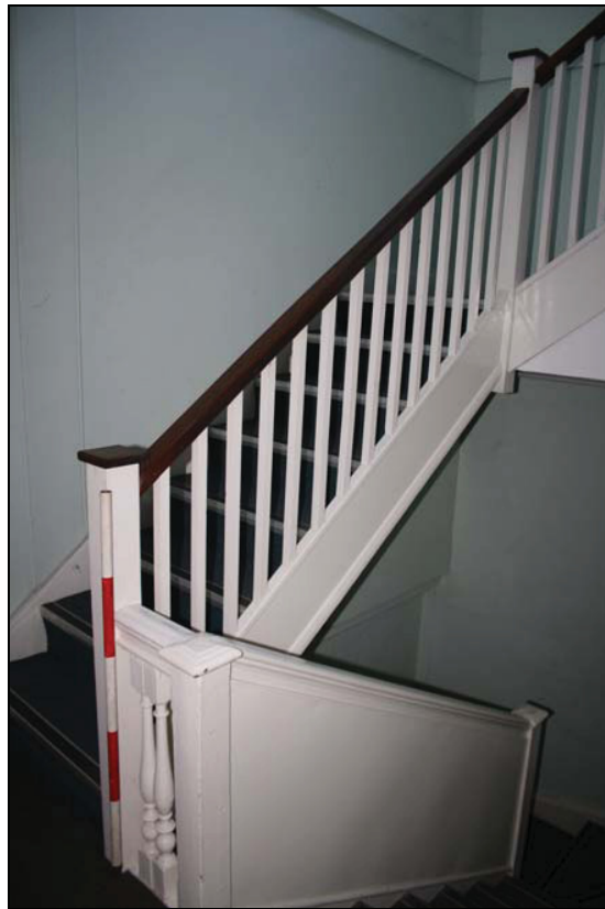
Plate 16 Staircase rising to the attic floors, FF01, taken from the east (DP43)
