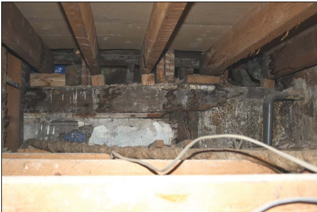
Plate 20 Timber-framing of the adjoining property seen in the roof space above FF08, taken from the south-east (DP58)
