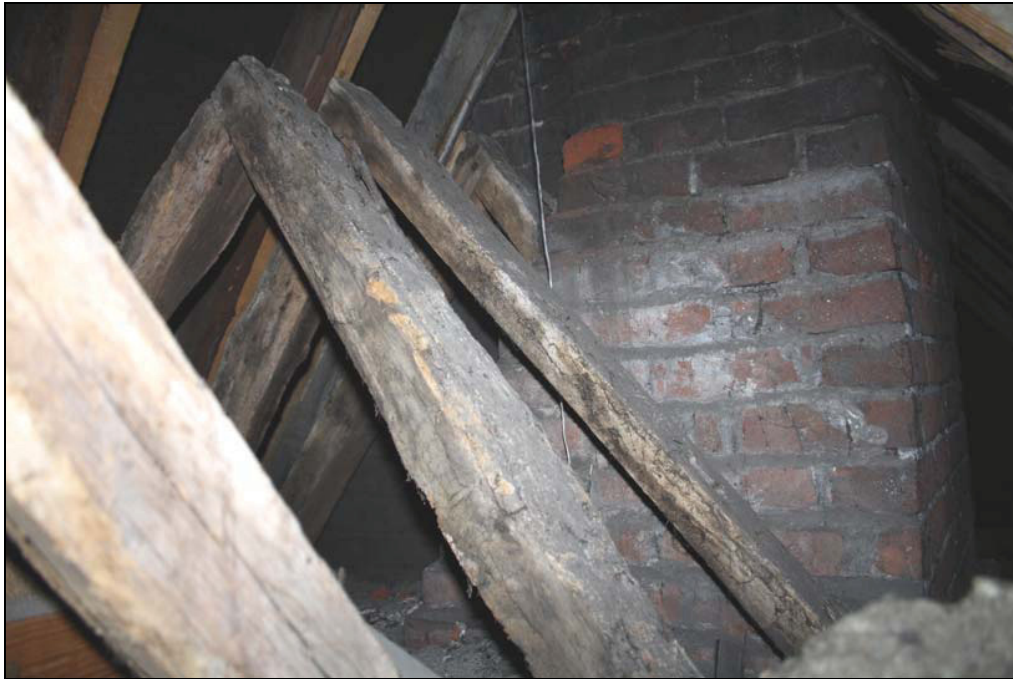
Plate 23 Short span of rafter couples rising between the hip of the roof and the chimney stack superimposed by the later extension to the north, taken from the east (DP73)
