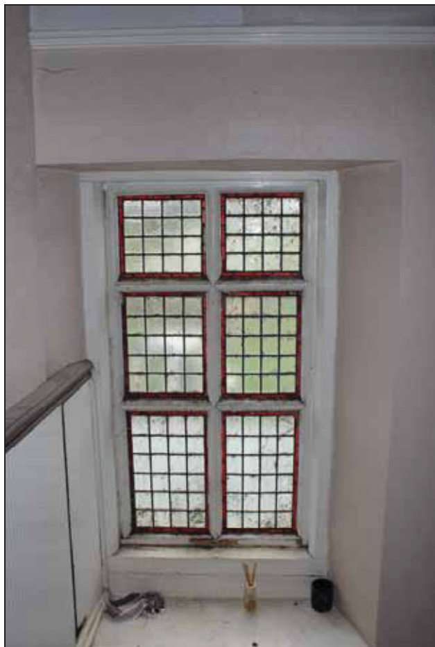
Plate 6 Original stair light in the west range at first floor level, taken from the south (DP 44)
