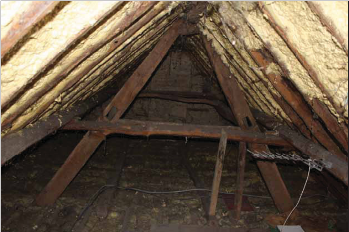
Plate 7 Roof space above the main range showing the original central truss, taken from the east (DP 50)
