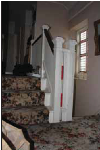
43 Staircase in the west range at first floor level (FF07), taken from the east
