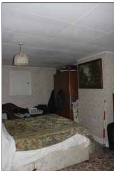
47 North side of Room FF01 in the main range, taken from the south
