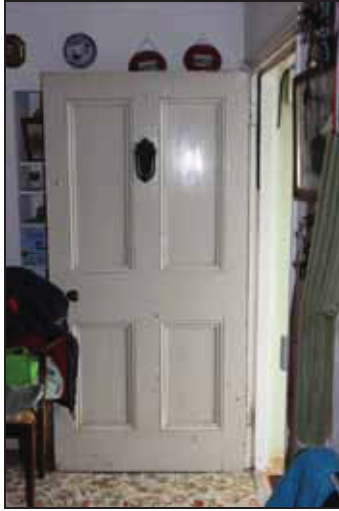
37 19 th century four-panelled front door on the south side of the main range (GF01), taken from the west
