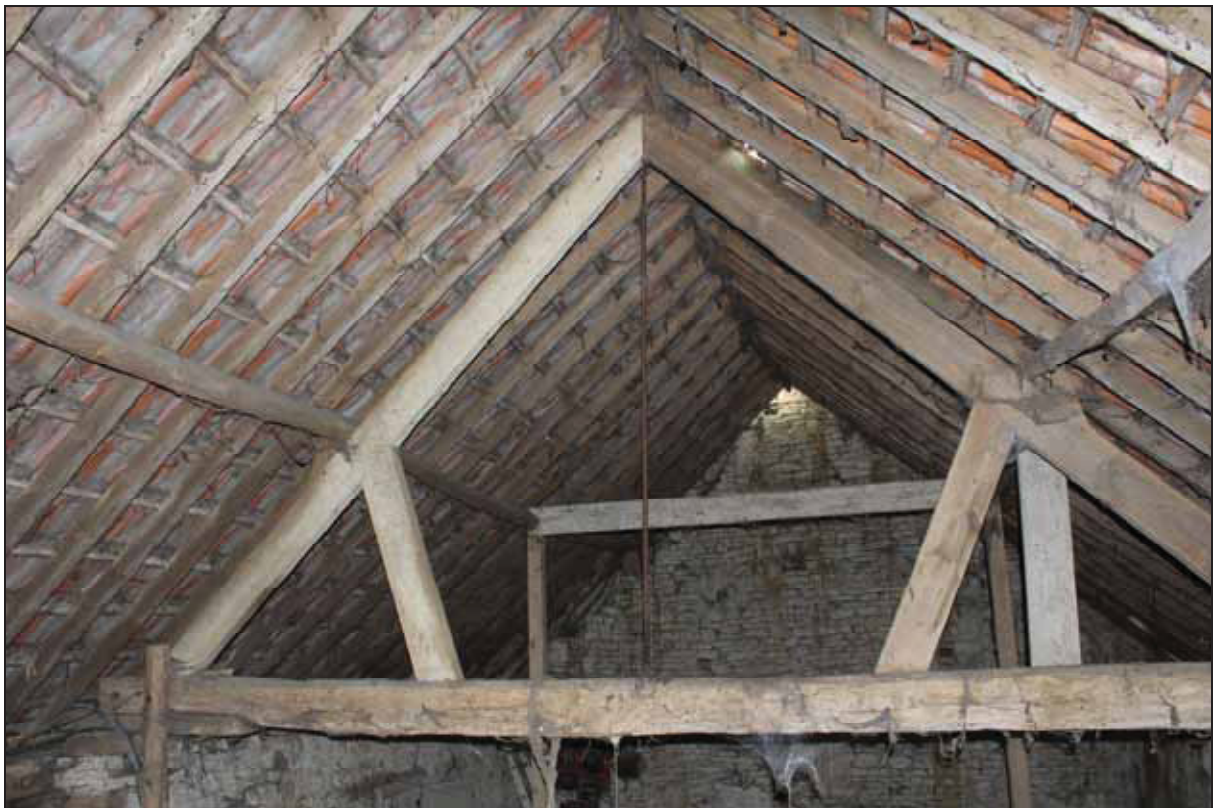
Plate 10 View of the roof structure of the barn, taken from the east (DP 31)
