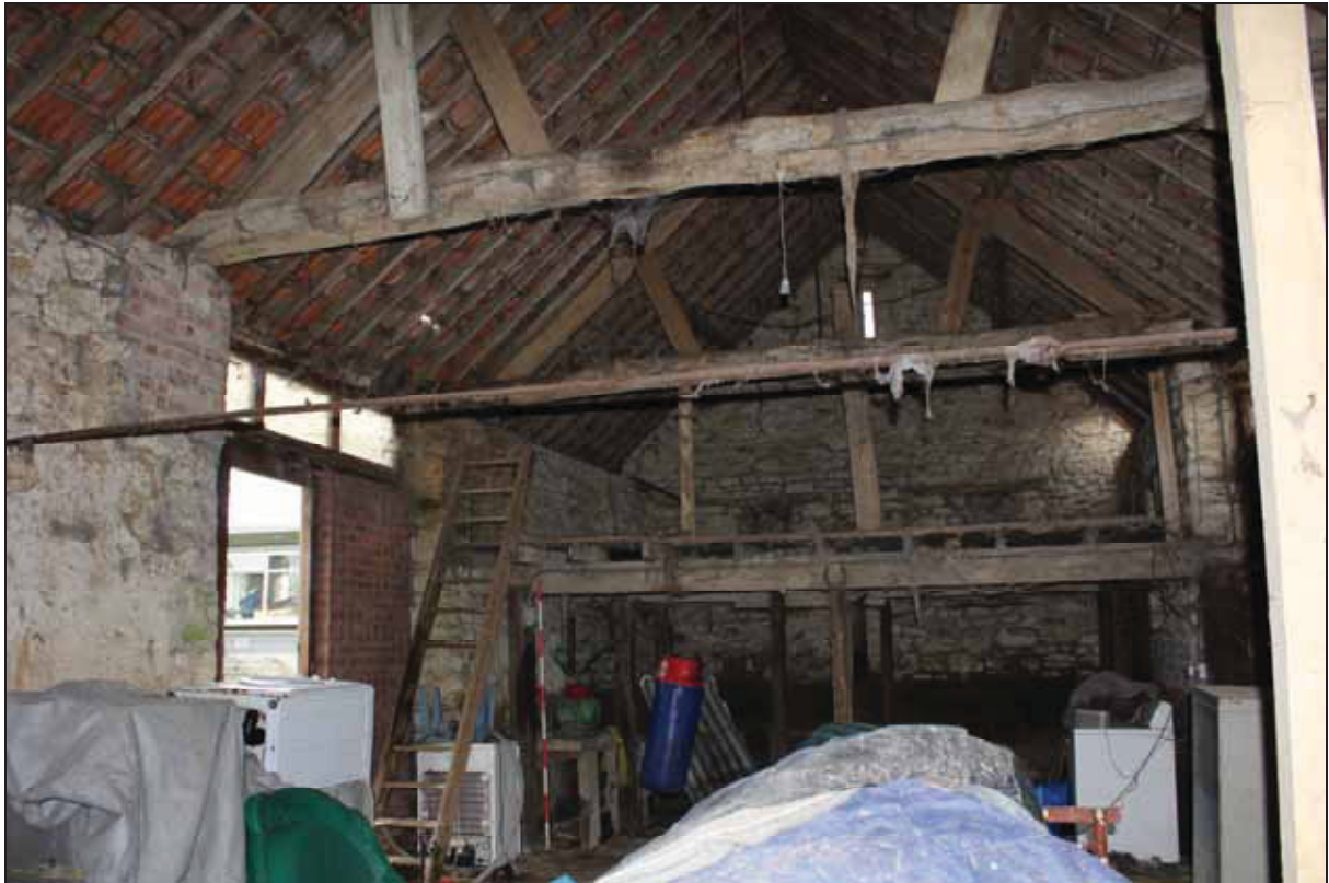
Plate 9 Interior of the barn showing inserted first floor in the east bay and threshing door on the north, taken from the west (DP 50)
