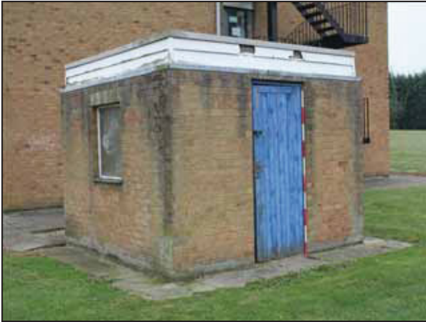
13 Sub-station building at the western end of the rear range. Taken from the north-west.
