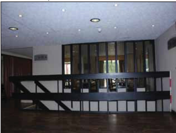
23 Shot of staircase from ground floor to lower floor of rear range, also showing glazed panels, taken from the north-east.
