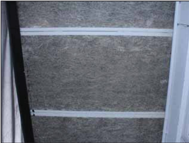
33 Soffit view of the roof over the northern wing of the main frontage, showing fibre glass panels and aluminium supports, taken from the north-east.
