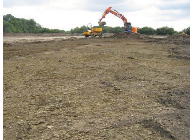
DP 14. Central part of the grass pitches area during the excavation. Looking north-east.
