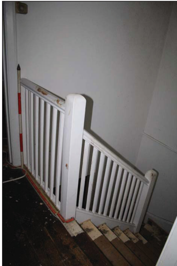
Plate 4 View of the staircase at first floor level (FF01), taken from the south (DP 15)
