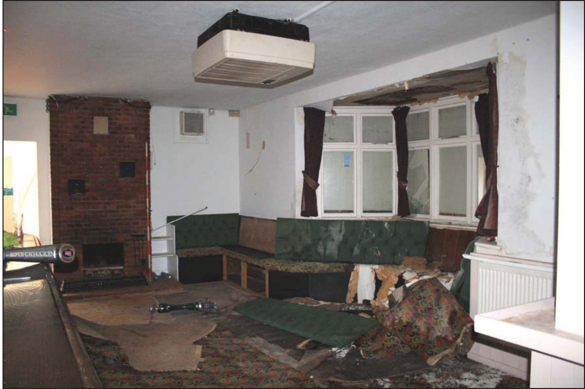
Plate 3 Main public bar area (GF01) with fireplace and bay window, taken from the north (DP 08)
