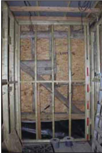
DP 19 View of the south wall in the area of the former aperture (Area 1: west end), taken from the north
