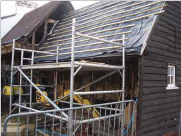
6.7 East side of the building following removal of the pan-tiles as well as the timber-framing on this side.
