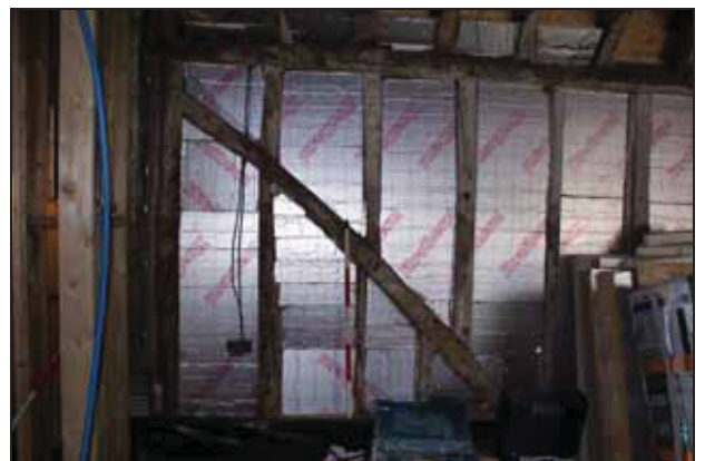
DP 12 Detail of the timber-framing on the west wall (Area 2: south end), taken from the east
