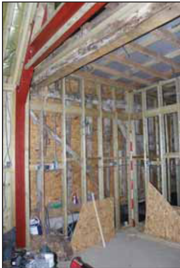
DP 21 View of the south wall with east binding joist/tie-beam visible above (Area 1), taken from the north
