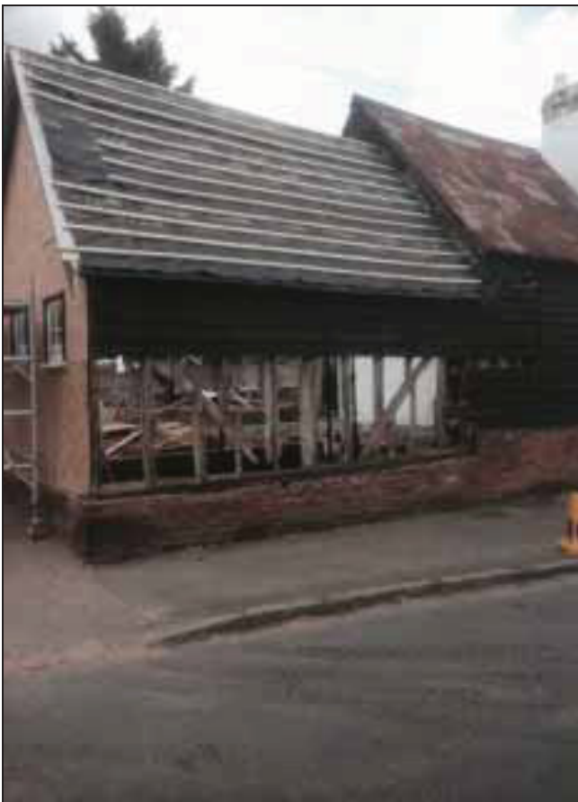
6.5 West side of the building. The weatherboarding has been partially removed though the underlying timber-framing is visible above the sole-plate and dwarf wall.
