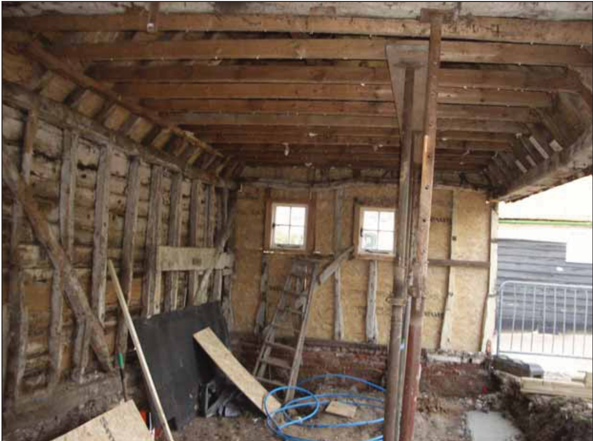
6.15 Interior of the north unit showing timber-framing of the west and north walls. Note the weatherboarding to the rear on the left.
