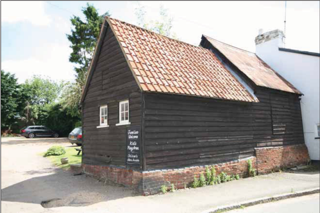
6.1 View of the west side of the assessment building prior to the start of works. Note the straight joint in the brickwork and varying roof cladding.
