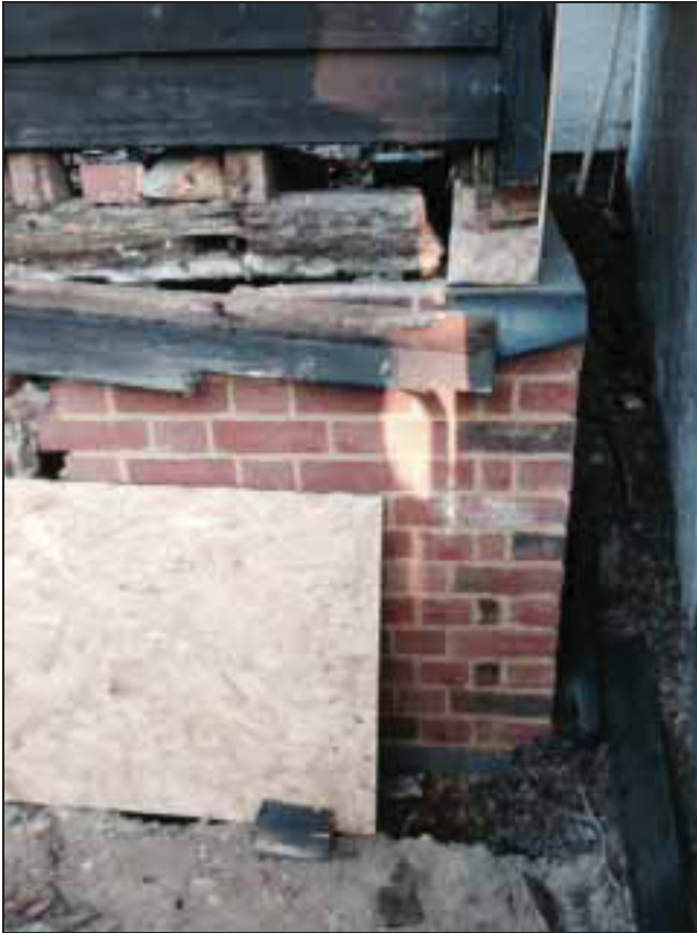
6.3 Detail of the south-west corner of the building. The dwarf wall has been replaced but the original sole-plate is visible.
