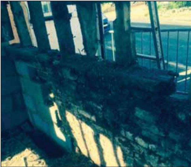
6.10 West side of the south unit showing surviving sole-plate with the corner below rebuilt in blockwork
