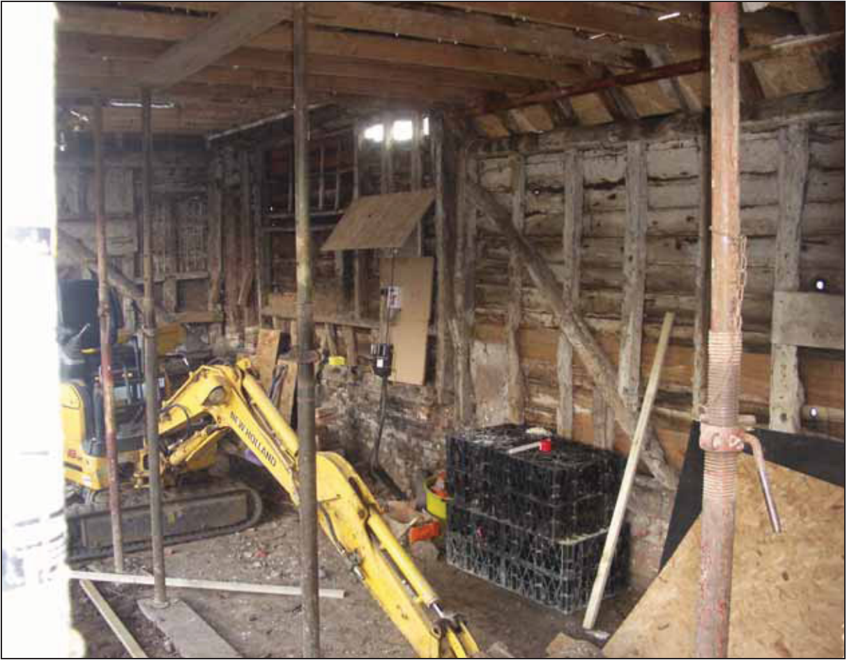
6.14 Interior of the building during planned works showing primary-braced studwork on the right with the former apertures visible to the rear.
