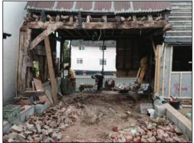
6.8 East side of the building (south unit) following removal of the early 20 th century pent-roofed element and during construction of the extension.
