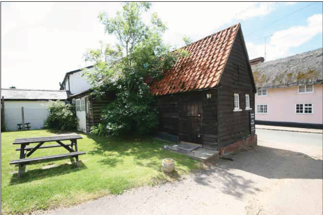
6.2 View of the east side of the assessment building prior to the start of works. The early 20 th century rebuilding of the east range is visible enclosed by typical double garage doors.
