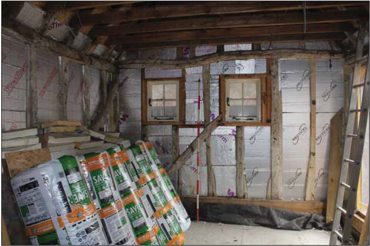
Plate 5 Timber-framing exposed on the west and north walls (Area 2), taken from the south (DP 6)
