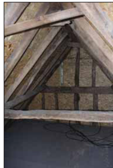
DP 24 View of the roof structure over Area 1, taken from the north
