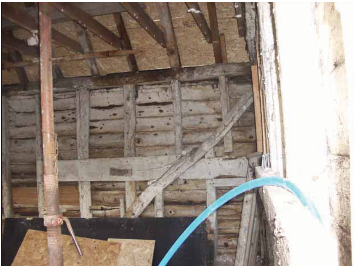
6.17 Detail of the west wall of the north units showing studwork with later applied brace.
