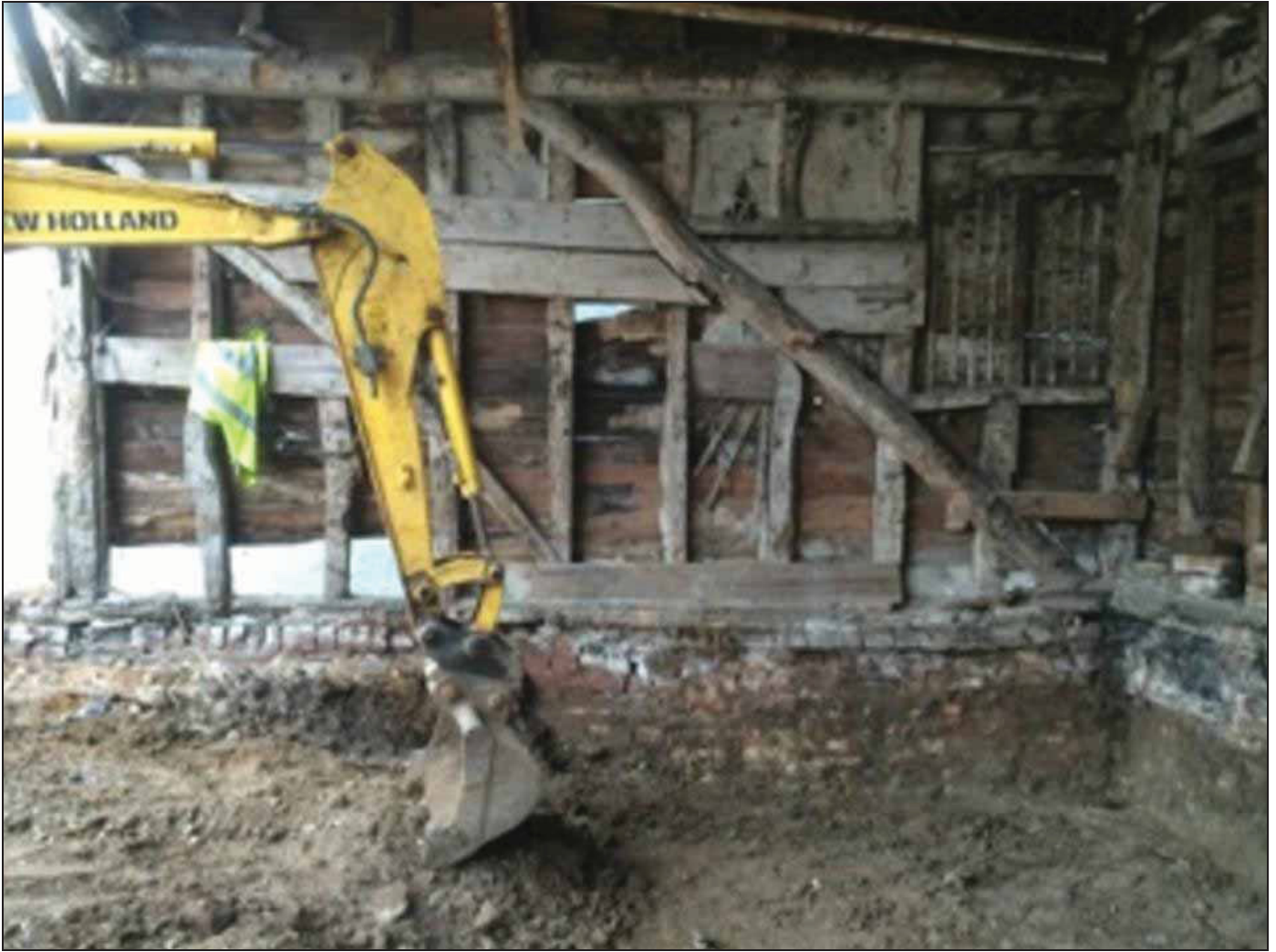
6.18 South wall of the south unit taken during floor reduction works. The former aperture is visible on the right. What appears to be sections of historic lath and plaster are visible infilling the gaps between the studs.
