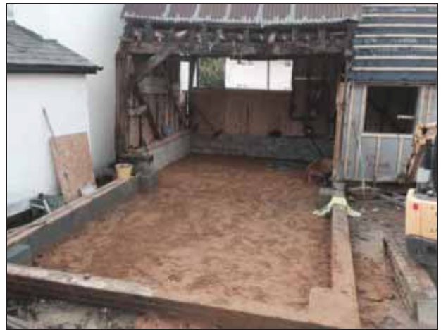
6.13 East side of the building (south unit) following removal of the early 20 th century pent-roofed element and during construction of the extension.
