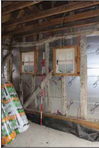
DP 7 Section of the north wall (Area 2) showing casements serving the former WCs, taken from the south-east
