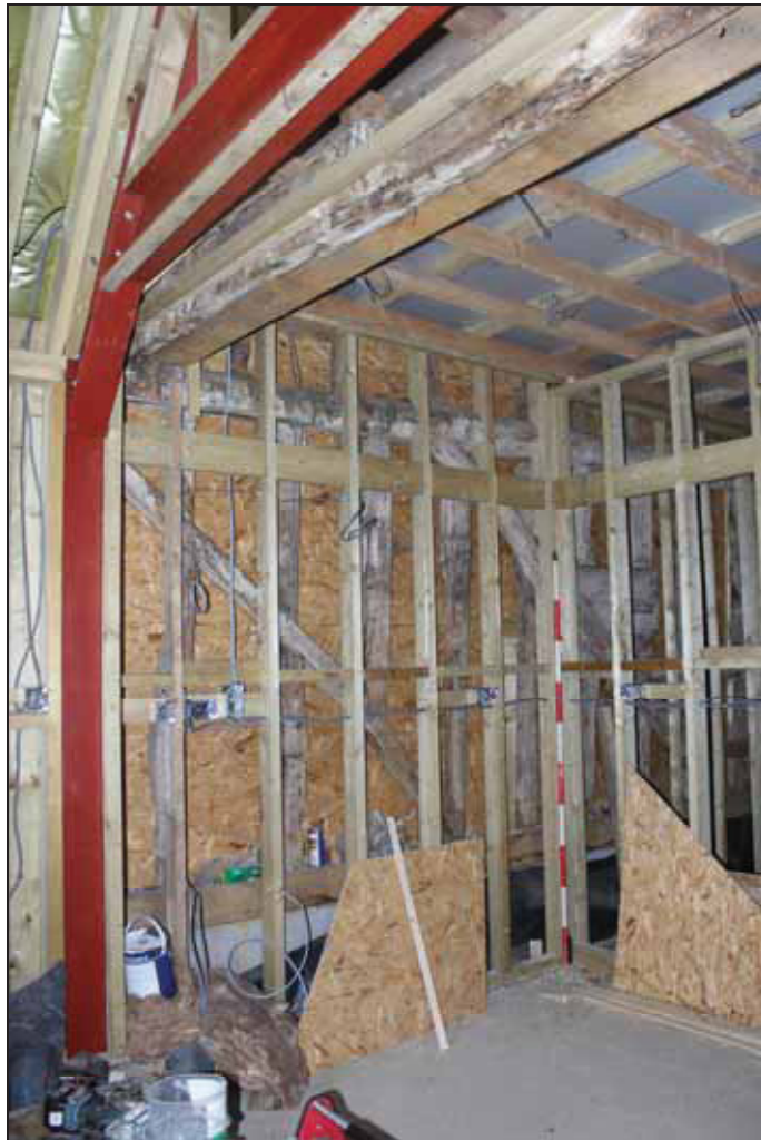
Plate 3 View of the south wall with east binding joist/tie-beam visible above (Area 1), taken from the north (DP 21)
