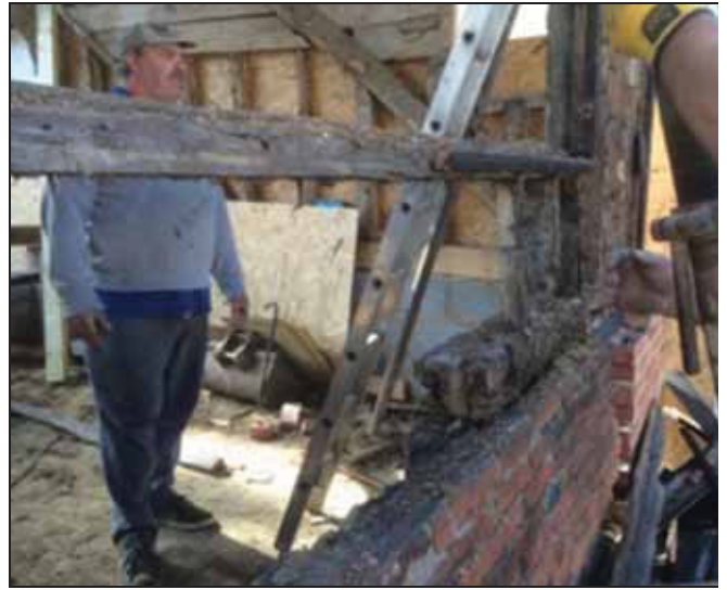
6.11 West side of the south unit showing fragment of sole-plate over the early brickwork of the dwarf wall
