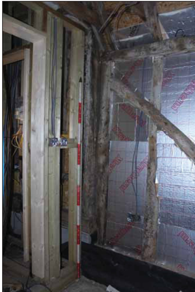
Plate 2 Detail of the junction between the two units showing adjacent posts marking the structural divide, taken from the north-east (DP 14)
