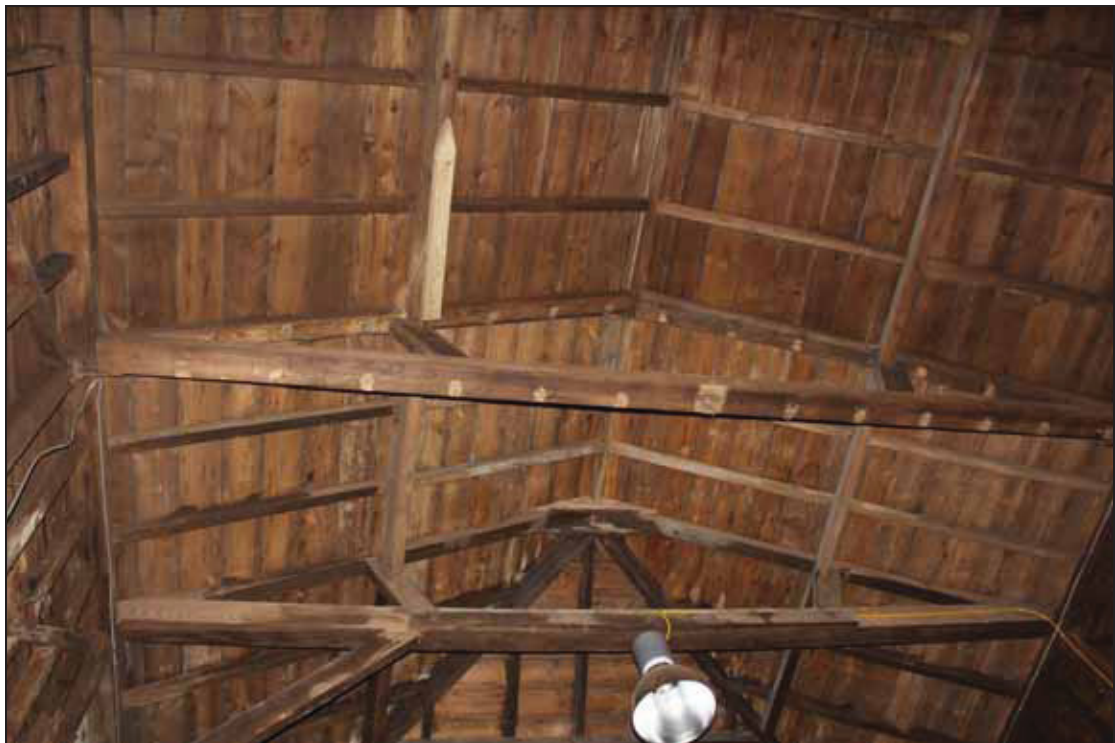
Plate 4 Roof of Bay 5 showing redundant mortices in the tie beam and principal rafter, which was once partitioned (DP 06)
