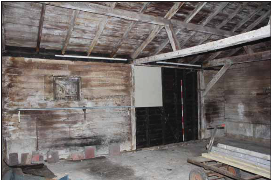
Plate 8 North wall of the Garage showing later inserted panel, perhaps once a door, now painted with black preservative, taken from the south (DP 20)
