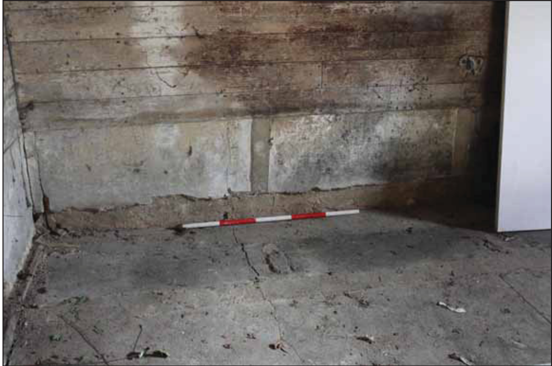
Plate 7 Original stall partitions on the east wall of the Garage, the cement infill represents the partition and the concrete dwarf wall would have once supported a trough, taken from the west (DP 16)
