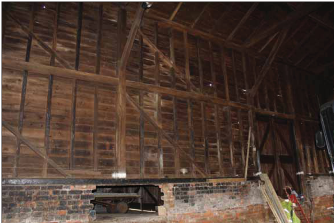
Plate 2 East side of the building showing loading door in Bay 3, taken from the north-west (DP 13)
