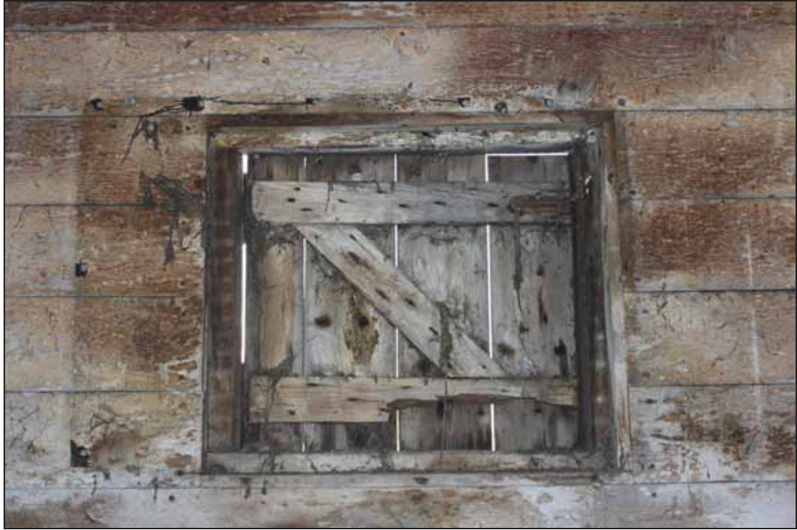
Plate 9 Small ledged and braced shutter on the north wall of the Garage, taken from the south (DP 15)
