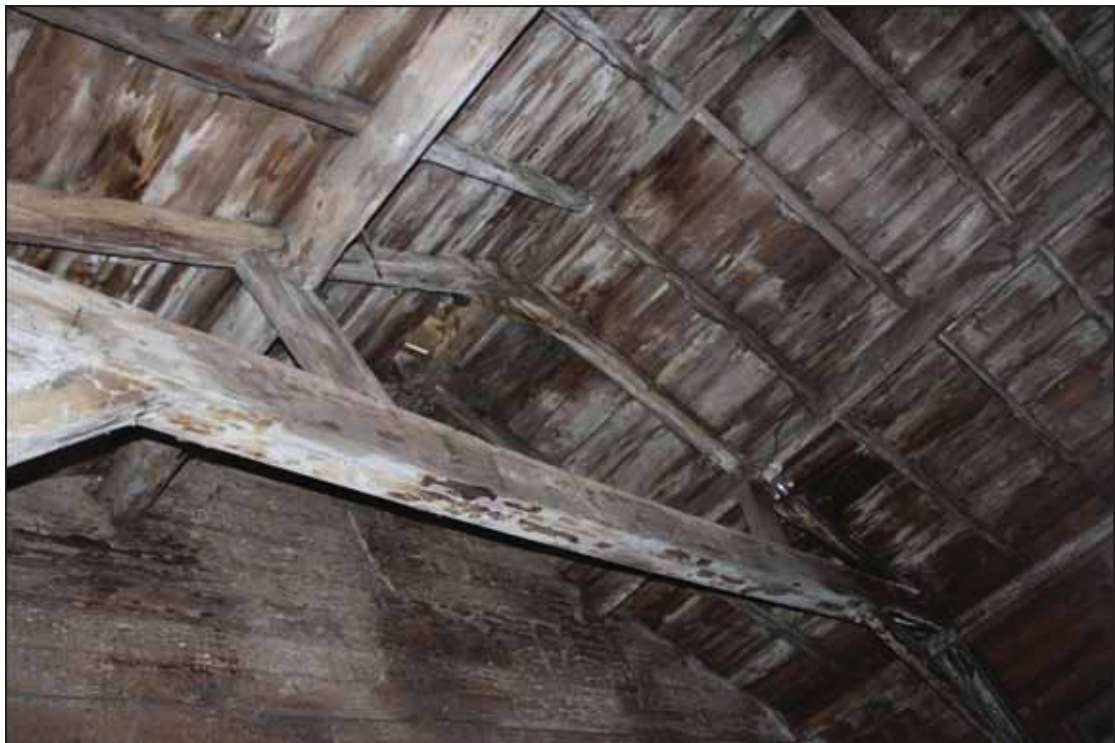
Plate 6 Roof structure in the Garage showing the louvre at the east end over the original animal pens, taken from the west (DP 22)
