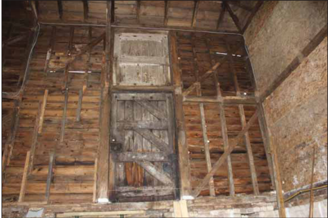
Plate 5 East side of Bay 5 showing conventional door, of some age, and pitching door in the upper register (DP 09)
