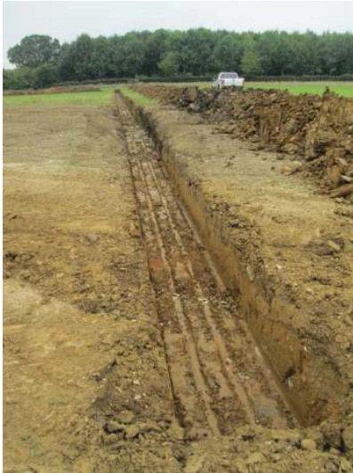
DP 9. The cable trench within east part of solar farm. Looking north.
