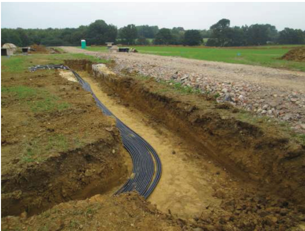
DP 15. Trench for new inverter in central part of solar farm. Looking north-north-east.
