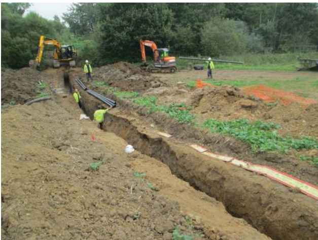
DP 5. Central section of power grid connection trench during groundworks. Looking east-south-east.
