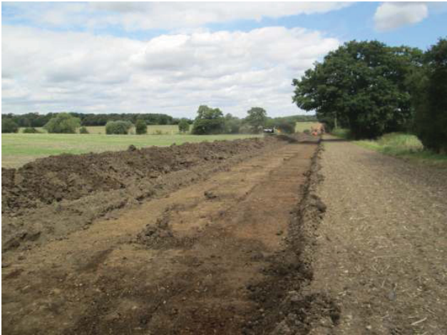
DP 1. South section of power grid connection trench. Initial strip of topsoil. Looking north-east.
