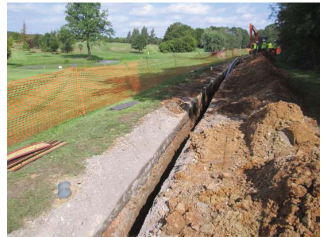
DP 6. Central section of power grid connection trench within golf course. Looking north-east.
