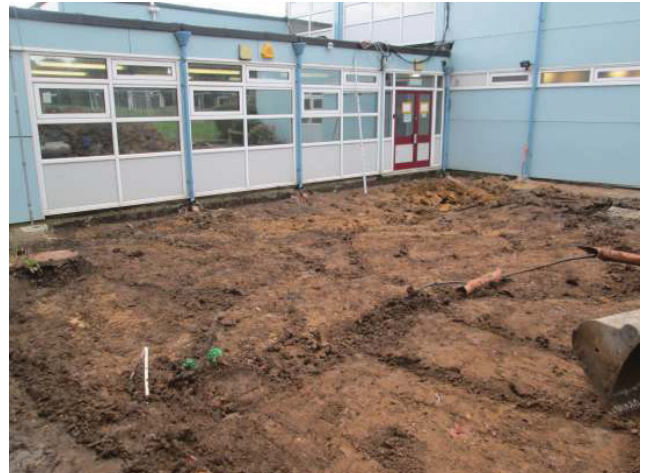
DP 2. East part of the site after initial strip of the soil. Looking south-east.
