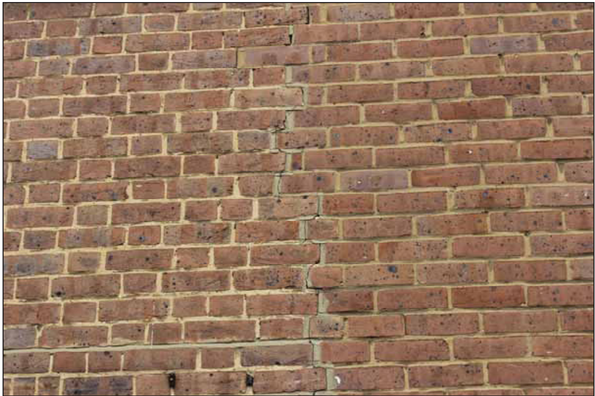
Plate 8 Sample of brickwork on the east side of No. 26-28 showing earlier brickwork to the west and modern brickwork to the right, taken from the east (DP 36)
