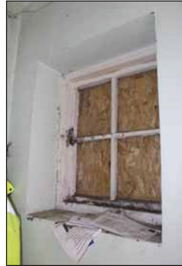
DP 20 Modern casement window in the porch (No. 32: GF01), taken from the north-east
