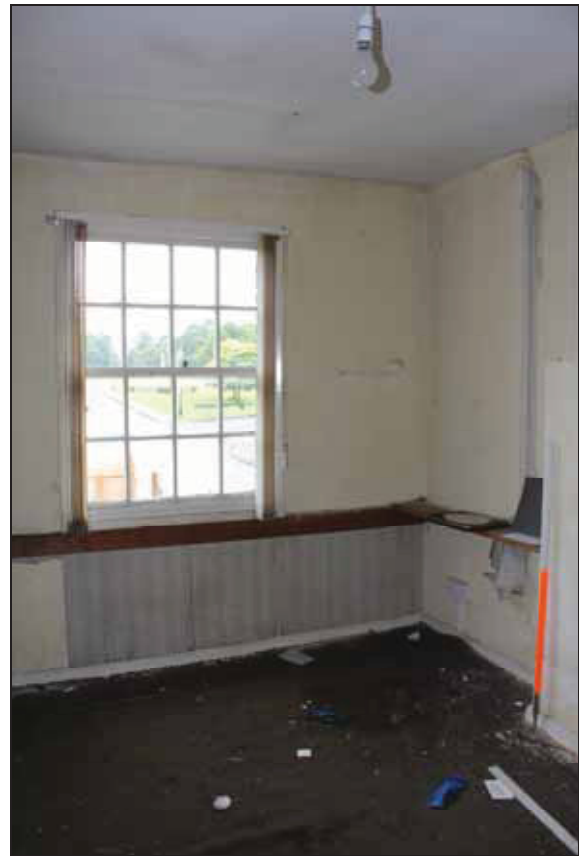
Plate 6 Replacement sash window on the west side of Room FF03 (No. 32), taken from the east (DP 30)
