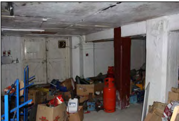
DP 101 East end of Room GF22 (Range 9) showing combination of original and later concrete columns with double doors to the exterior, taken from the west
