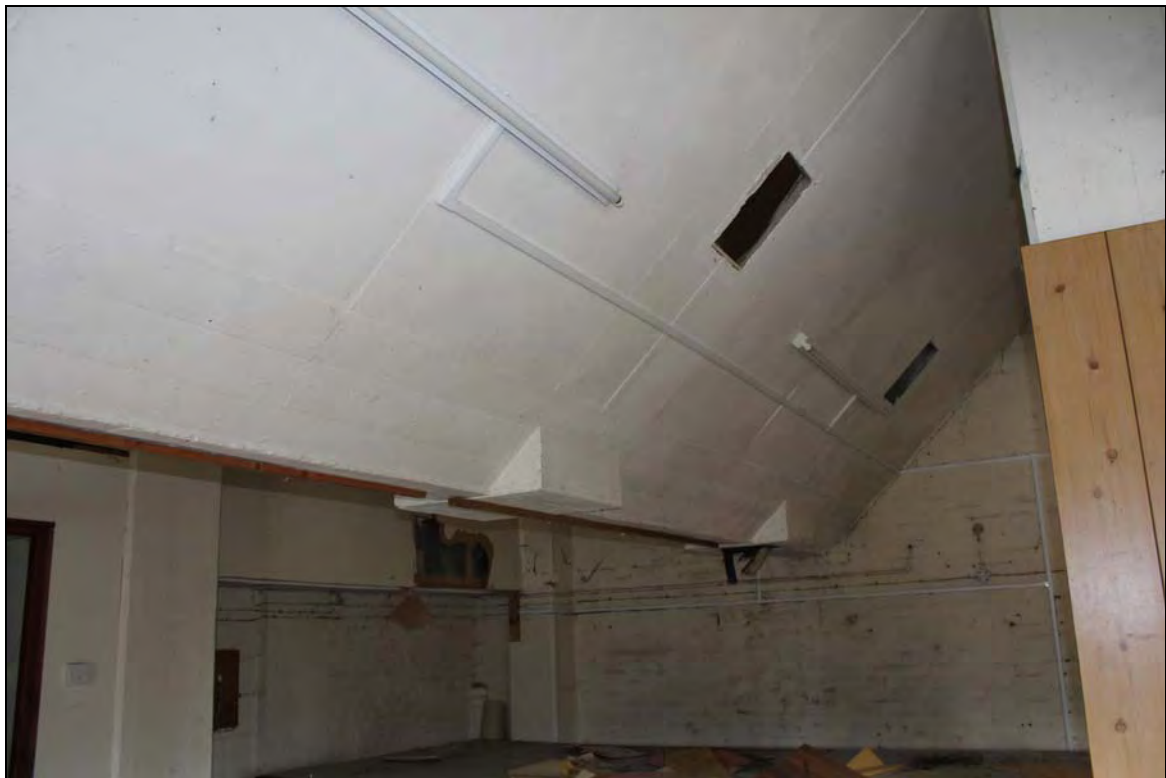
Plate 12 First floor of Range 4 (FF13) showing the underside of the concrete hoppers supported on large concrete columns, taken from the south-east (DP 163)
