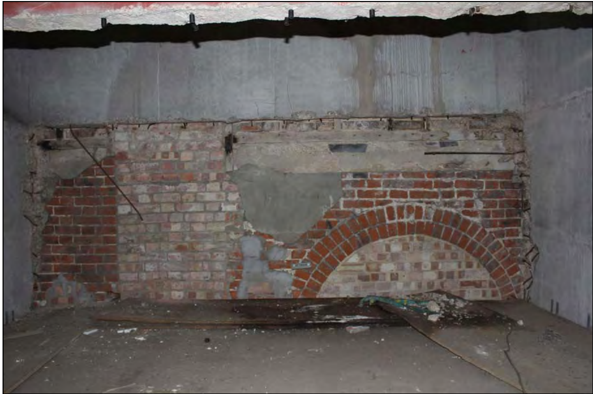
Plate 7 First floor of Range 1 (FF01) showing east wall with earlier brick arch infilled and much rebuilt in Flettons, taken from the west (DP 127)
