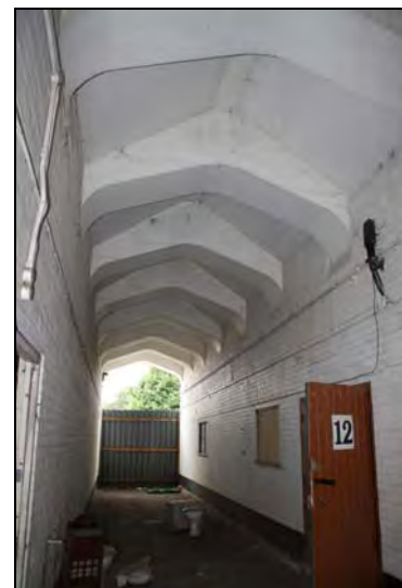
DP 48 View of the tunnel below Range 1 showing shuttered concrete arches, taken from the east
