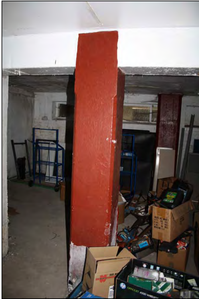
Plate 17 Detail of an original pre-cast concrete column in Range 9 (GF21), taken from the south (DP 97)
