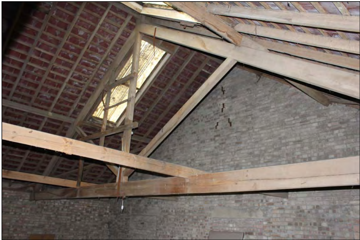
Plate 19 Third floor of Range 9 (TF01) showing king-post roof truss, taken from the north-east (DP 154)
