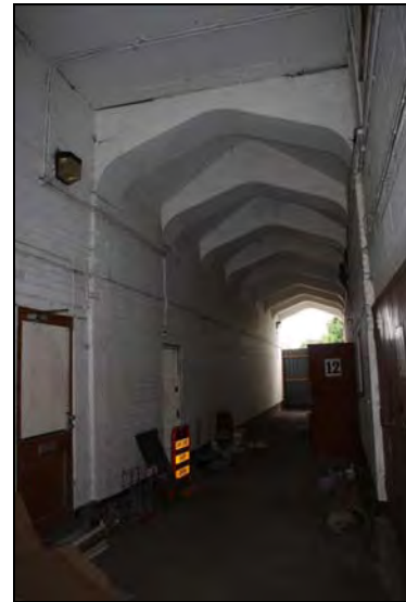
DP 46 View of the tunnel below Range 1 showing shuttered concrete arches, taken from the east
