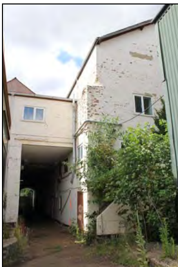
DP 35 View of Range 6 (left) abutting Range 9 (right), taken from the east
