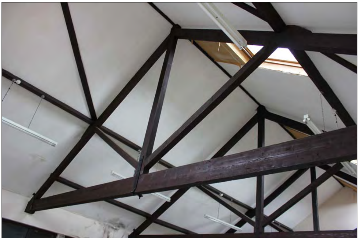
Plate 10 Second floor of Range 3 (SF01) showing the king post roof trusses, taken from the south-west (DP 182)
