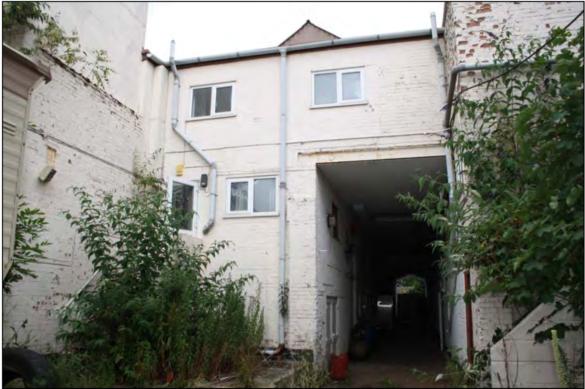
Plate 13 East side of Range 6 showing the tunnel and replacement uPVC windows, taken from the east (DP 31)
