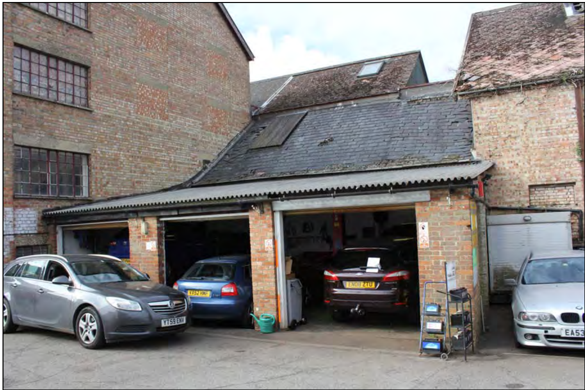
Plate 15 View of Range 8 with the roof pitches of Ranges 7 and 6 above, taken from the north (DP 67)
