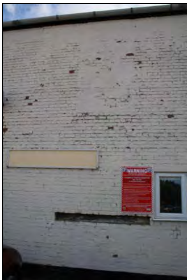
DP 5 Detail of the south elevation (Range 1) showing blocked aperture at low level, taken from the south
