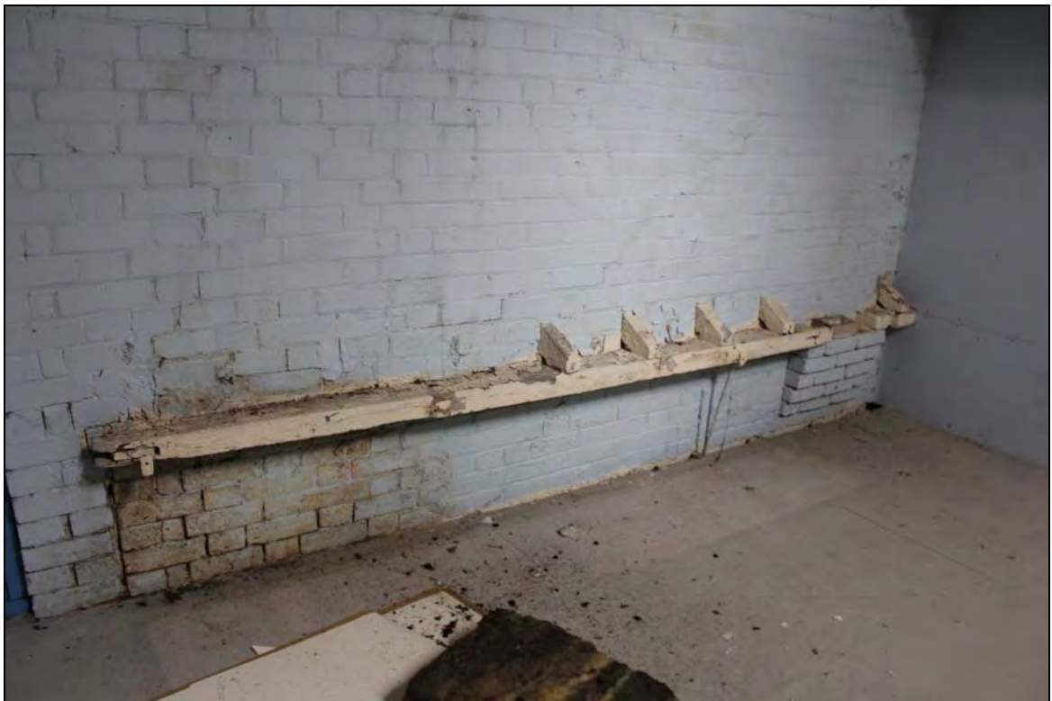
Plate 14 Second floor of Range 6 (SF04) showing the south wall (west end) where the stumps of rafters survive from a lost adjoining roof structure, taken from the north-east (DP 190)
