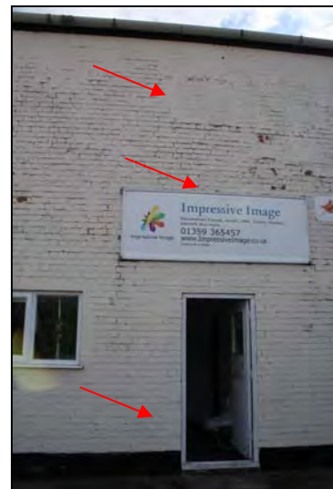
DP 6 Detail of the south elevation (Range 1) showing small blocked apertures marking three original floor levels, taken from the south
