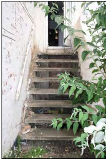
DP 33 Steps on the east side of Range 6 leading to first floor level, taken from the east
