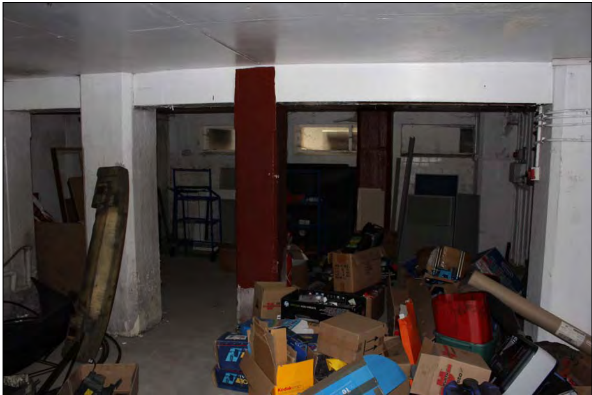
Plate 18 Interior of Range 9 showing pre-cast concrete pillar system supporting the structure above as well as concrete columns of larger profile inserted at the east end (GF21-22), taken from the south (DP 96)
