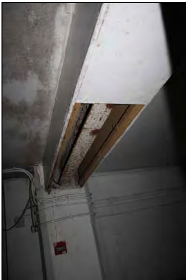
DP 99 Detail of one of a system of ceiling beams supporting the floor above (Range 9: GF21) showing I-profile joist, taken from the south-west
