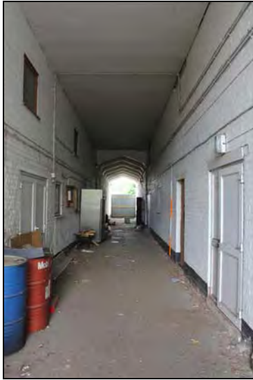
DP 43 View of the tunnel below Ranges 6 and 1 , taken from the east
