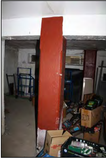
DP 97 Detail of an original pre-cast concrete column in Range 9 (GF21), taken from the south
