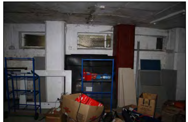
DP 102 North side of Room GF22 (Range 9) showing external brick wall and narrow windows bisected by later concrete columns, taken from the south
