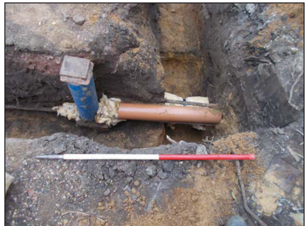
12 Modern services at north eastern corner, looking west.
