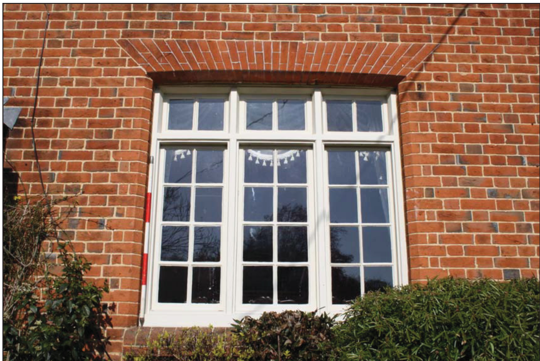
Plate 2 Ground floor window with wide gauged arch, south elevation, taken from the south (DP 4)
