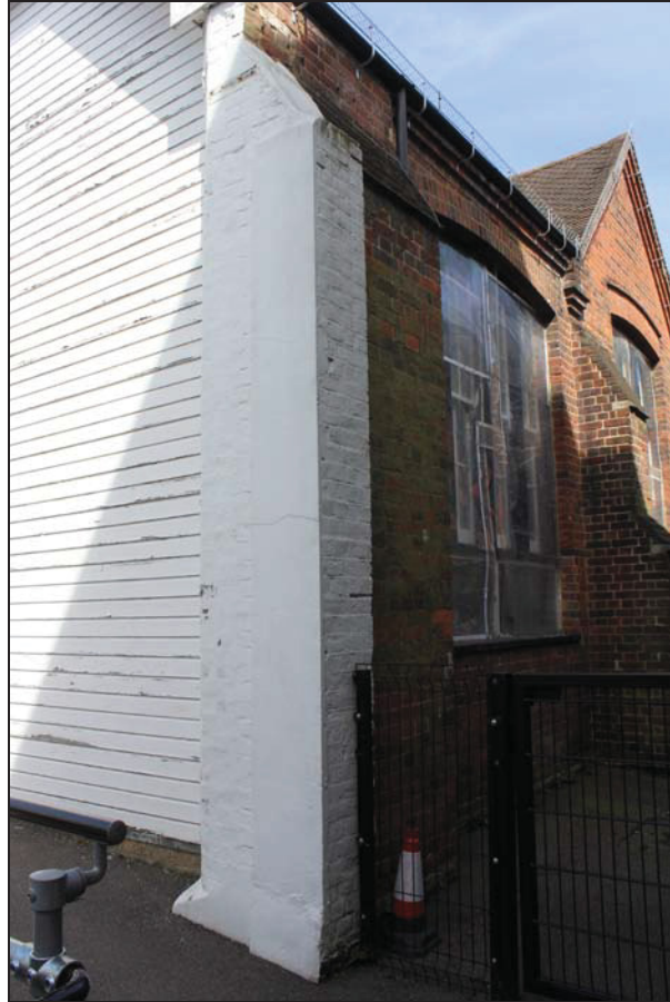
Plate 7 Buttress on the south-east corner of Classroom 3, taken from the south-east (DP 94)
