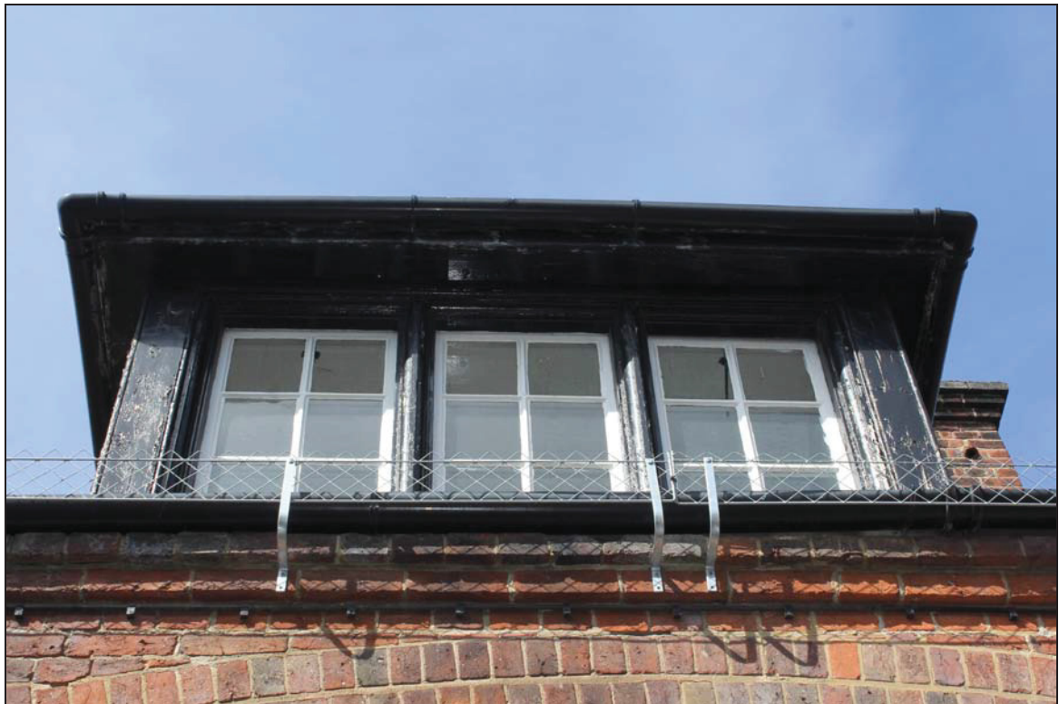
Plate 4 Dormer window in the roof on the east elevation, taken from the east (DP 100)
