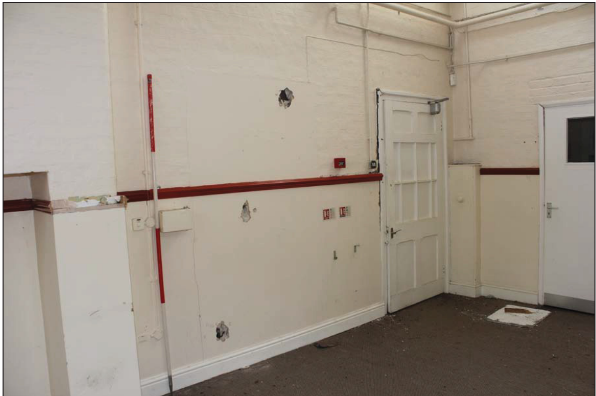
Plate 20 Blocked doorway and external door on the south wall of Classroom 2, taken from the north (DP 59)
