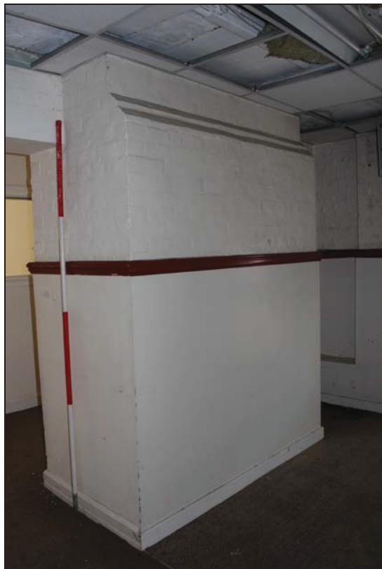
Plate 30 Chimney stack on what would have been the west external wall of Classroom 3, taken from the north-west (DP 83)
