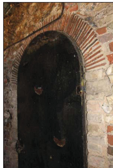
23 North side of the curved wall showing inserted doorway with tiled arch and gault brick jambs, looking south
