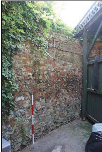
18 North-west side of the curved wall showing mixtures of fabrics including flint and brick of varying dates, looking south
