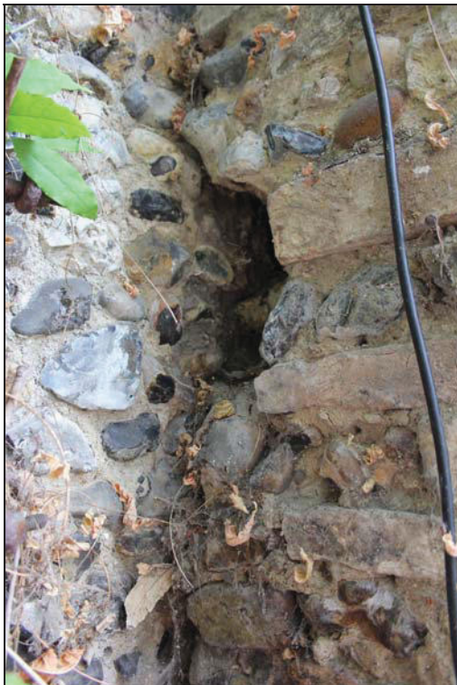
16 Detail of a buttress on the east side of the curved wall showing straight joint, looking north
