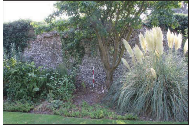
25 Precinct wall (north-west side) to the north-east of the breakfast room showing section of coursed flintwork, looking south-east
