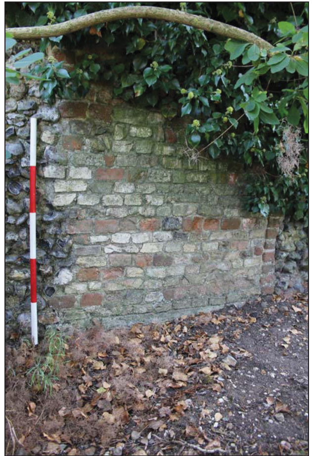
27 Precinct wall to the north-east of the breakfast room showing blocked doorway at the west end that formerly gave access to the glass-house, looking south-east
