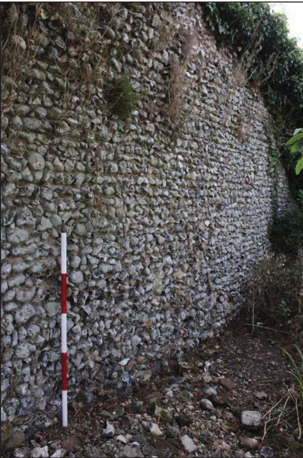
26 Precinct wall (north-west side) to the north-east of the breakfast room showing section of coursed flintwork, looking south-west
