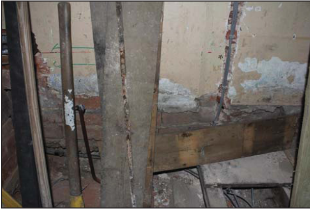
DP 21 Obscured view of the brickwork on the south side of Room GF01 (main range), taken from the north-west
