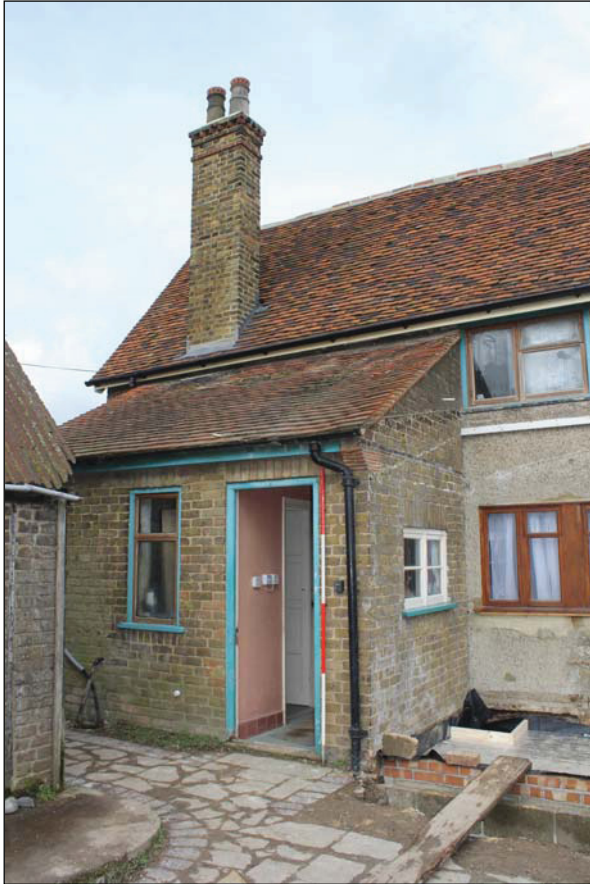
Plate 3 Unit 3 on the south-west side of Unit 2, taken from the south (DP 05)
