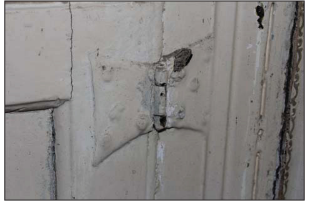
DP 26 Detail of the cupboard showing butterfly hinges on the single-panel door (GF01; main range), taken from the north-west
