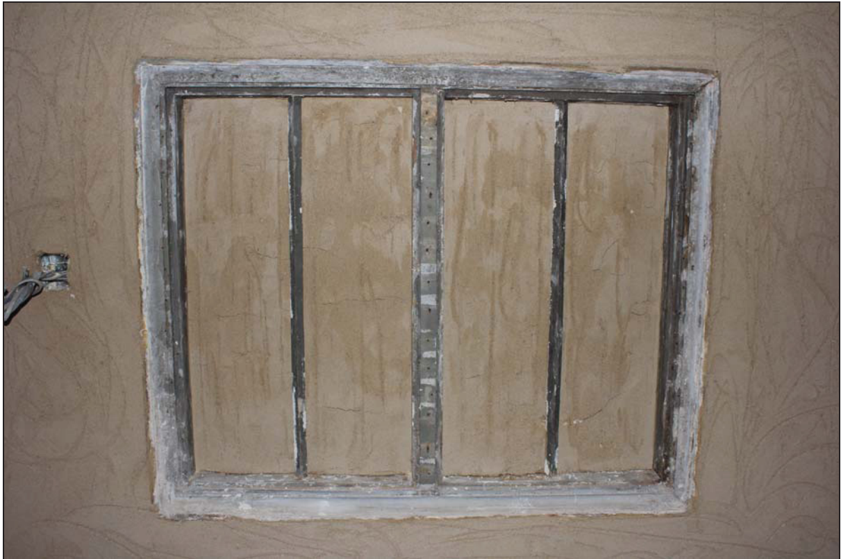
Plate 12 External face of the mullion window on the south-east side of Room FF02 (Unit 2) taken from the north-west (DP 50)
