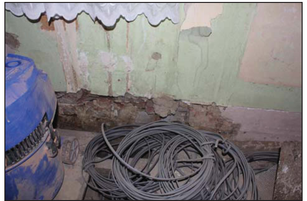
DP 28 Obscured view of the brickwork on the south-west side of Room GF01 (main range), taken from the north-east
