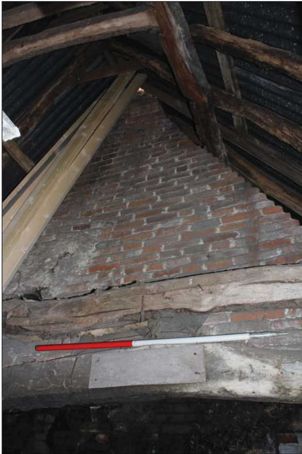
Plate 14 Detail of the chimney stack in the outbuilding showing brickwork of the stack with roof structure over, taken from the south-west (DP 66)
