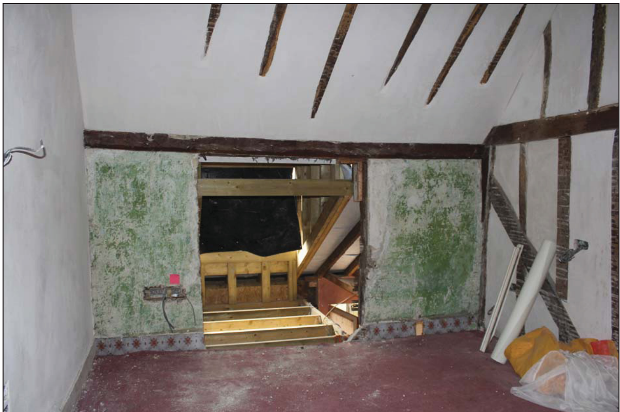
Plate 11 South-west wall of Room FF01 following removal of the window, taken from the north-east (DP 93)
