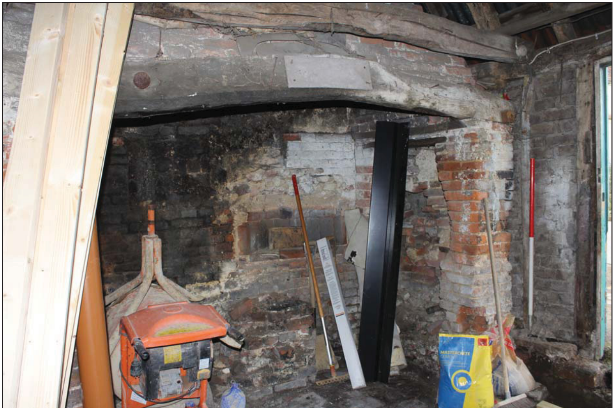
Plate 13 Massive inglenook fireplace at the north-east end of the outbuilding, taken from the west (DP 64)
