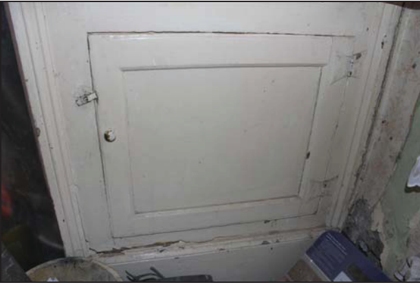
DP 25 Detail of the cupboard showing single-panel door (GF01; main range), taken from the north-west
