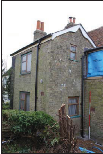
DP 13 Unit 1 on the north-east side of the main range, taken from the north-west
