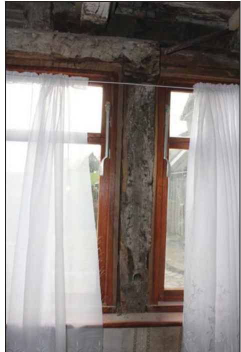
DP 30 South-west side of Room GF01 (main range) showing surviving pegged stud and truncated mid-rail, taken from the north-east
