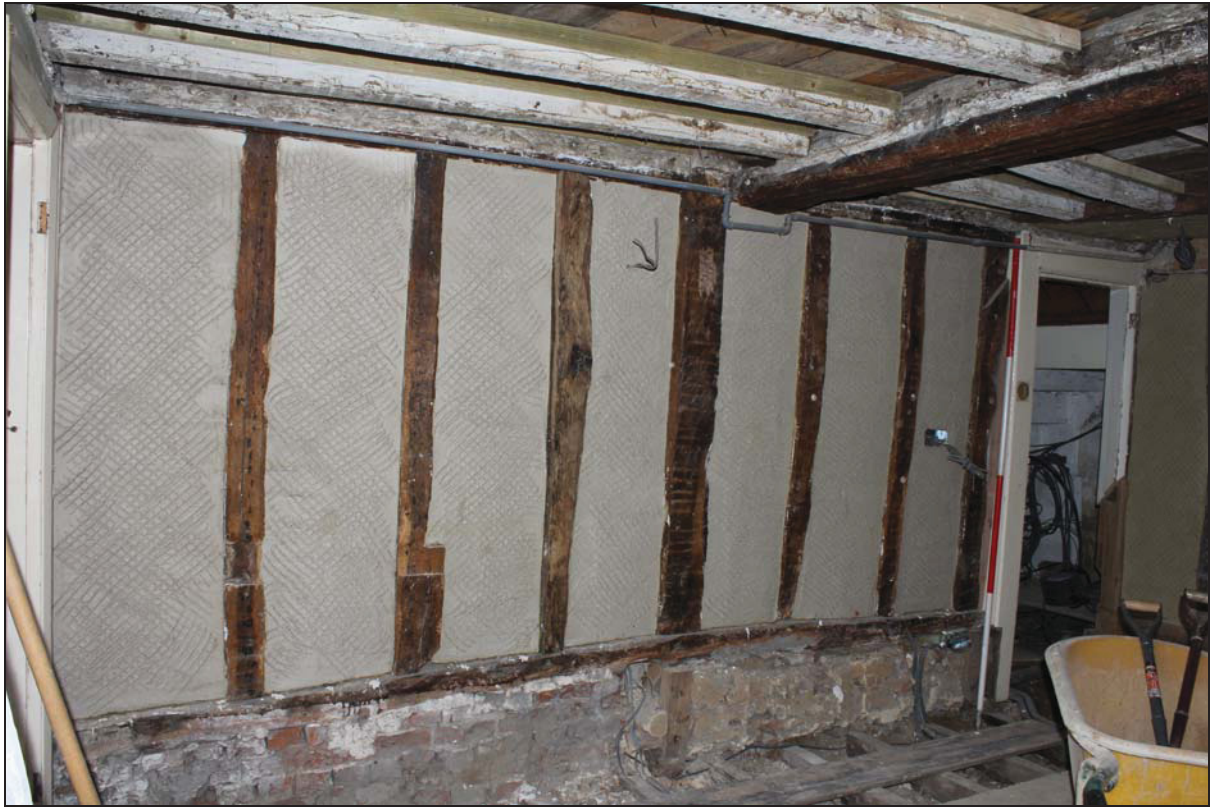
Plate 5 North-west wall of Room GF01 (main range), taken from the south (DP 32)
