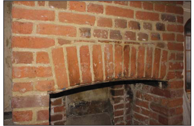
DP 22 Detail of the chimney stack in Room GF01 (main range) showing cambered brick arch and iron soffit strip, taken from the north
