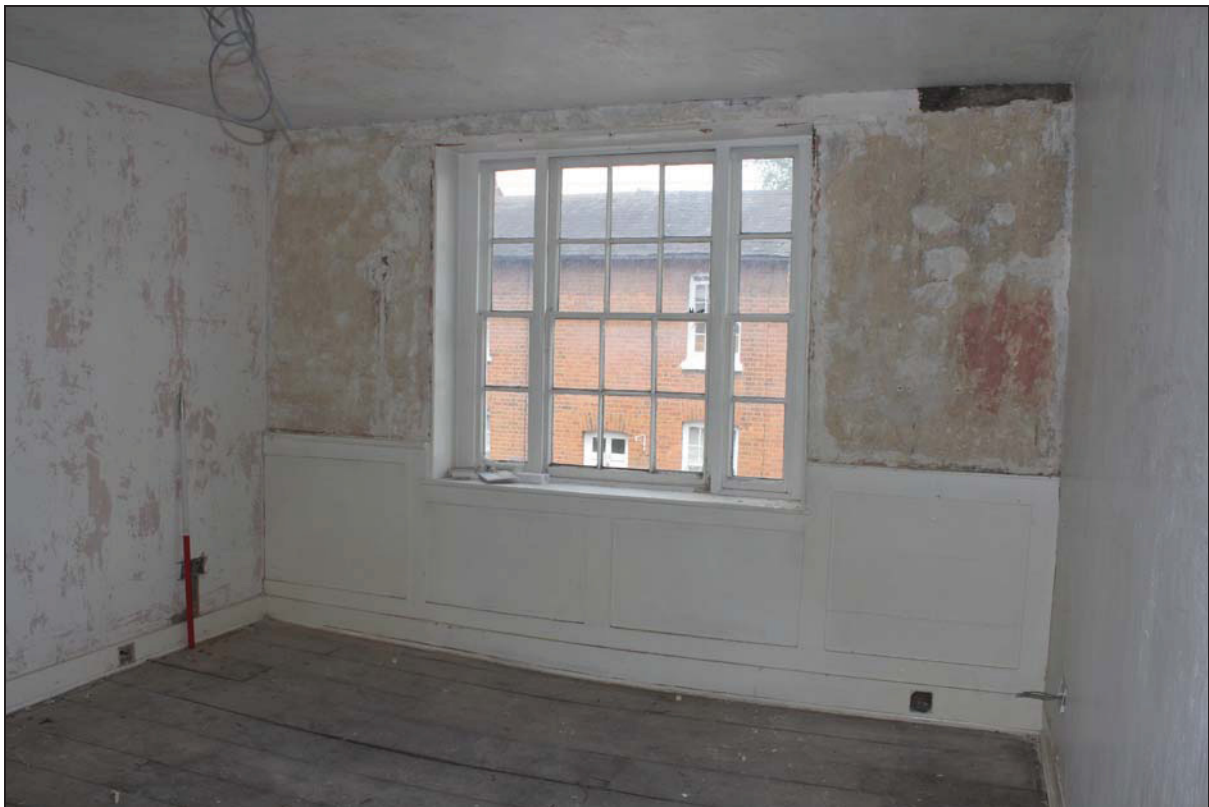
Plate 18 View of Room FF03 during the planned works, taken from the south (DP 95)
