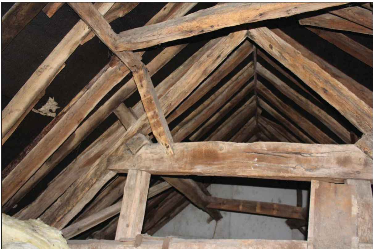
Plate 22 View of the west roof structure over the street front range, taken from the east (DP 14)
