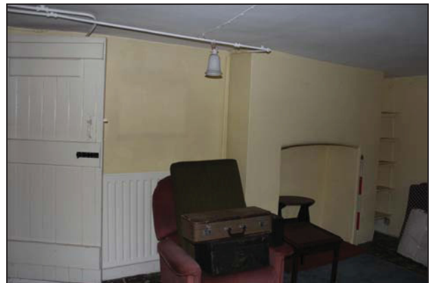
DP 58 North side of Room BF01 showing chimney breast with fireplace aperture, taken from the south-west
