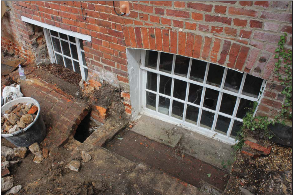
Plate 7 View of the south side of the building (east end) showing original brick retaining structure keeping the fabric of the terrace away from the house, taken from the south (DP 119)
