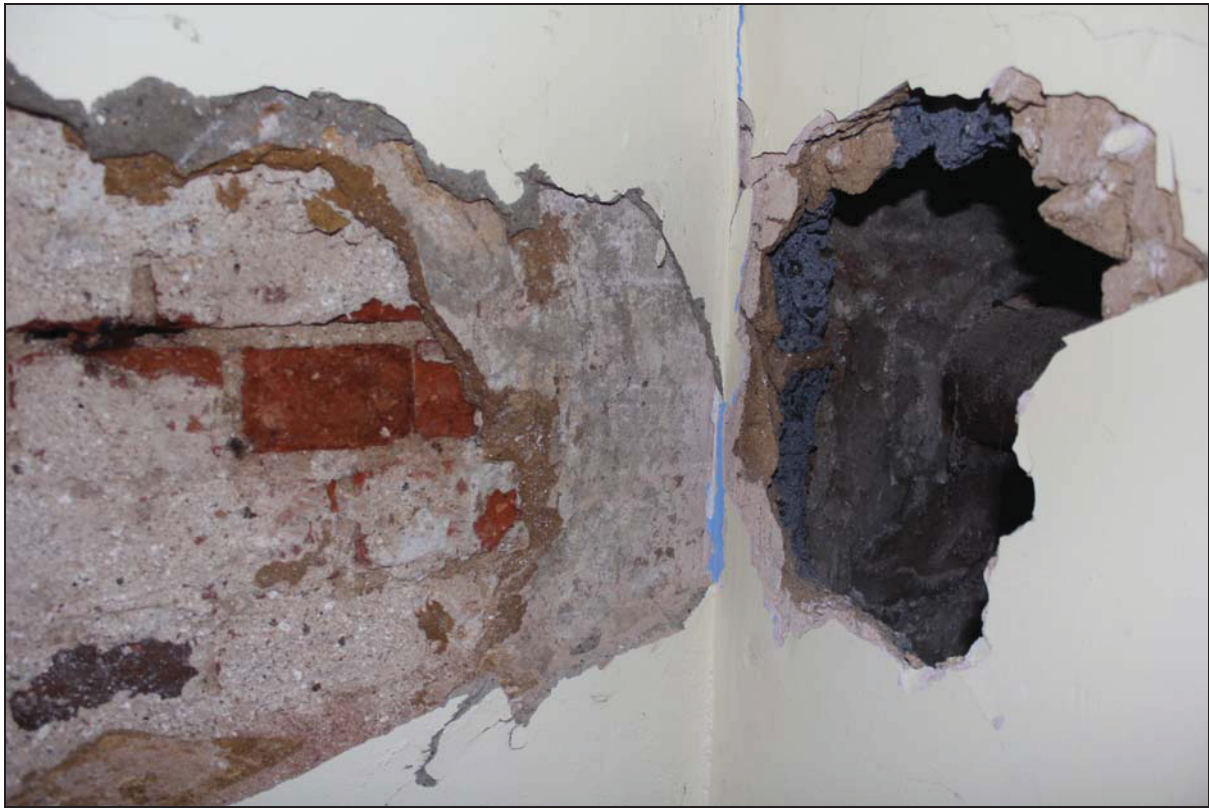
Plate 21 Detail showing the south-west corner of Room BF01 showing brickwork on the left and block work of the attached pier to the right, taken from the north (DP 72)
