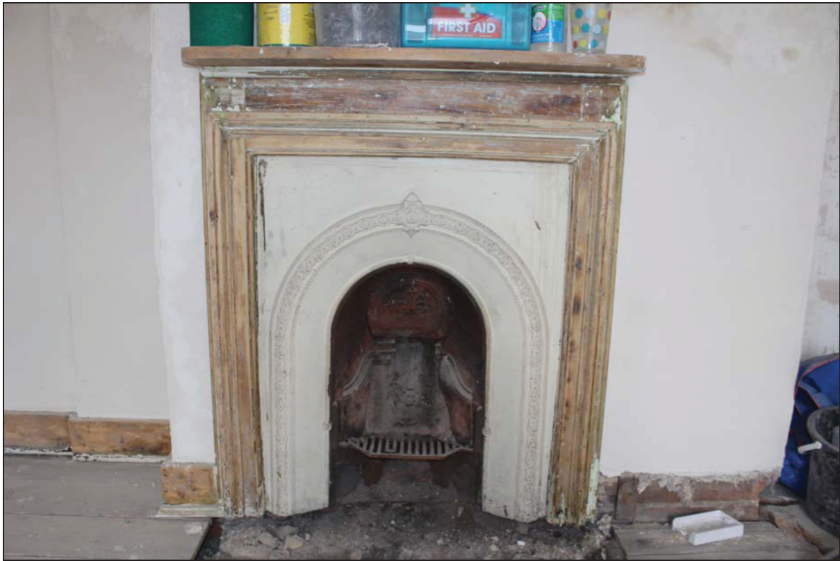
Plate 17 Fireplace on the south side of Room FF03, taken from the north (DP 110)
