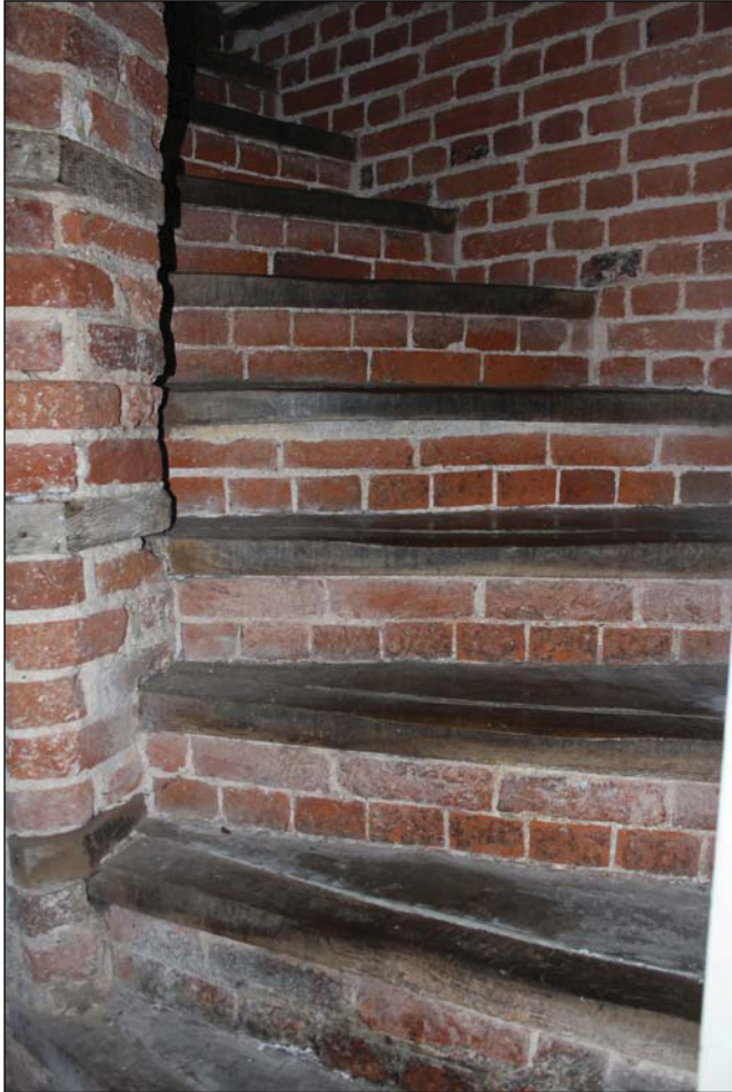
Plate 19 Detail of the timber and brick staircase at basement level, taken from the south (DP 55)
