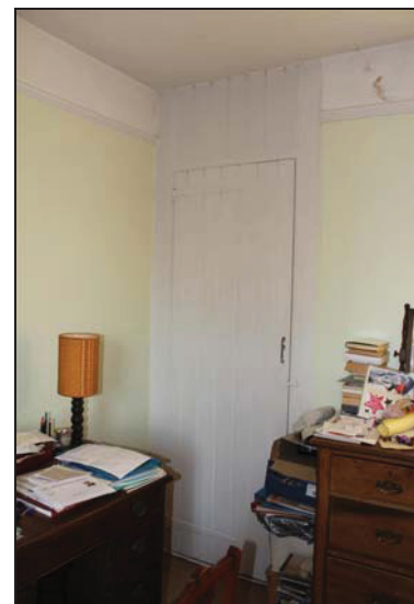
DP 30 Integral cupboard in the north-west corner of Room FF06, taken from the south-east
