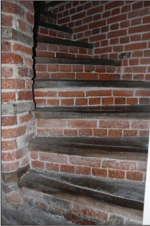
DP 55 Detail of the timber and brick staircase at basement level, taken from the south
