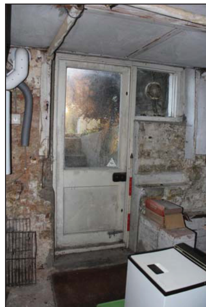
DP 66 Doorway on the south side of Room BF02, taken from the north
