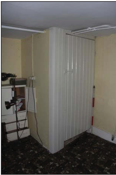
DP 63 Door enclosing the lobby area at basement level, taken from the south-east
