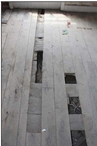
DP 89 View of Room FF04 showing modern boarding over the original floorboards, taken from the north
