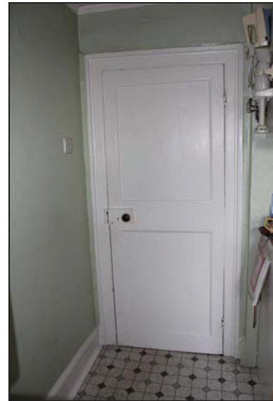
DP 52 Two-panelled door on the north side of Room GF06, taken from the south
