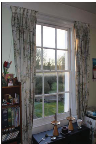
DP 29 Window on the south side of Room FF06, taken from the north
