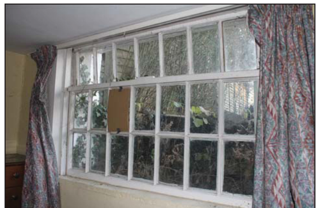
DP 60 East window on the south side of Room BF01, taken from the north
