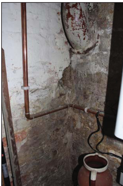
DP 65 Internal walls between Room BF01 and BF02 showing junction with the south wall, taken from the north-west
