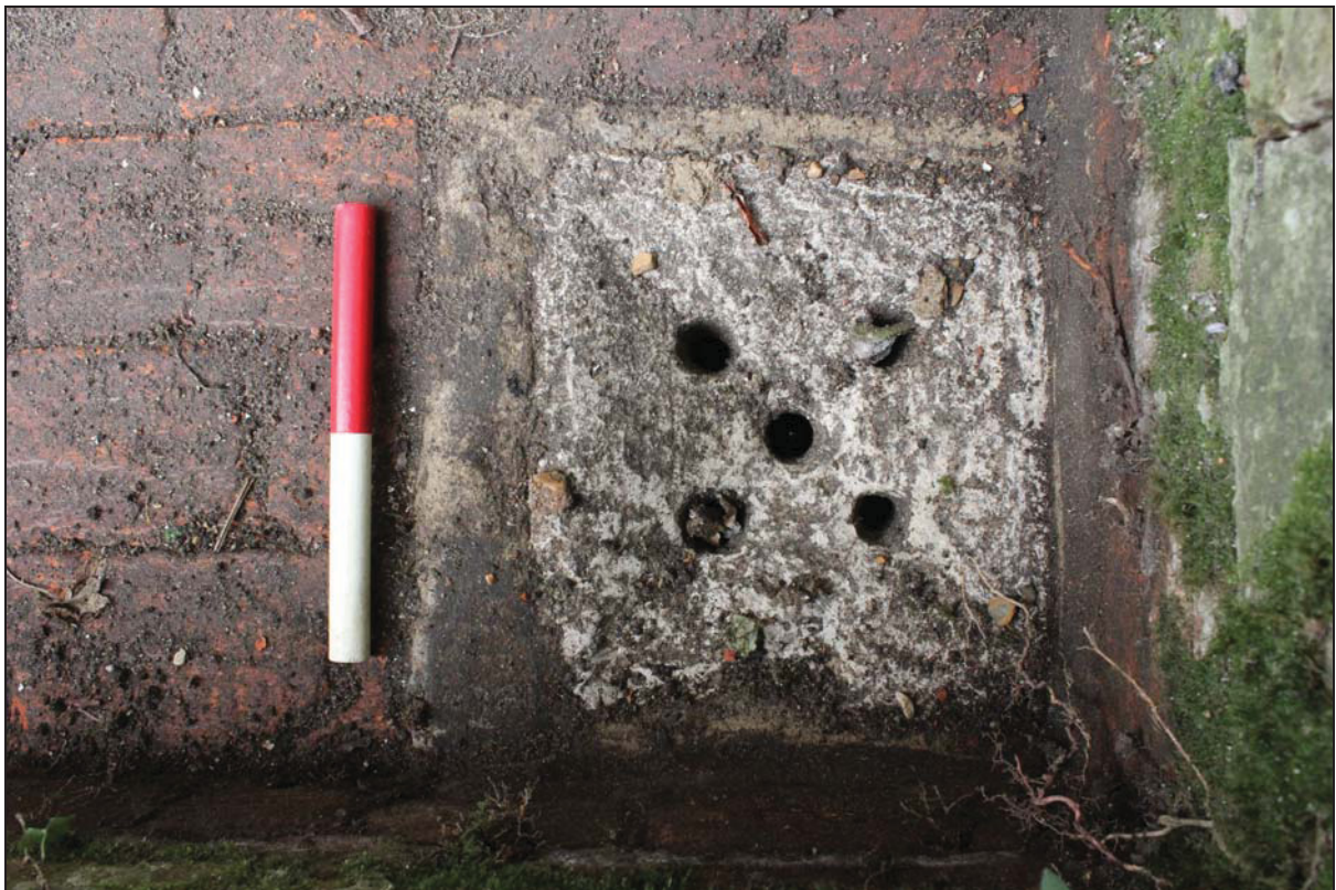
Plate 8 Detail of the stone drain within the brick retaining structure on the south side of the building (east end), taken from the south (DP 126)
