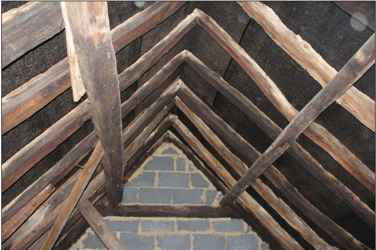
Plate 23 View of the east roof structure over the street front range, taken from the west (DP 15)
