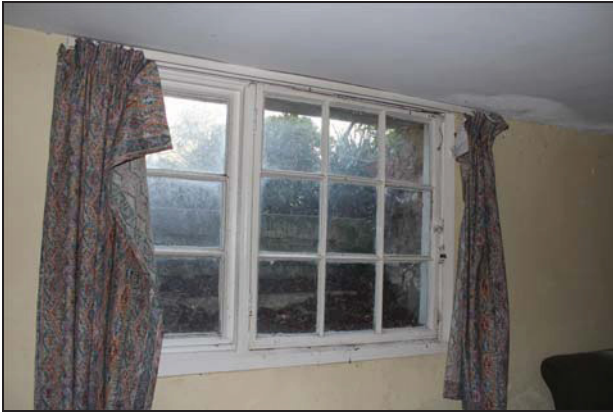
DP 61 West window on the south side of Room BF01, taken from the north
