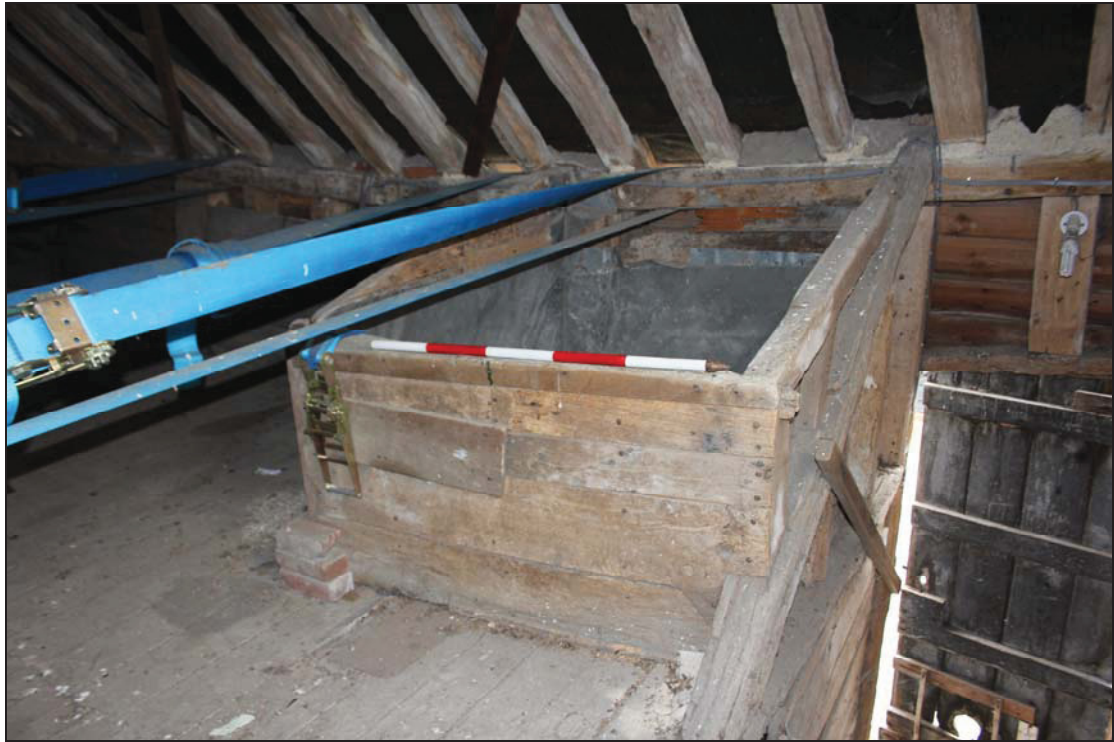
Plate 21 Granary bin on the first floor of Building 2, taken from the west (DP 48)
