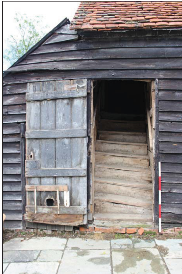
Plate 20 Staircase giving access to the first floor of Building 2, taken from the south-east (DP 65)
