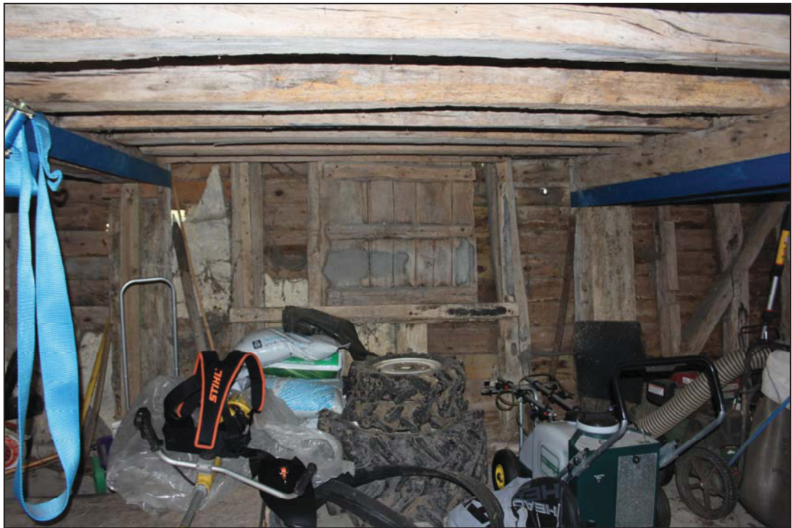
Plate 16 North wall of the central bay in Building 2, taken from the south-east (DP 60)
