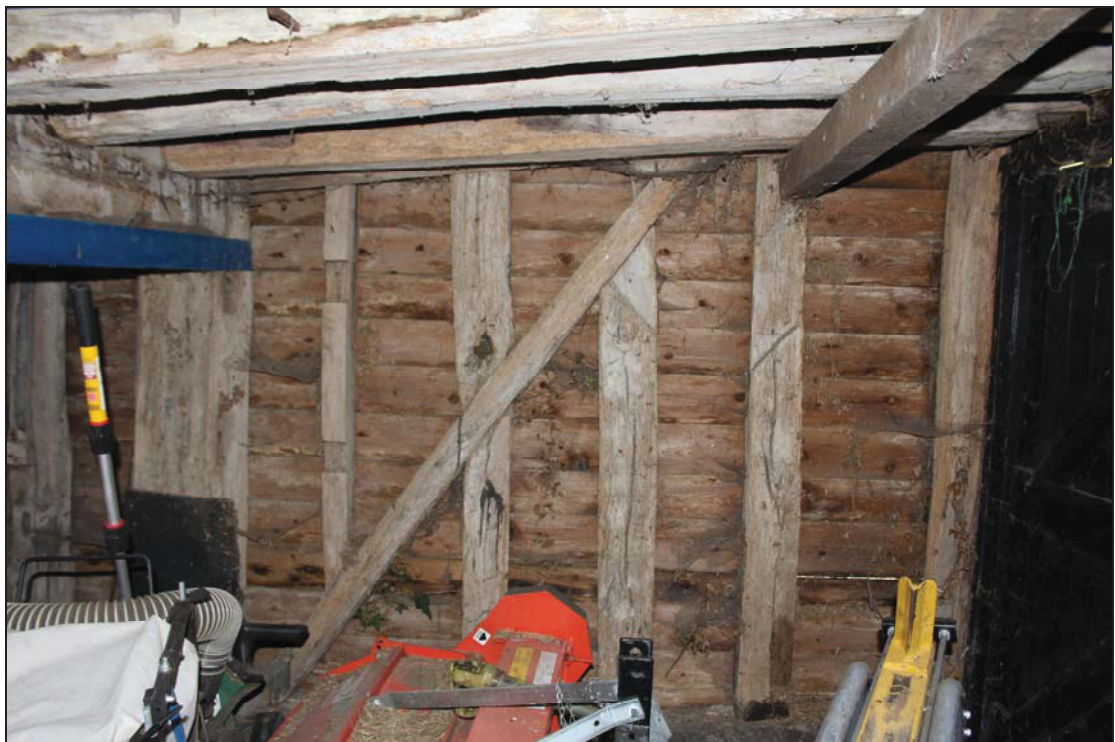
Plate 14 North wall of the east bay of Building 2, taken from the south-east (DP 45)
