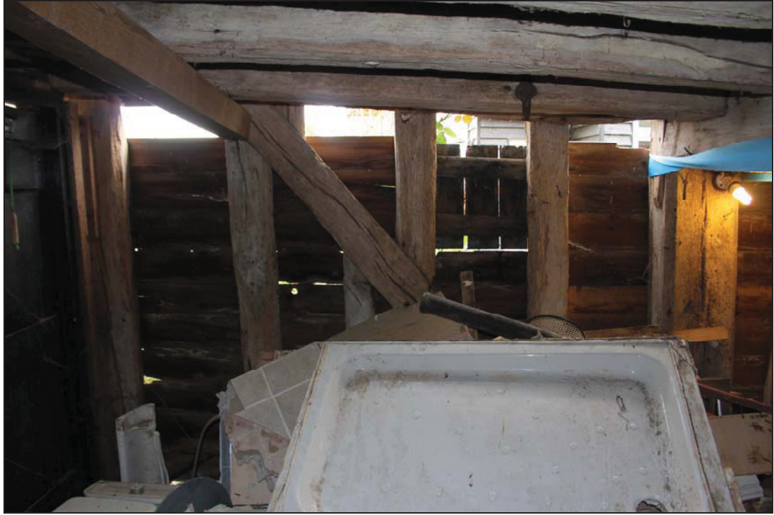
Plate 15 South wall of the east bay of Building 2, taken from the north-west (DP 44)
