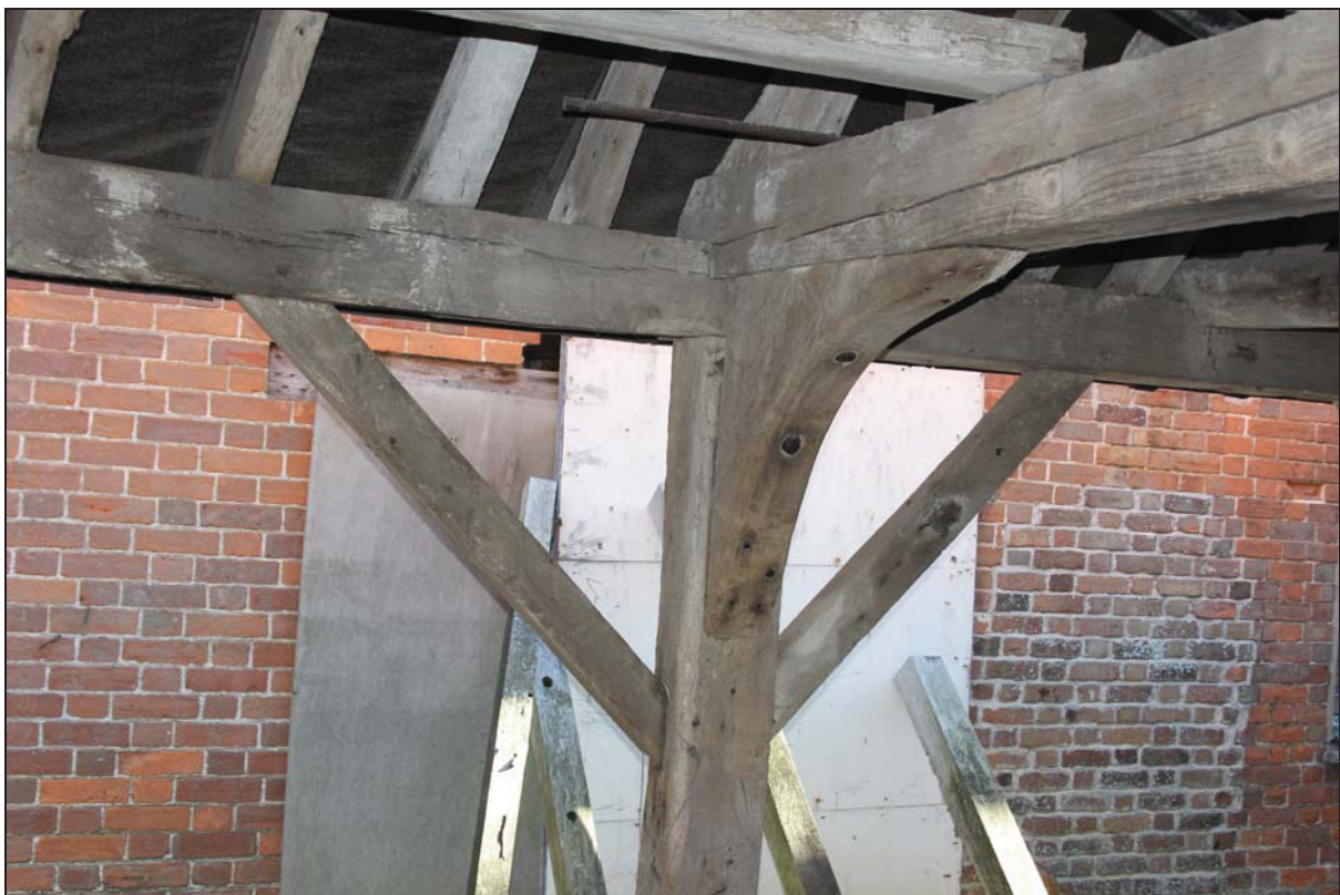
Plate 12 Triangulation of the principal post and tie-beam with an elbow bracket in Building 2, taken from the north-west (DP 75)
