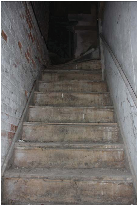
Plate 8 Staircase giving access to the first floor of Building 1, taken from the north (DP 56)
