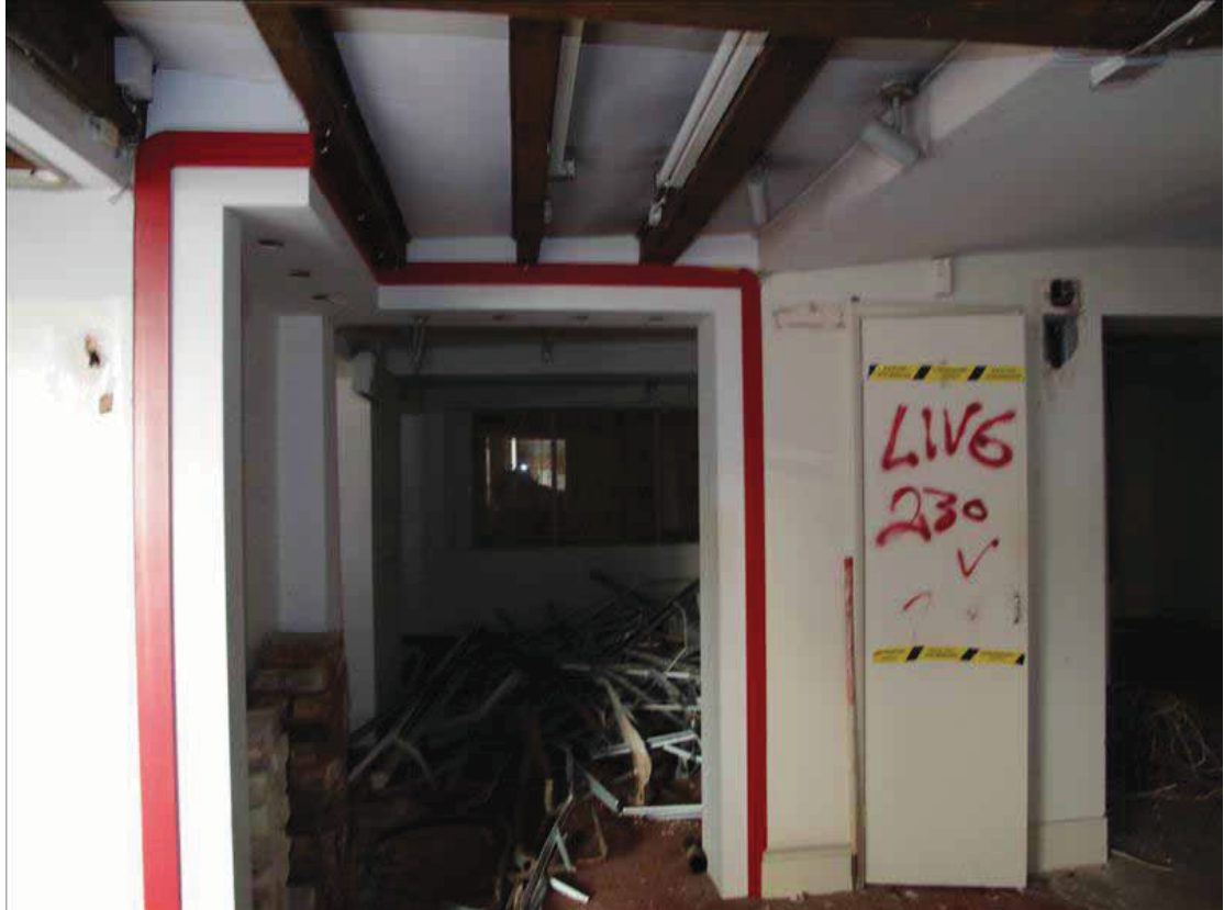
Plate 3 Interior ground floor space of No. 15, with modern room divisions and preserving roof timbers. Taken from the west (DP 7)
