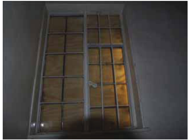
26 Window preserved above winder stair towards 2 nd floor of No. 17. Taken from the west.
