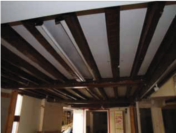
11 Roof timbers above ground floor space of No. 15. Taken from the west.
