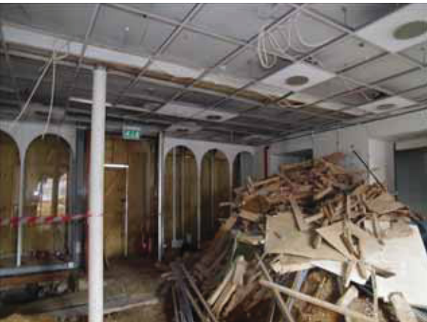
5 Main interior ground floor space of No. 17 (GF01). Taken from the north-west.
