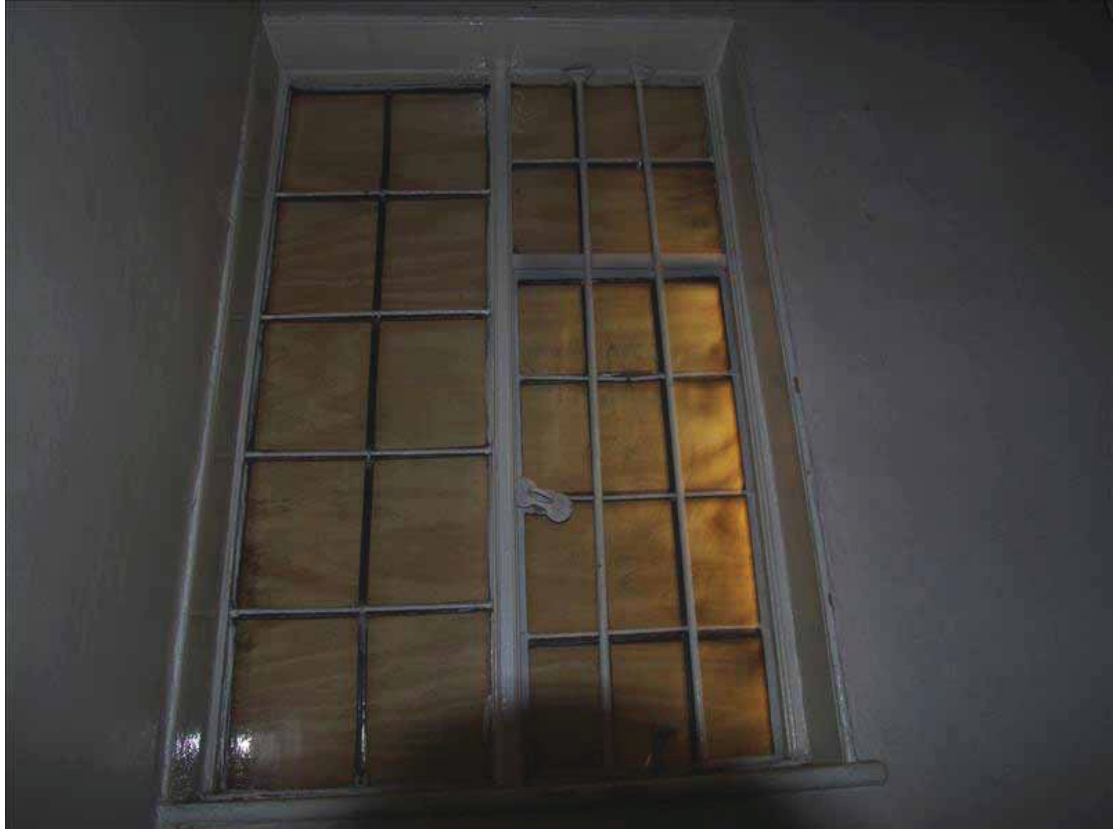
Plate 9 Early window preserved above stairway to second floor of No. 17. Retaining original casements and late 17 th century moulding style, with iron catch and scrolled pull (DP 26)
