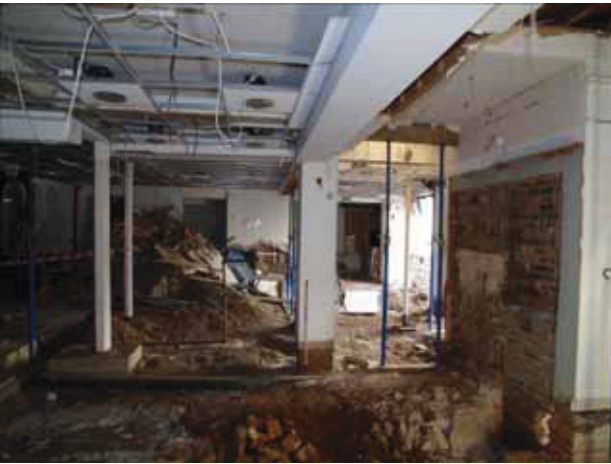
3 Main interior ground floor space of No. 17 (GF01). Taken from the north.
