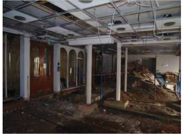
2 Main interior ground floor space of No. 17 (GF01). Taken from the north-west.
