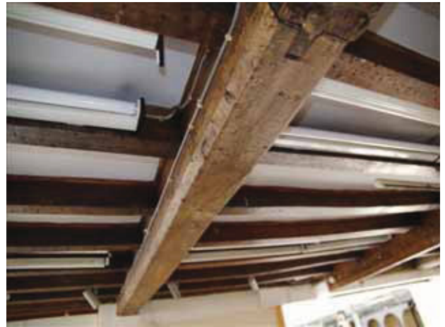
12 Roof timbers above ground floor space of No. 15. Taken from the south-west.
