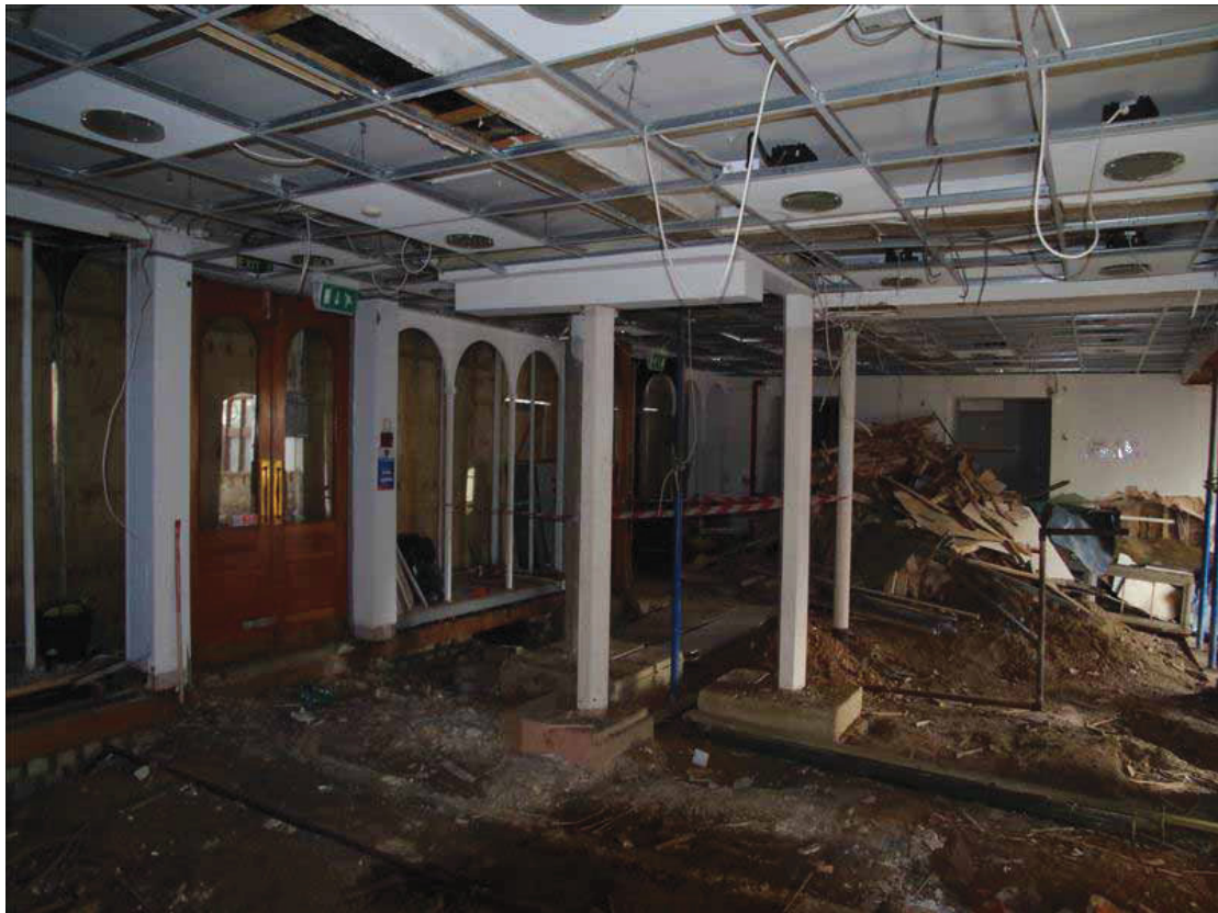
Plate 2 Main interior ground floor space of No. 17, showing cast iron shop front, and columns replacing the original chimney stack. Taken from the north-west (DP 2)
