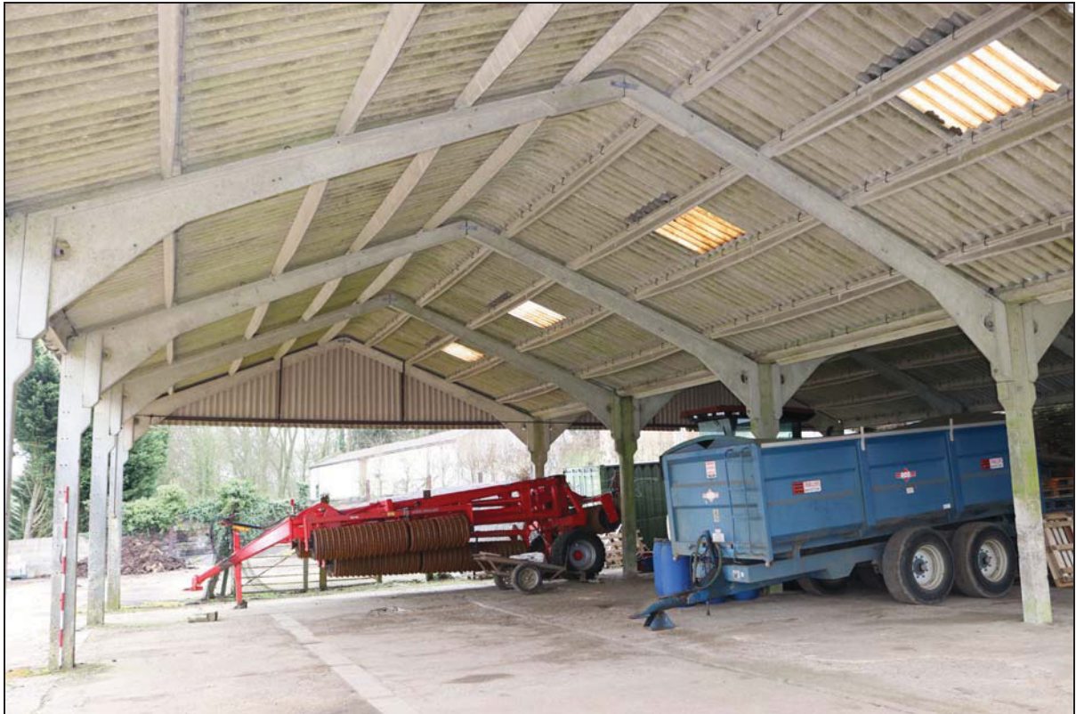
Plate 15 Interior of Building 3 showing concrete Atcost construction, taken from the south-west (DP 21)
