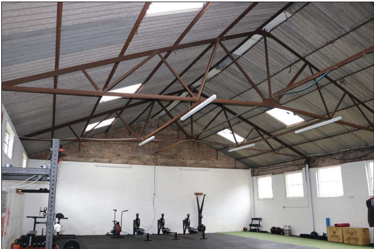
Plate 14 Interior of Building 2 showing iron trusses and Fletton brickwork to the outer walls, taken from the south-east (DP 73)
