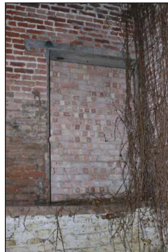
DP 42 North-east wall of the southern unit showing high-set aperture infilled with 20 th century Fletton brickwork, taken from the south-west
