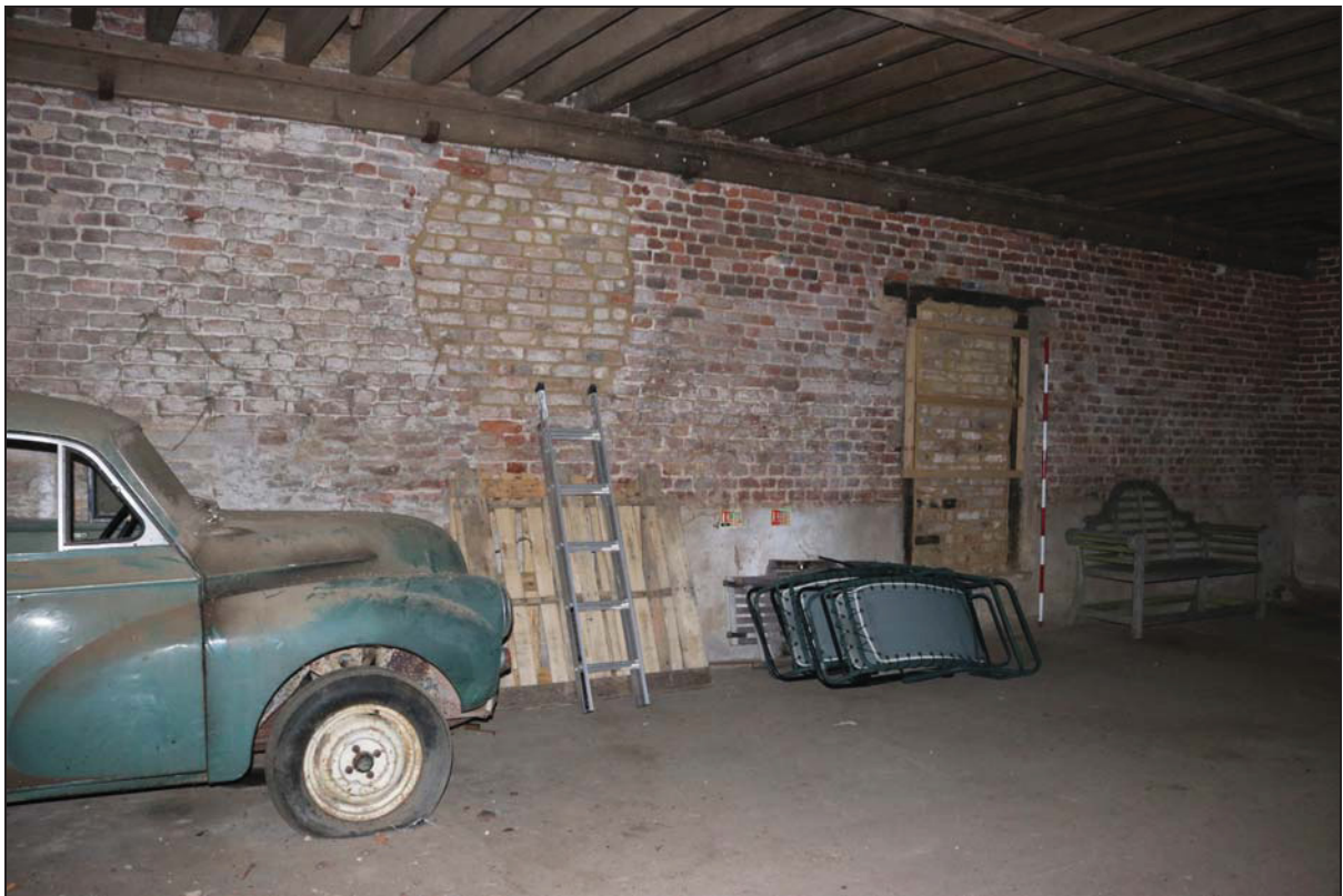
Plate 8 South-east wall of the southern unit (Building 1: barn) at the southern end with inserted circular aperture and doorway, both now blocked, taken from the north-west (DP 54)
