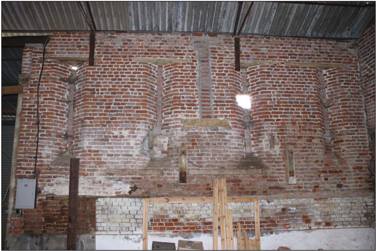
Plate 7 North-west wall of the southern unit (Building 1: barn) showing infilled wind-eyes and infilled recess in the position of a former truss, taken from the south-east (DP 40)
