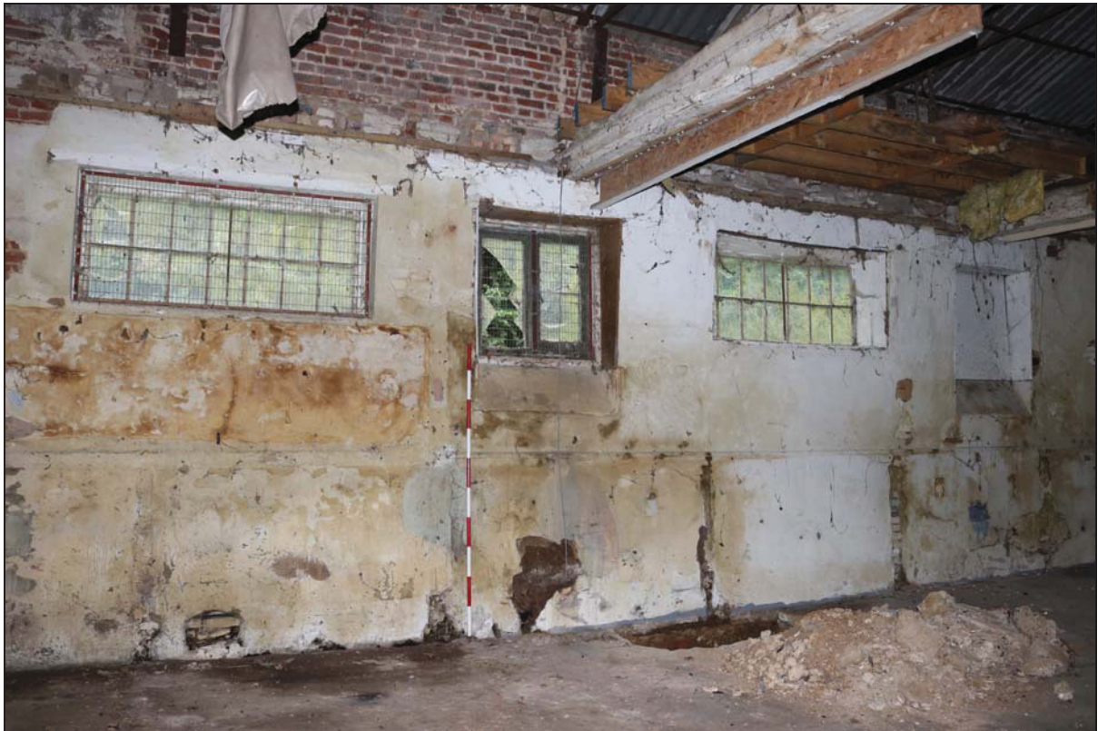
Plate 12 South-east wall of the northern unit (Building 1: barn), taken from the north (DP 26)
