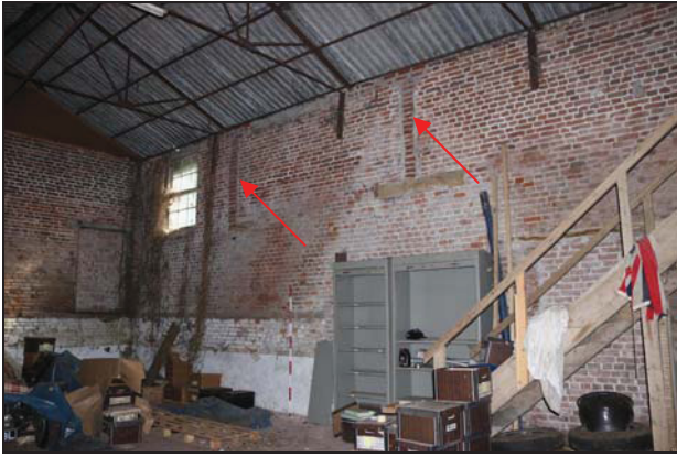
DP 37 South-east wall of the southern unit (Building 1: barn) showing infilled recesses in the brickwork for former wall posts (indicated), taken from the west
