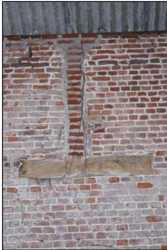
DP 39 Detail of the south-east wall of the northern unit (Building 1: barn) showing infilled recess for wall-post over a timber pad, taken from the north-west
