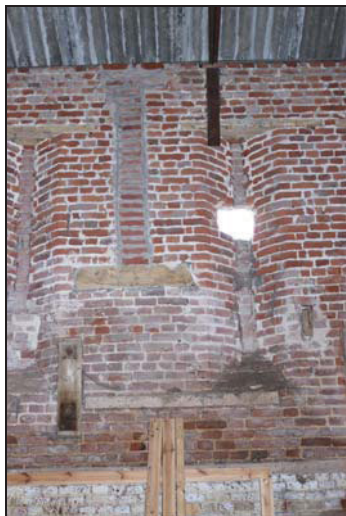
DP 41 Detail of the north-west wall of the southern unit (Building 1: barn) showing infilled wind-eyes and infilled recess in the position of a former truss, taken from the south-east
