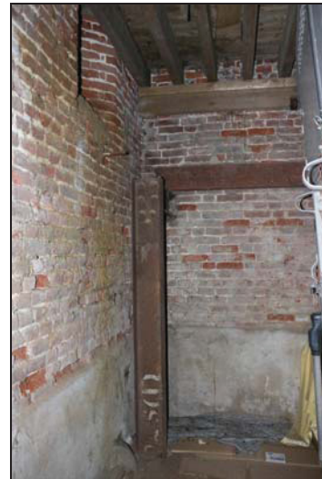
DP 58 South-west end of the southern unit (Building 1: barn) showing later steel elements presumably to hold driveshaft machinery, taken from the south-east
