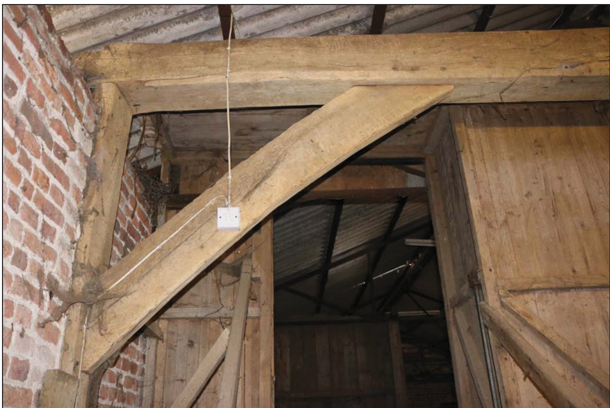
Plate 10 Detail of the surviving truss (Building 1: barn) showing pegged wall-post, tie-beam and brace, taken from the north-east (DP 50)
