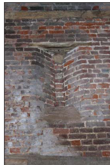
DP 36 Detail of the south-west wall of the porch (Building 1: barn) showing infilled wind-eye, taken from the north-east
