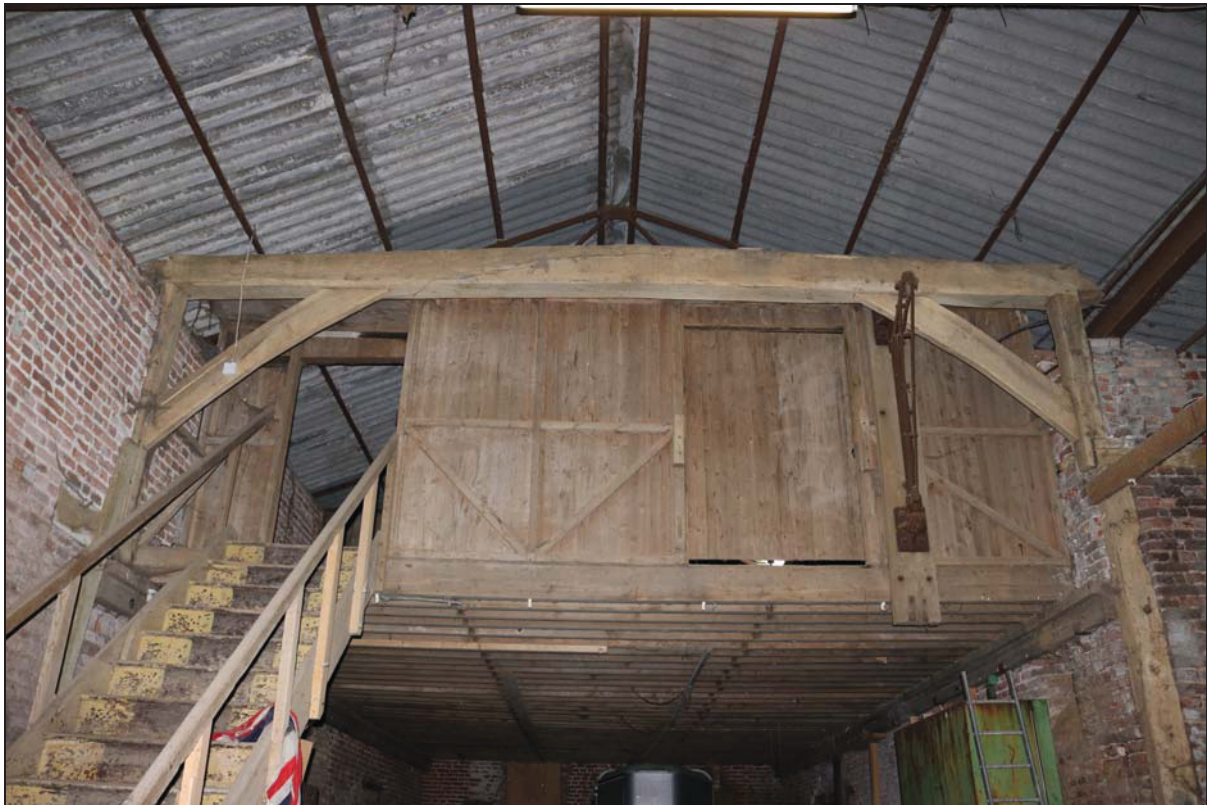
Plate 9 Detail of the surviving original truss (Building 1: barn) with inserted upper floor beyond, taken from the north-east (DP 45)
