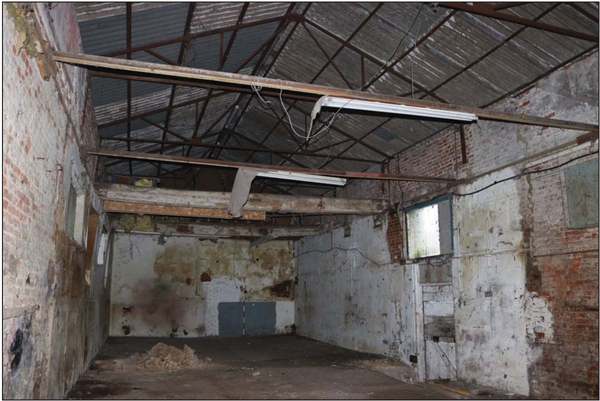
Plate 11 Interior of the northern unit (Building 1: barn), taken from the north-east (DP 24)
