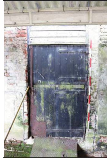
DP 32 North-west elevation of the barn (Building 1) showing entrance to the northern unit, taken from the north-west
