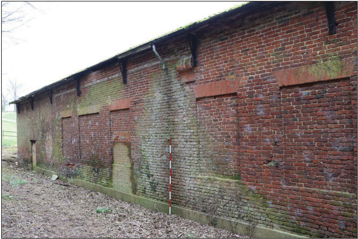
Plate 5 South-east elevation (Building 1: barn) showing blind panels with blocked apertures, taken from the north-east (DP 7)
