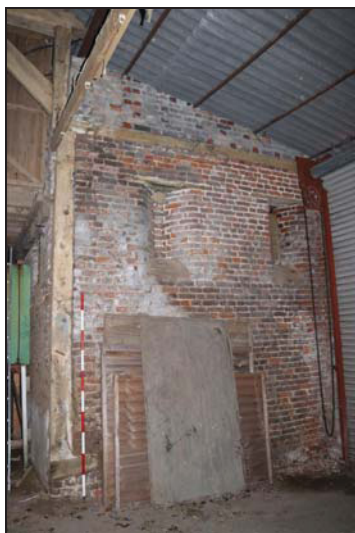
DP 35 South-west wall of the porch (Building 1: barn) showing infilled wind-eyes, taken from the south-east
