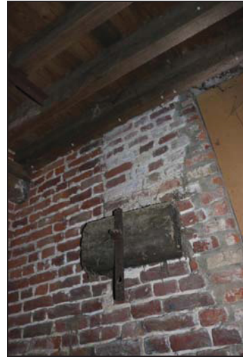
DP 56 South-west wall of the southern unit (Building 1: barn) showing infilled wind-eye with timber block and iron tie, taken from the north-east
