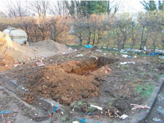
DP 1. Test pit within cycle store to the north-east of the building. Looking north-north-east.
