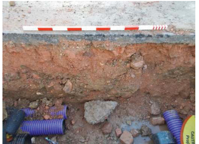
DP 4. Drainage trench to the north-west of the building. Sample section 2. Looking east-north-east.
