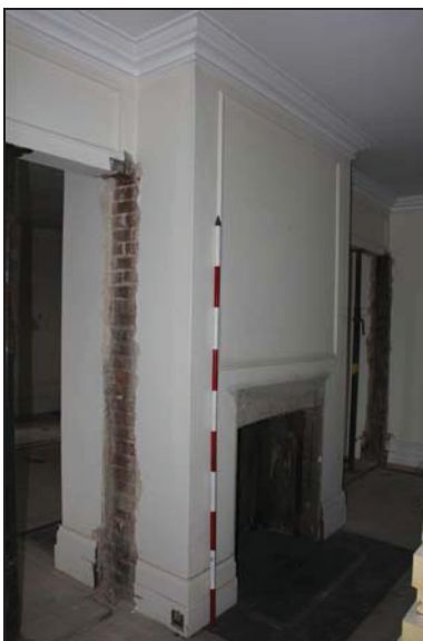
DP 59 Chimneybreast on west side of Room GF04, taken from the south-east
