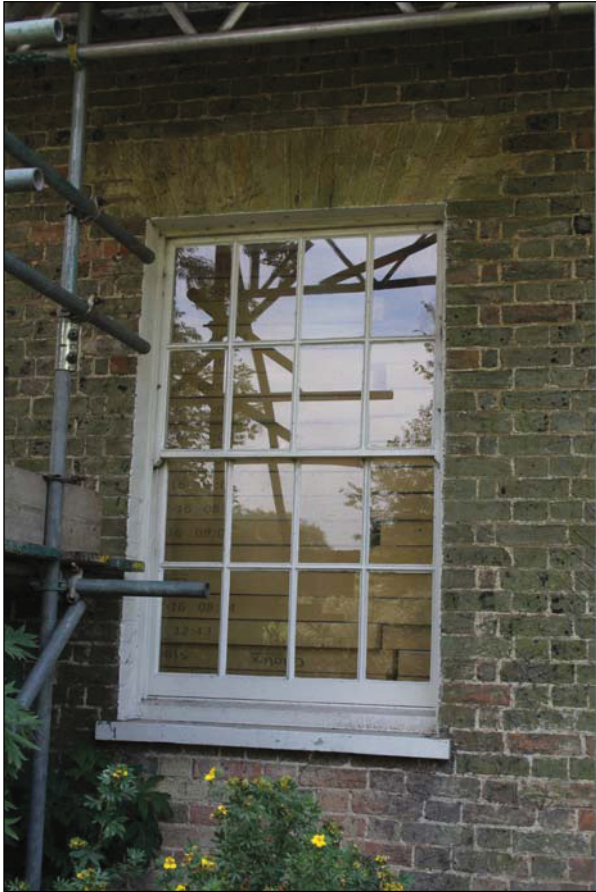
Plate 3 Recessed sash window on the east elevation with a flat gauged brick arch, taken from the east (DP36)
