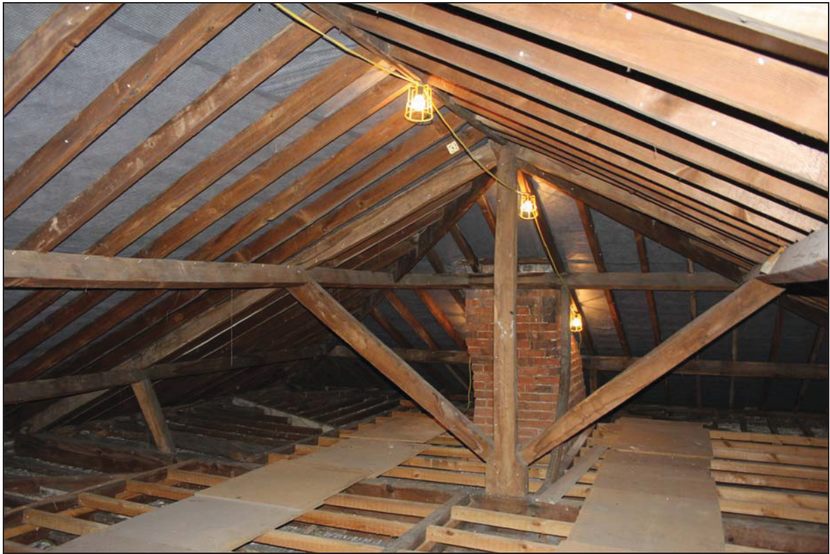
Plate 17 King-post roof structure over the house (south-truss), taken from the north (DP17)
