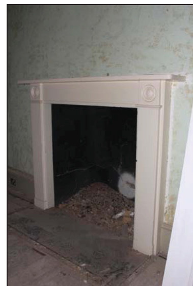
DP 66 Simple Regency fire surround on the east side of Room GF02, taken from the south-west
