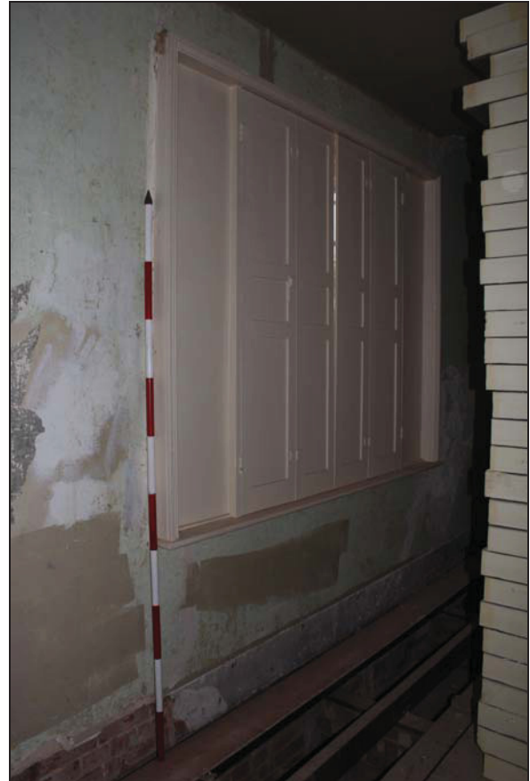
Plate 8 Sash window with shutters on the west side of Room GF02, taken from the south-east (DP65)
