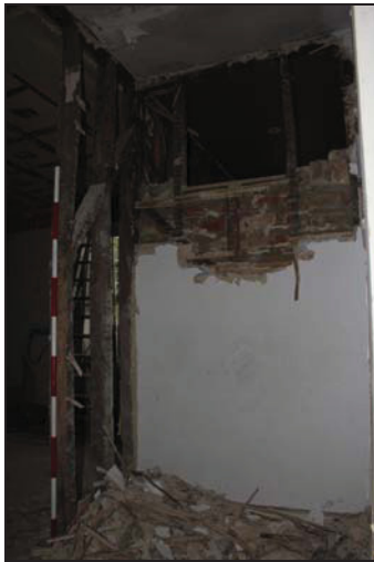
DP 3 Primary-braced studwork partition in Room GF05 during removal of lath and plasterwork, taken from the west
