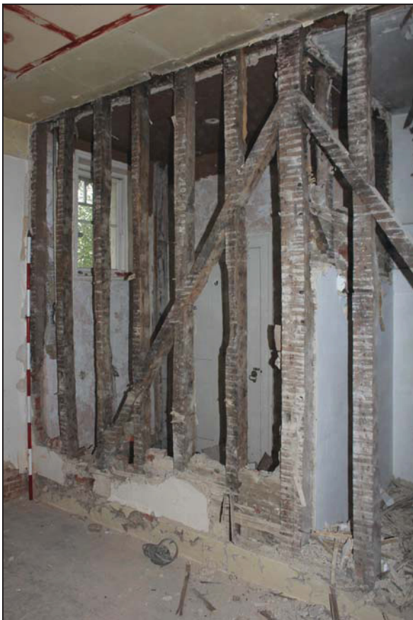
Plate 11 Primary-braced studwork partition in Room GF05 after removal of lath and plasterwork, taken from the north-west (DP01)
