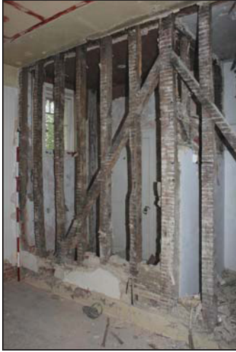
DP 1 Primary-braced studwork partition in Room GF05 after removal of lath and plasterwork, taken from the north-west
