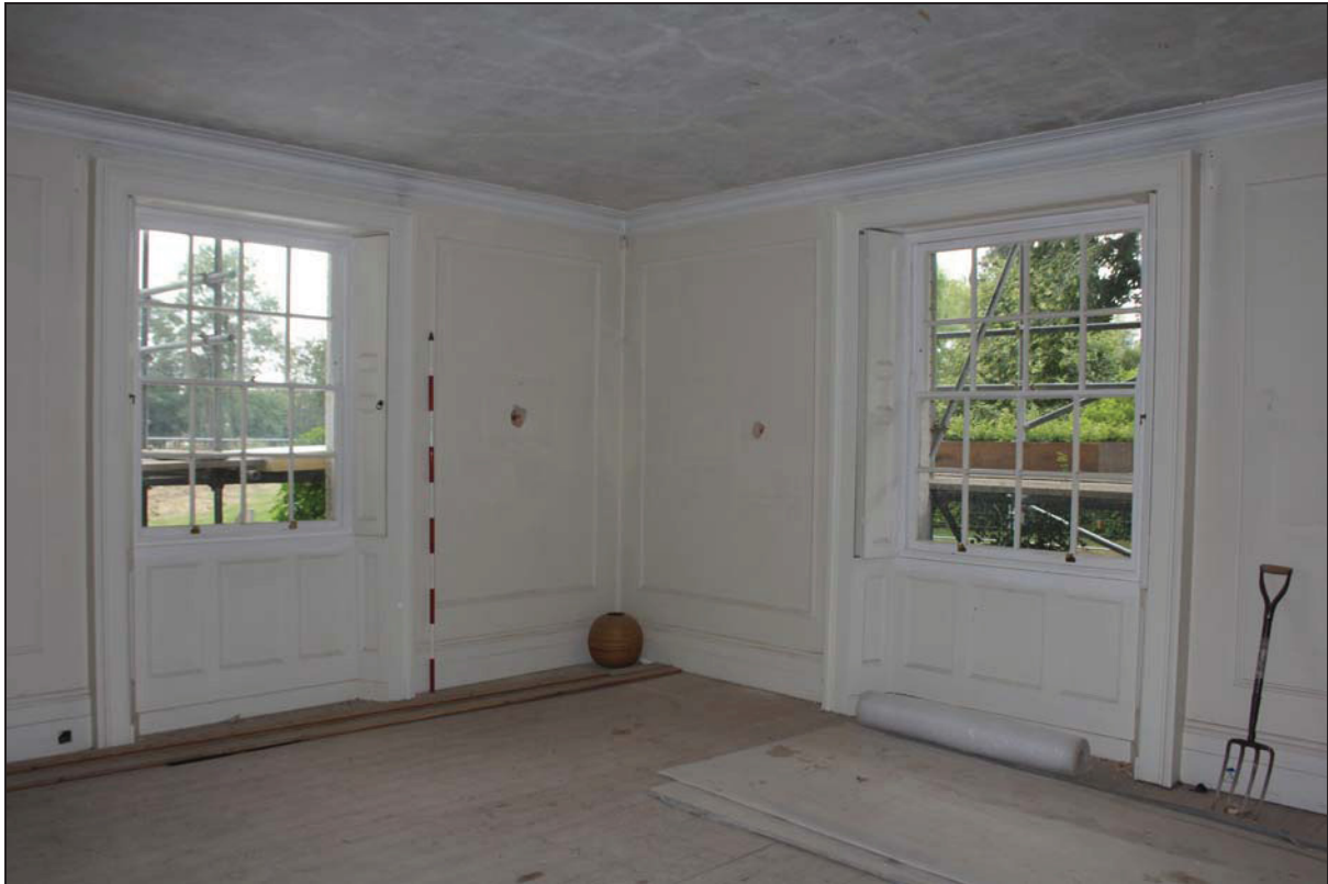
Plate 10 Sash windows with shutters on the west and south sides of Room GF03, taken from the north-east (DP55)
