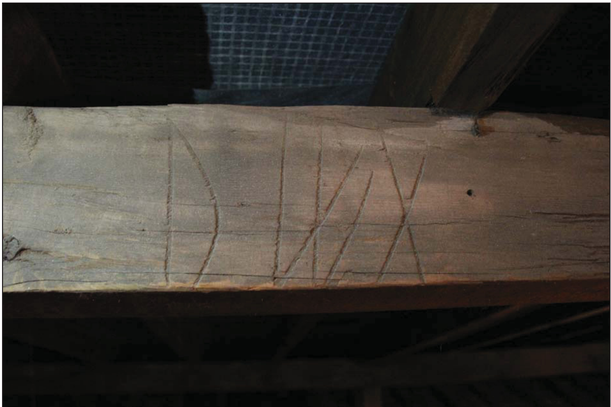
Plate 18 Scribed Baltic timber mark on a purlin in the roof structure (DP25)
