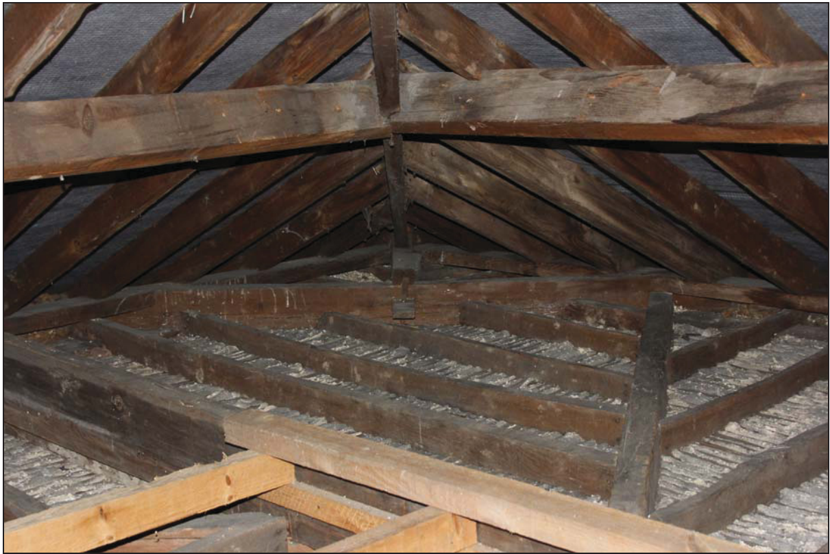
Plate 19 South-west corner of the roof space showing corner angle tie and ceiling structure to the room below, taken from the north-east (DP20)
