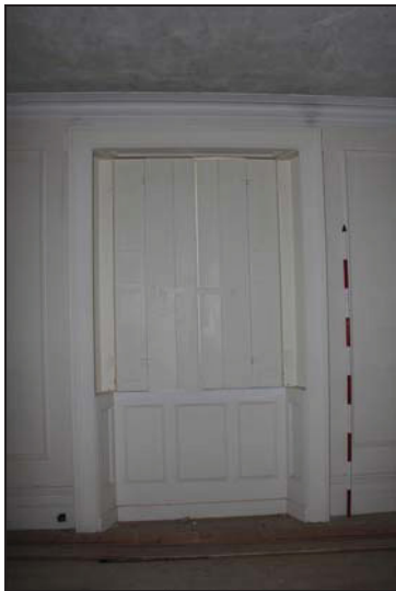
DP 57 Sash window with shutters on the south side of Room GF03, taken from the north
