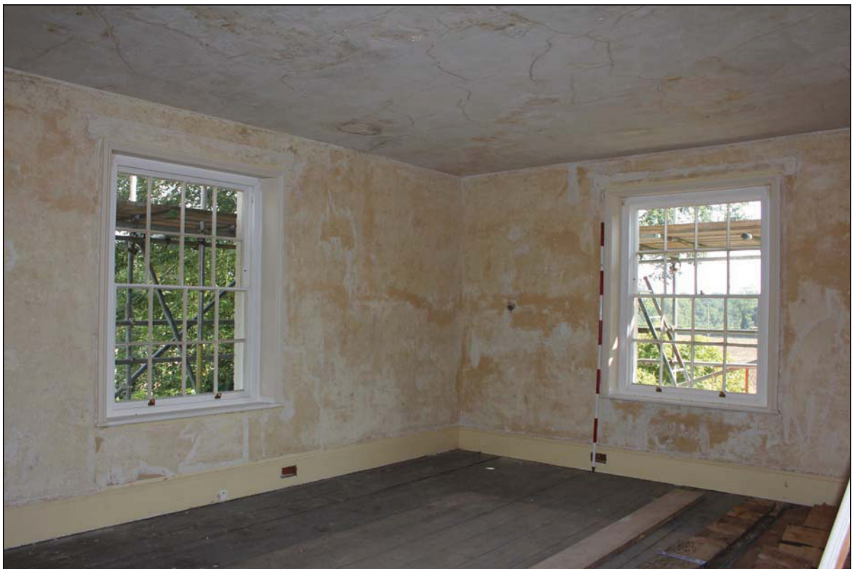
Plate 14 Windows on the east and south sides of Room FF05, taken from the north-west (DP91)
