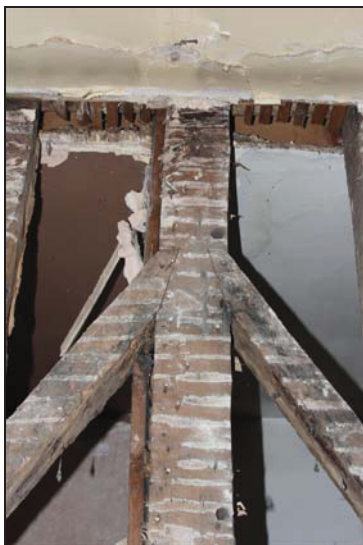
DP 5 Detail of the primary-bracing in Room GF05, taken from the north
