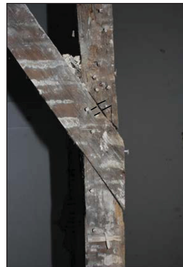
DP 6 Detail of the primary-bracing in Room GF05 showing setting out lines (emphasised), taken from the north
