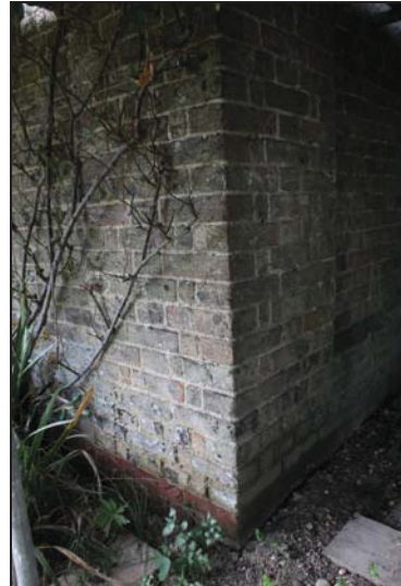
DP 34 Detail of the south-east corner showing red brick lower courses, taken from the south-east
