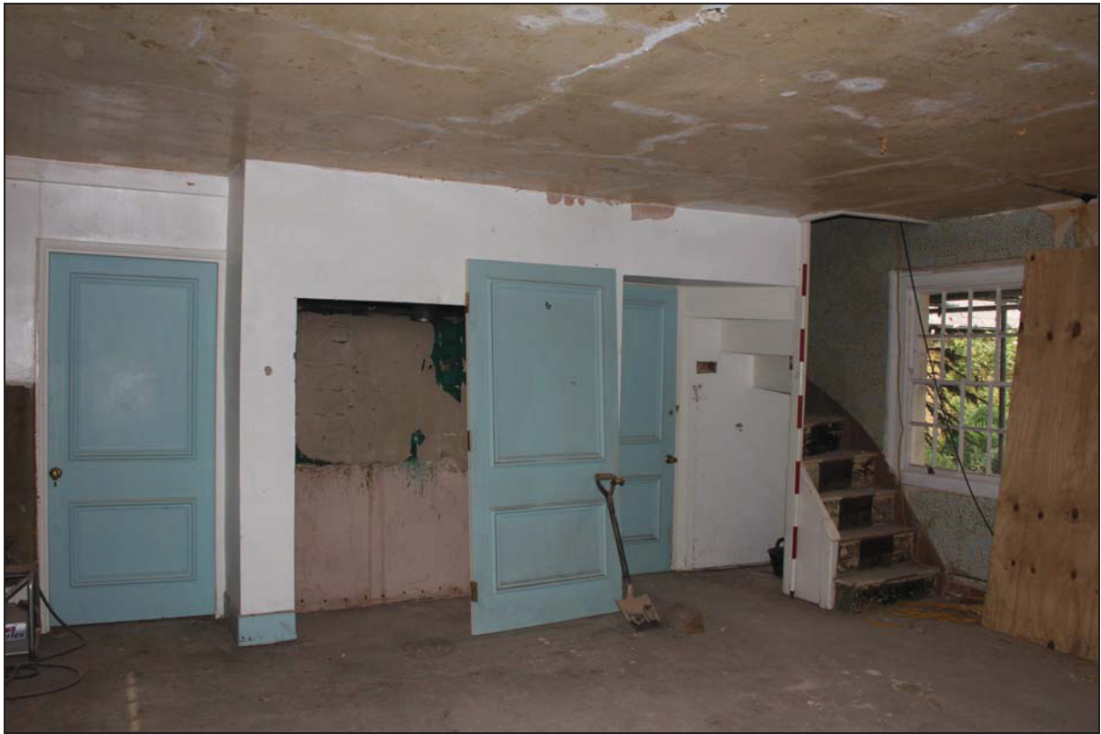
Plate 13 North side of Room GF06 (service range) showing kitchen fireplace, taken from the south (DP69)
