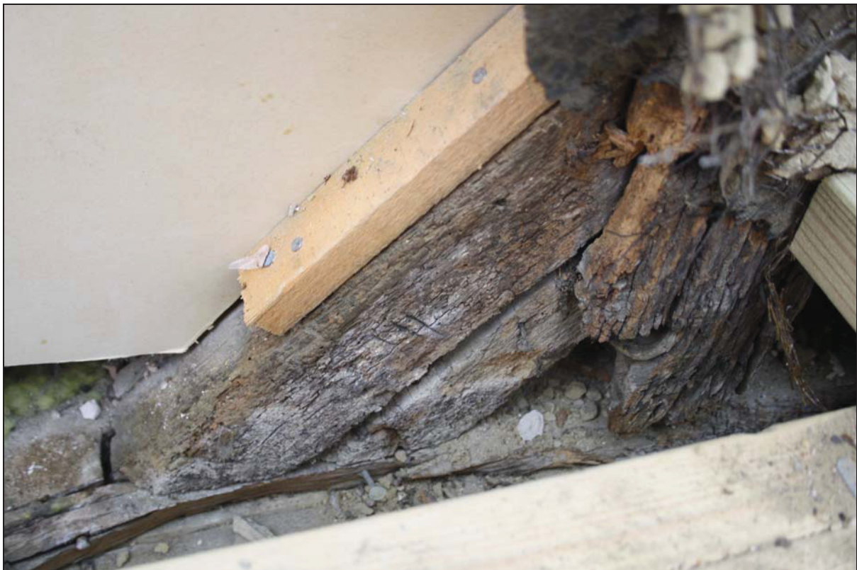
Plate 14 View of the timber-framing on the south-west side of Range 1 exposed during the planned works showing base of tension brace with assembly mark, taken from the south-west (DP 75)
