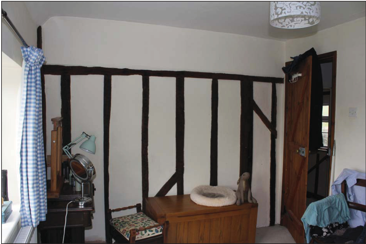
Plate 17 North-west wall of Room FF04 showing ephemeral primary-braced studwork and position of an inserted aperture later blocked, taken from the south-east (DP 35)
