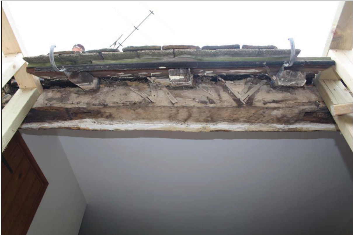
Plate 13 View of wall-plate on the south-west side of Range 1 exposed during the planned works showing stud mortices either side of a plain area, taken from the south-west (DP 77)
