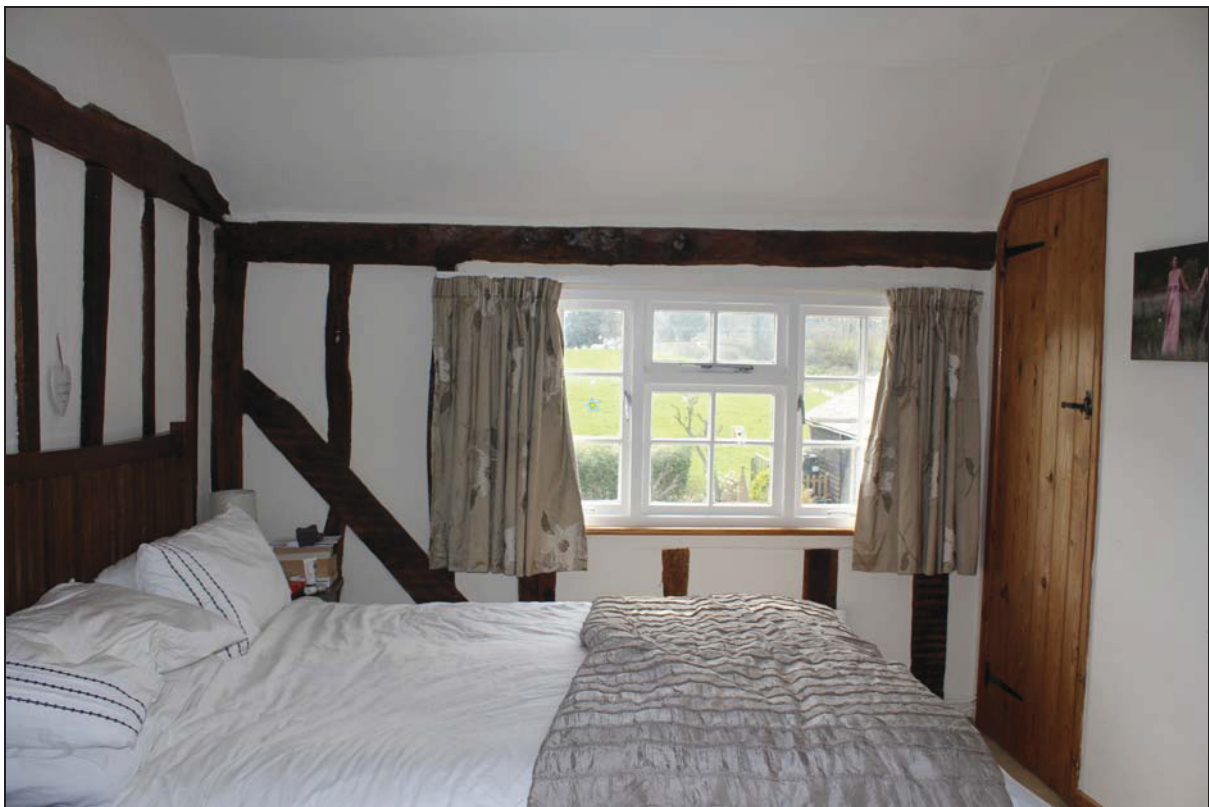
Plate 12 South-east wall of Room FF01 showing tension brace, taken from the north-west (DP 50)
