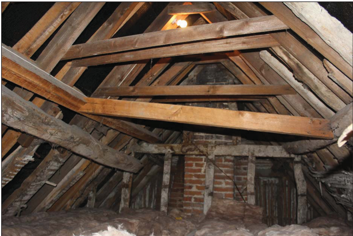
Plate 18 Roof structure over the historic core (FF01) showing clasped side-purlin form, taken from the south-east (DP 55)
