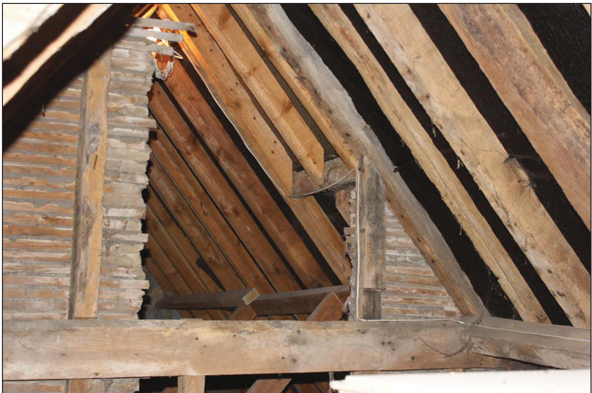
Plate 20 South-east end of the roof structure over Range 2 showing formerly external framing with external lath and plasterwork with area cut through to the modern roof structure over Range 3, taken from the north-west (DP 62)
