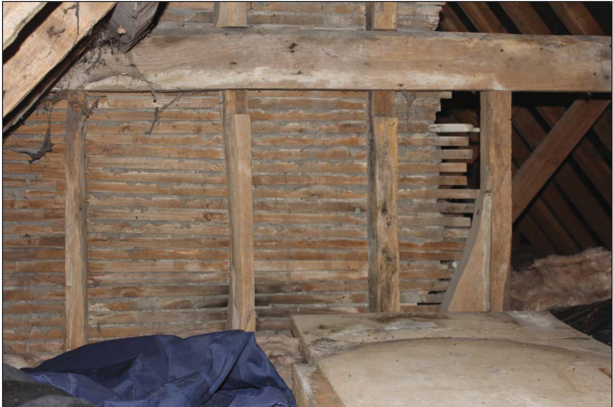
Plate 19 South-east end of the roof structure over Range 2 showing formerly external framing with external lath and plasterwork, taken from the north-west (DP 61)
