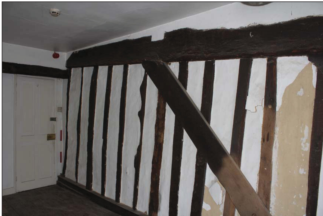
Plate 24 Timber-framing in FF02, showing a notch for a bridging joist in the tie-beam, taken from the north-east (DP 135)
