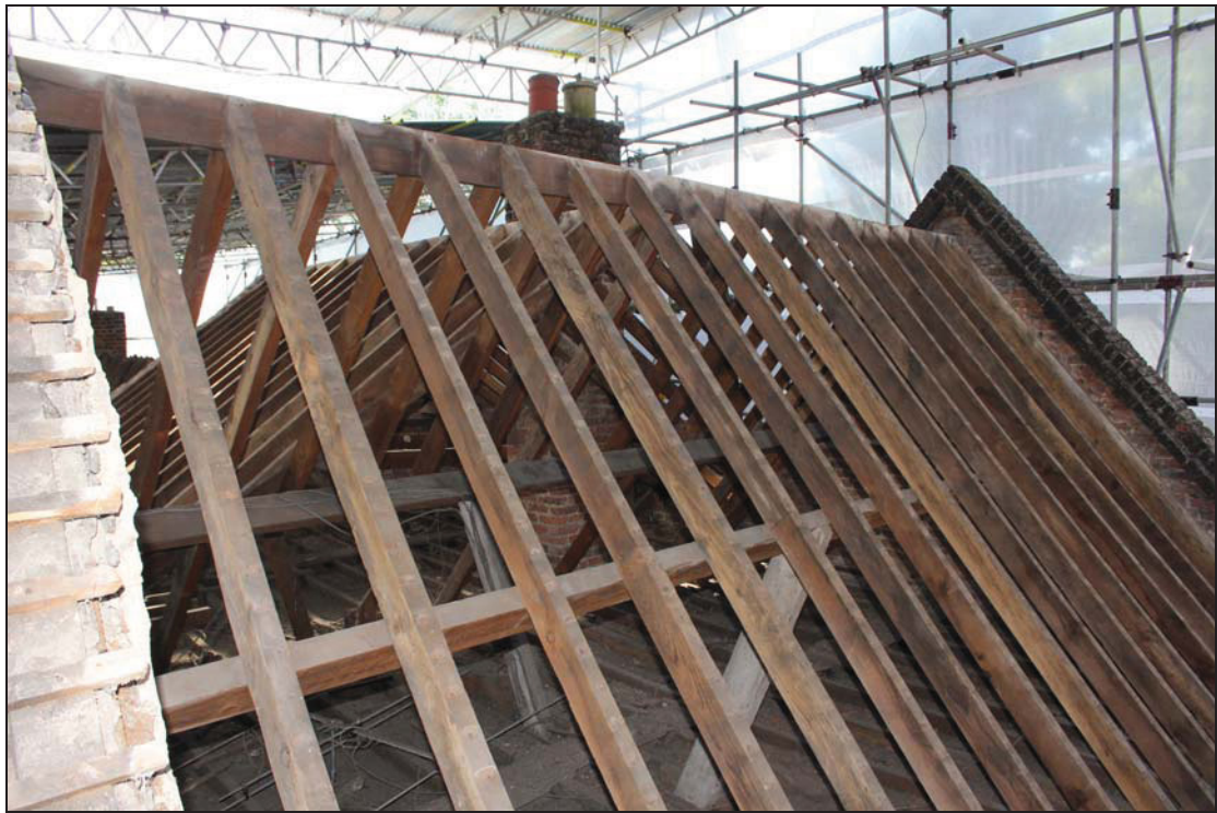
Plate 33 Roof structure of the front west roof, taken from the north-east (DP 233)
