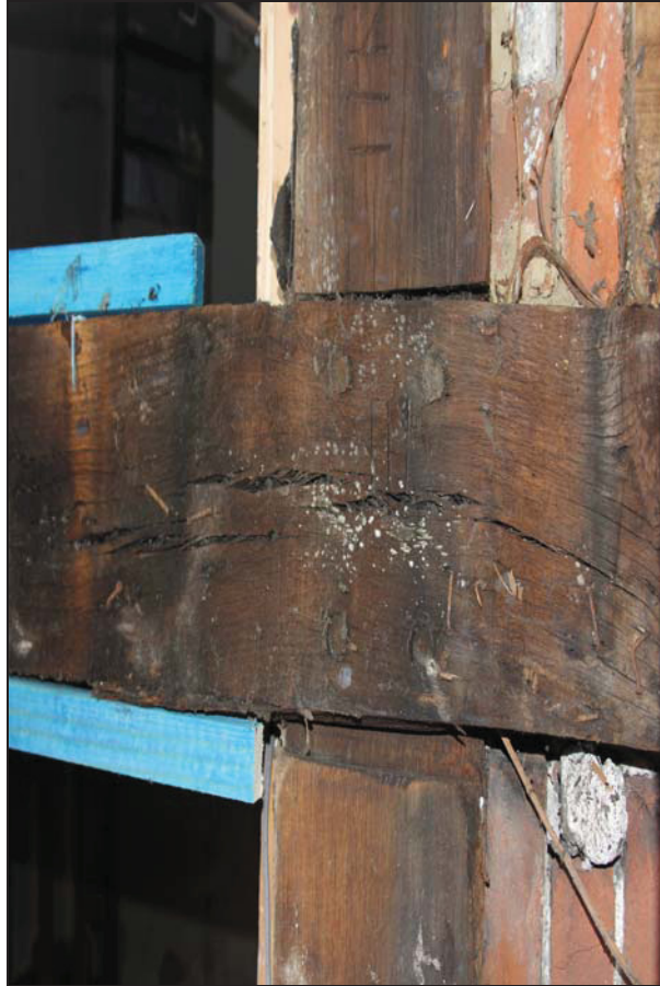
Plate 9 Detail of timber-framing with assembly marks along the western elevation of the rear range, taken from the west (DP 329)
