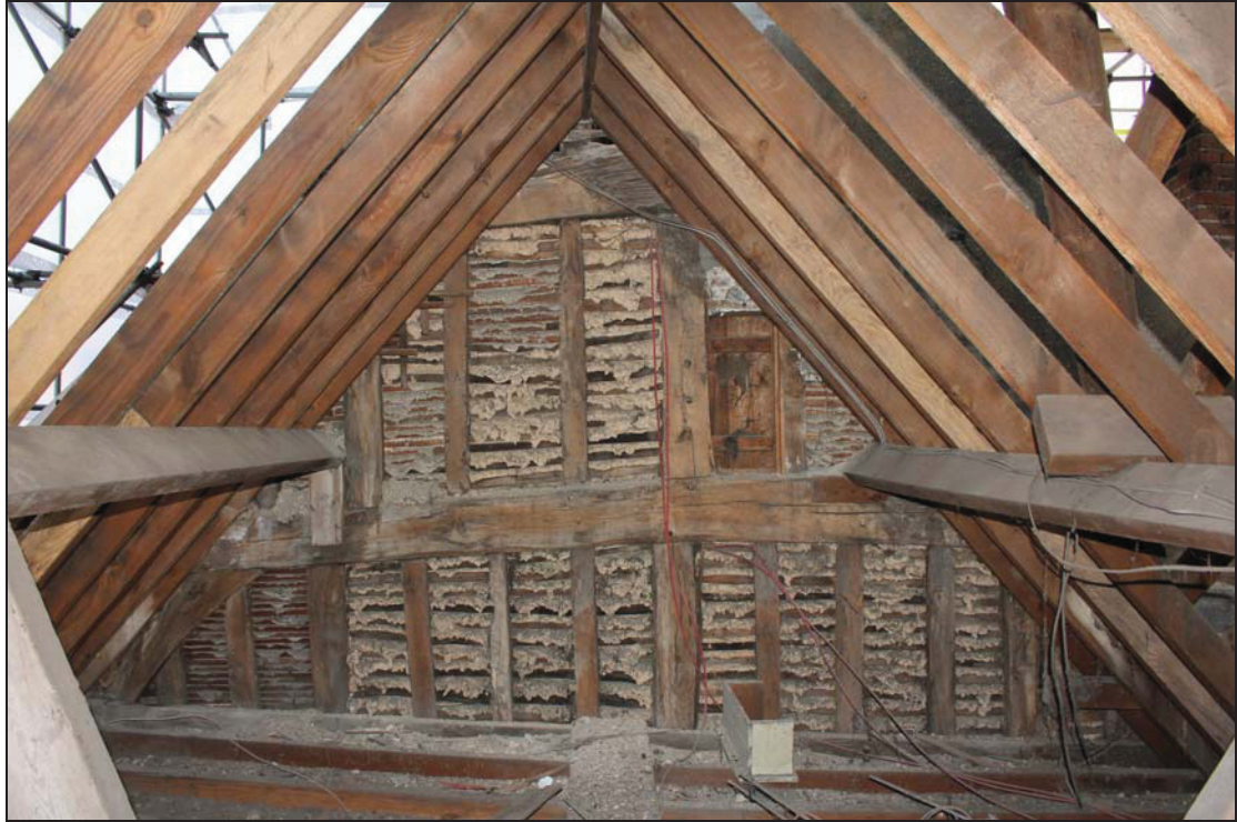
Plate 35 Gable end of the front west roof where it meets the east front roof, taken from the west (DP 238)
