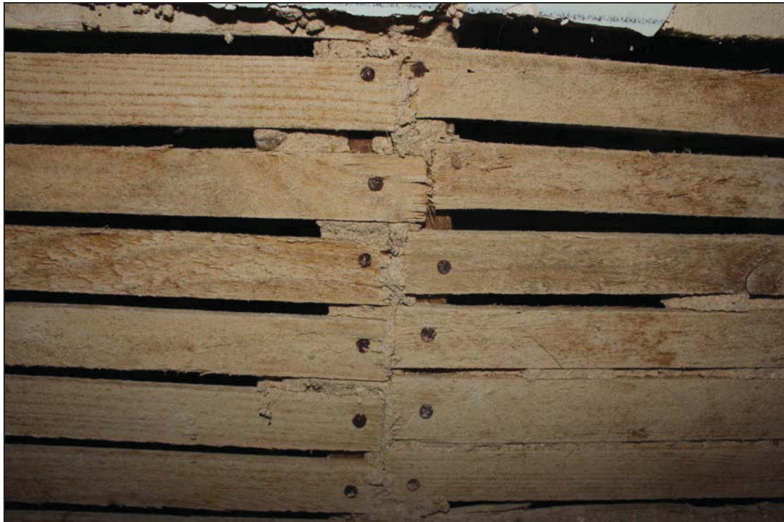
Plate 30 Previously hidden lath and plaster in FF05, taken from the west (DP 269)
