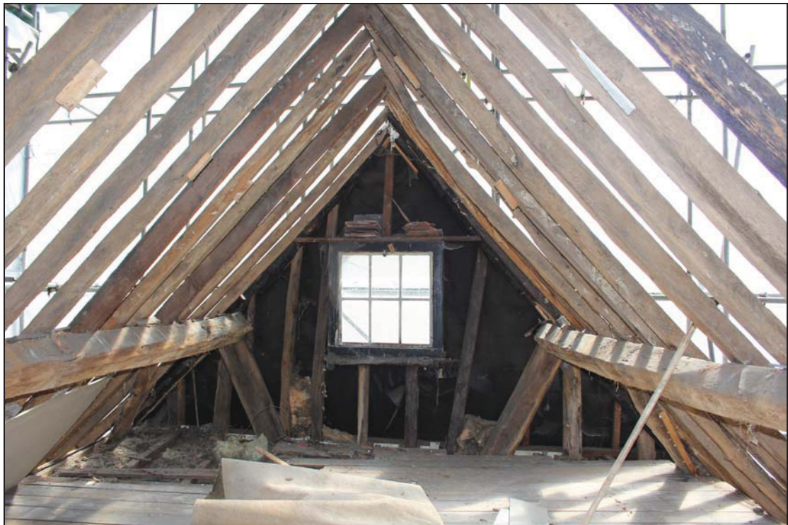
Plate 56 South gable end of the rear range at roof level, taken from the north (DP 256)
