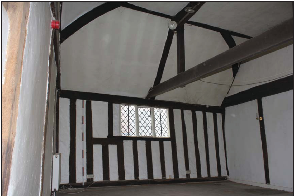
Plate 28 Interior of FF04, showing timber-framing on the north wall, taken from the south (DP 142)
