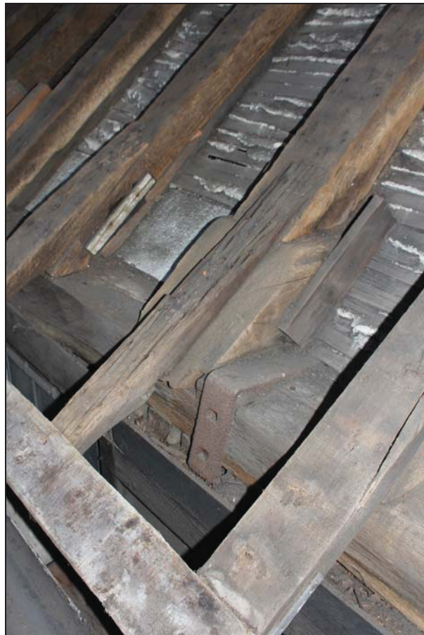
Plate 54 Rafter feet in the rear range and 18 th century strap to the wall plate, taken from the south-west (DP 201)
