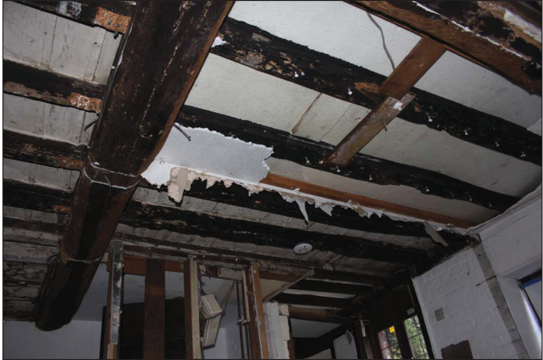
Plate 39 Ceiling joists in the area between GF06 and GF08, partitions now removed, taken from the south (DP 249)
