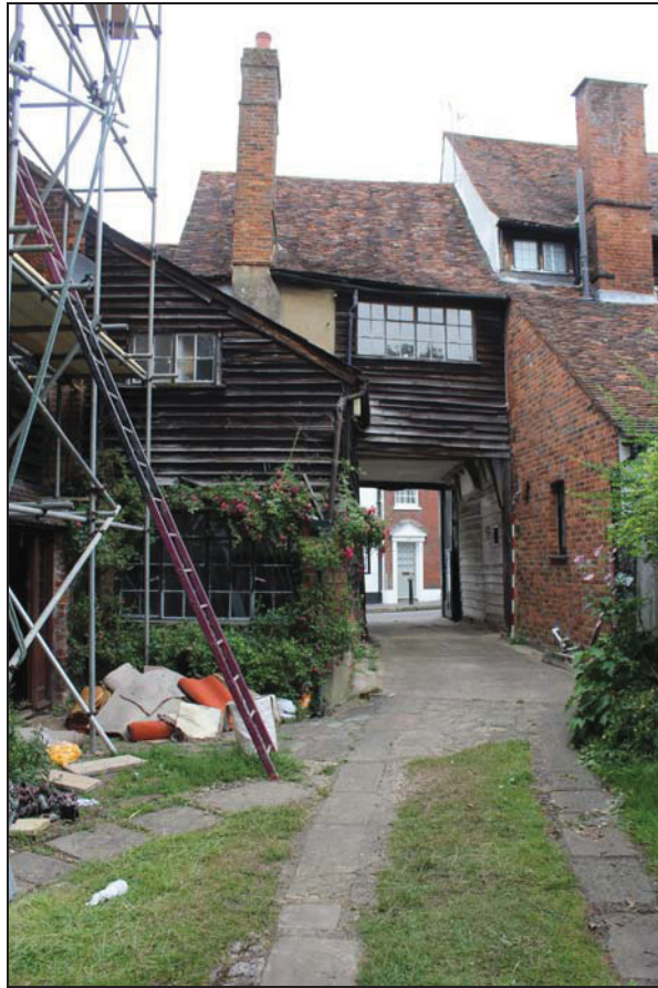
Plate 5 Rear of the front range and rear intermediate range, with pent-roof push-out, taken from the south (DP 013)
