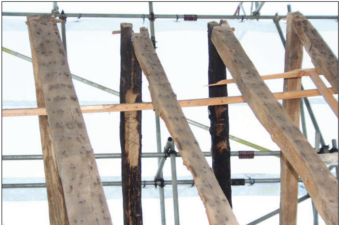
Plate 52 Detail of rafter couples in the rear range with assembly marks, taken from the east (DP 222)
