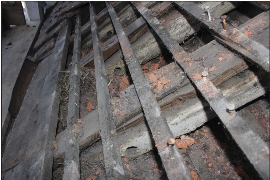
Plate 36 Rafter holes in the rafters of the east front roof, taken from the north-west (DP 229)
