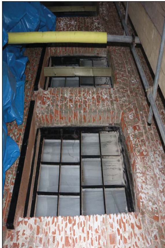
Plate 2 Brick fabric on the front range exposed during monitoring of works, taken from the north-west (DP 355)
