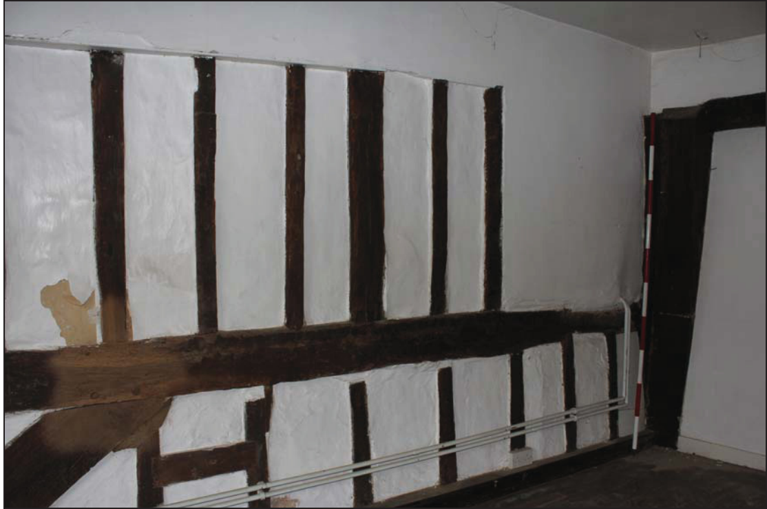
Plate 25 Timber-frame in FF02 with several members rising from the ground floor room below, taken from the north-west (DP 140)
