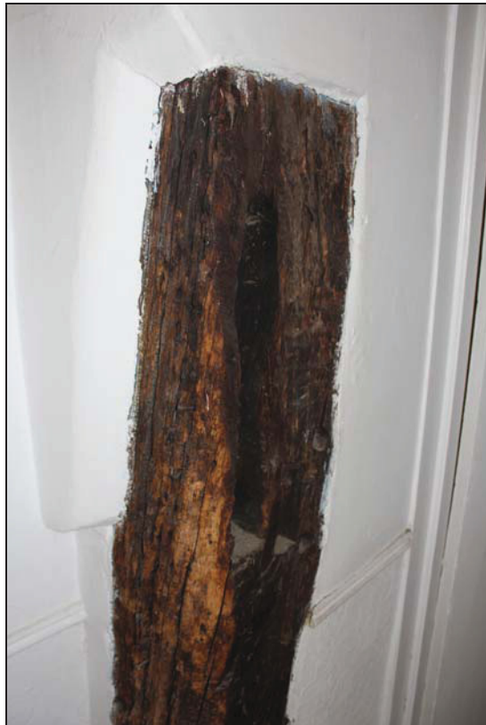
Plate 32 Timber-framing in FF06, a principal post with a mortise for a downward brace, taken from the north-east (DP 123)
