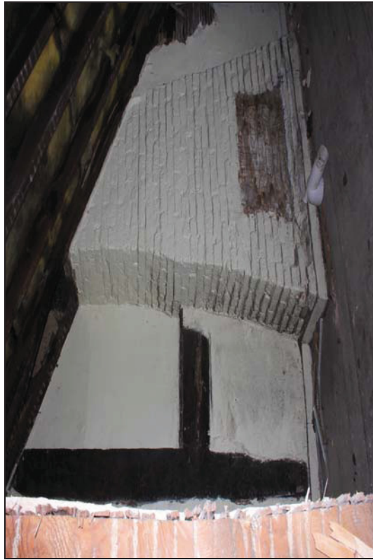
Plate 31 View of FF06, with timber-framing truncated by the chimney stack, taken from the south-west (DP 267)
