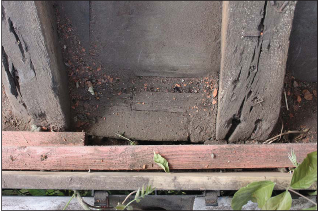
Plate 51 Scarf joint in the wall-plate of the rear roof range, mid-bay in Bay 4, taken from the east (DP 244)
