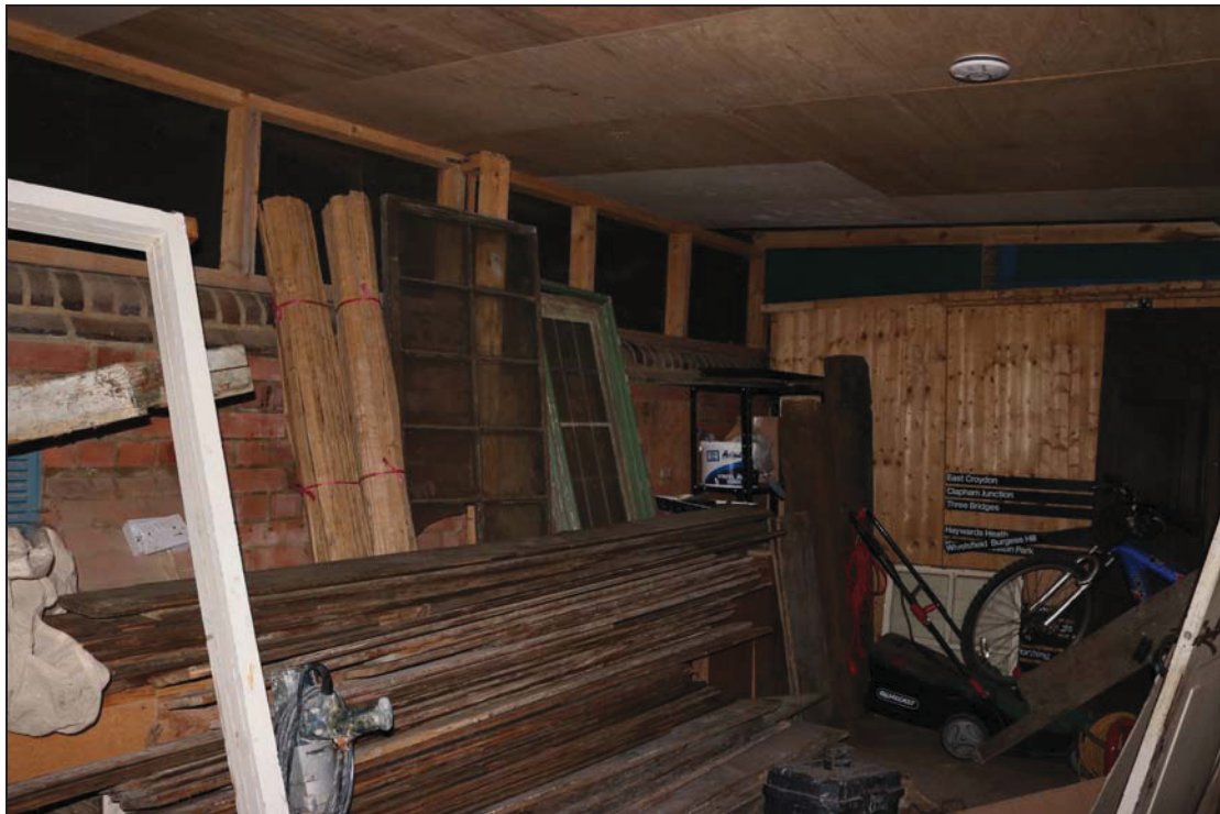
Plate 10 Interior of the workshop in the outbuildings, taken from the north-west (DP 366)
