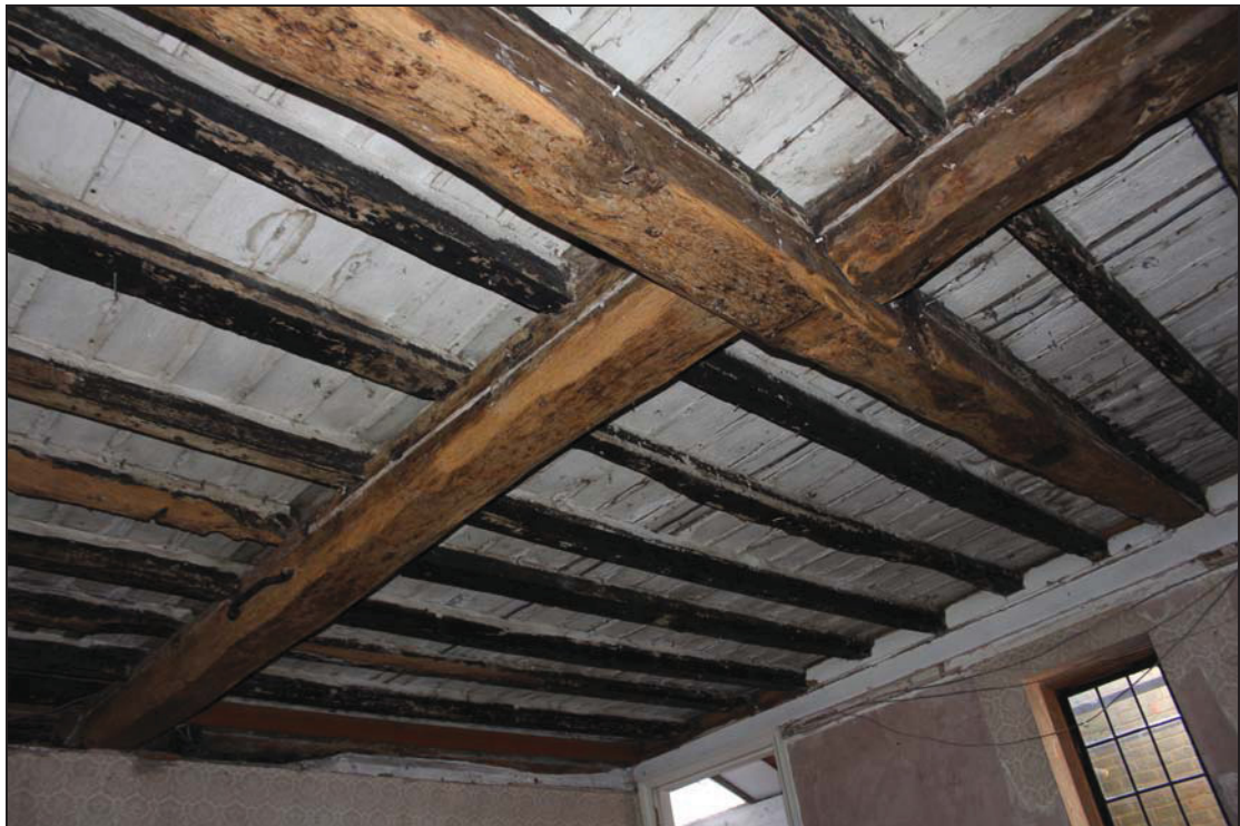
Plate 38 Ceiling joists of GF08 exposed during monitoring of works, taken from the north-east (DP 245)
