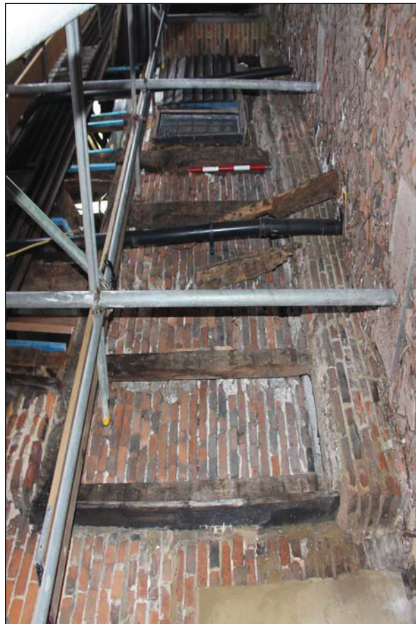
Plate 8 Hidden fabric revealed along the western elevation of the rear range, taken from the north-west (DP 323)
