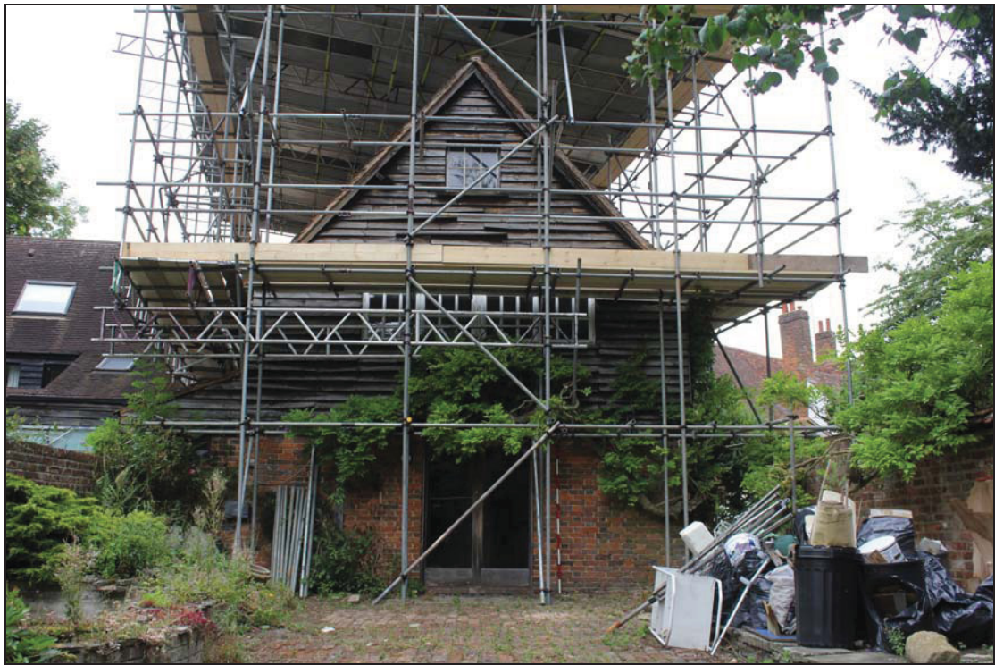
Plate 7 South gable end of the rear range, taken from the south (DP 018)
