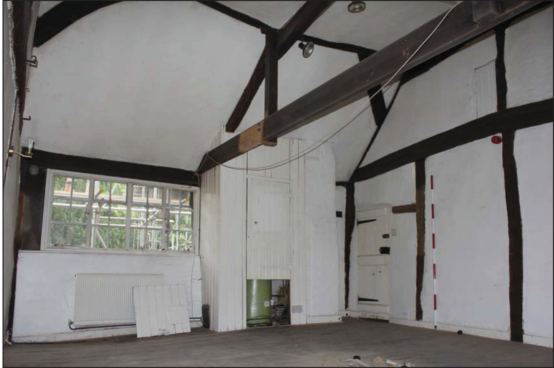
Plate 27 Interior of FF04, showing the roof structure over this range, taken from the north-east (DP 149)
