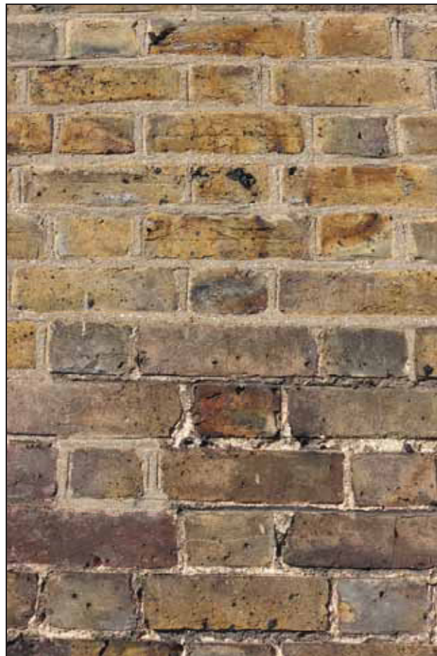
Plate 6 Detail of brickwork to the rear of the hotel, showing the raising of this previously single-storey extension, taken from the west (DP 024)
