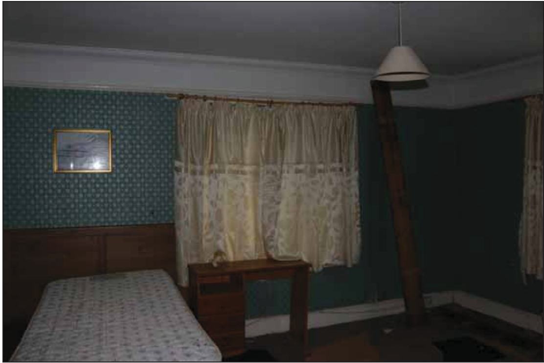
Plate 15 Room 5 on the first floor of the hotel, taken from the east (DP 084)
