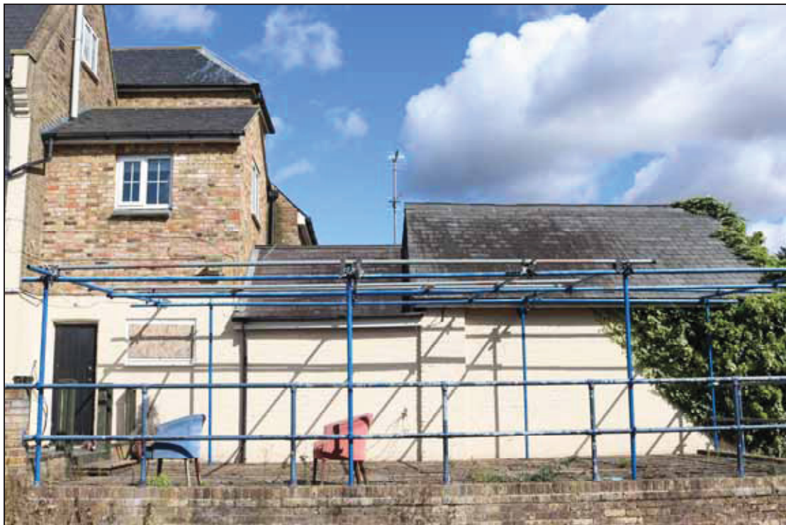
Plate 8 Partial view of the hotel's south elevation, taken from the south (DP 027)
