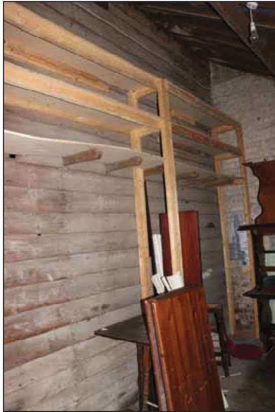
Plate 19 Weather-boarding in the interior of the outbuilding, taken from the south-west (DP 101)
