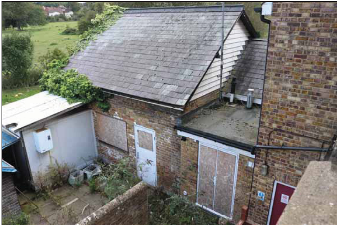
Plate 7 View of kitchen block from a first floor window in the hotel, taken from the north-west (DP 104)
