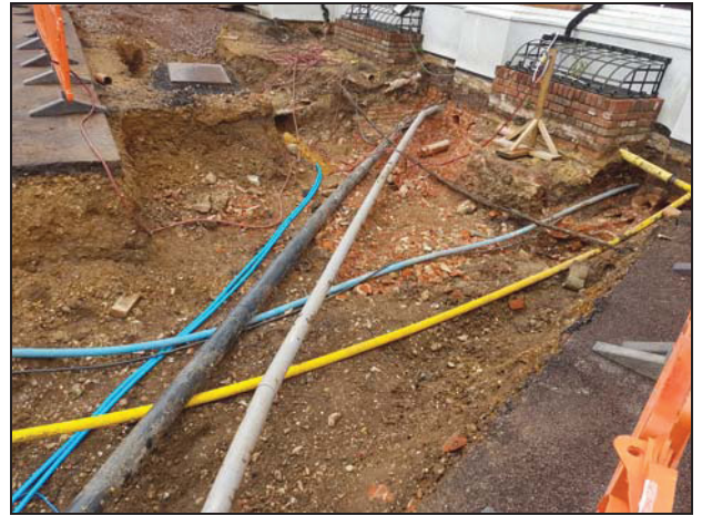
2 East end of the southern service trench (south-west corner of house), looking north-east
