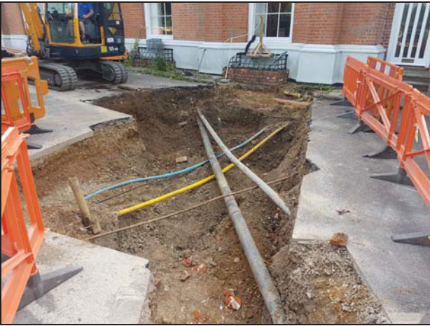
1 East end of the southern service trench (south-west corner of house), looking east
