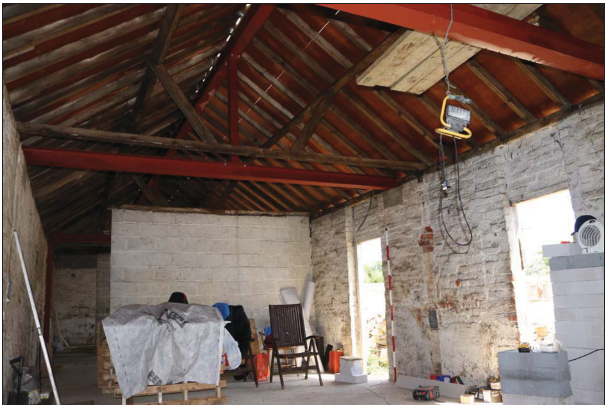
Plate 8 Bays 4 and 5 (Building 1) showing secondary timber truss (Truss 4) and recent inserted steel truss, taken from the west (DP 40)
