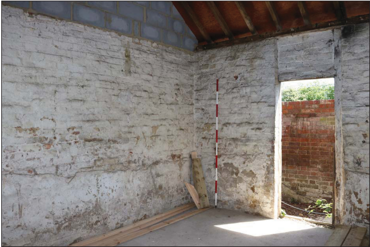
Plate 5 Bay 1 (Building 1) showing painted outer walls with cement render at low level, taken from the north-west (DP 29)
