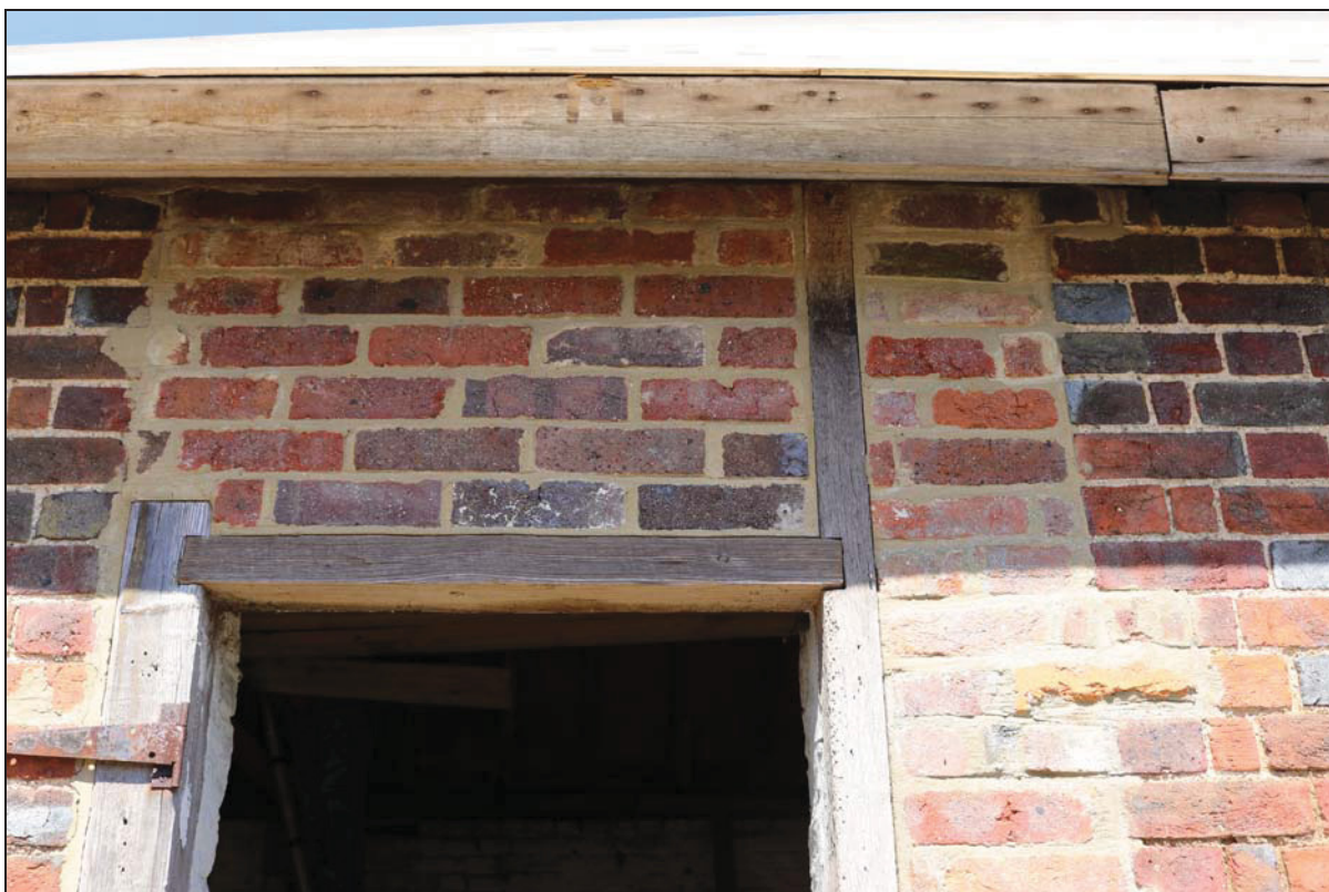
Plate 4 Detail of a doorway on the south side of Building 1 showing evidence for the reduction in doorway size, taken from the south (DP 13)
