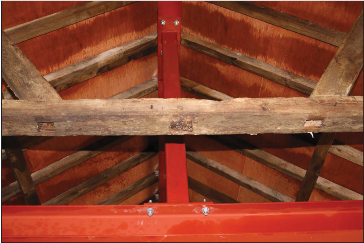
Plate 9 Detail of Truss 4 (Building 1) showing mortices for a lower studwork partition, taken from the west (DP 42)
