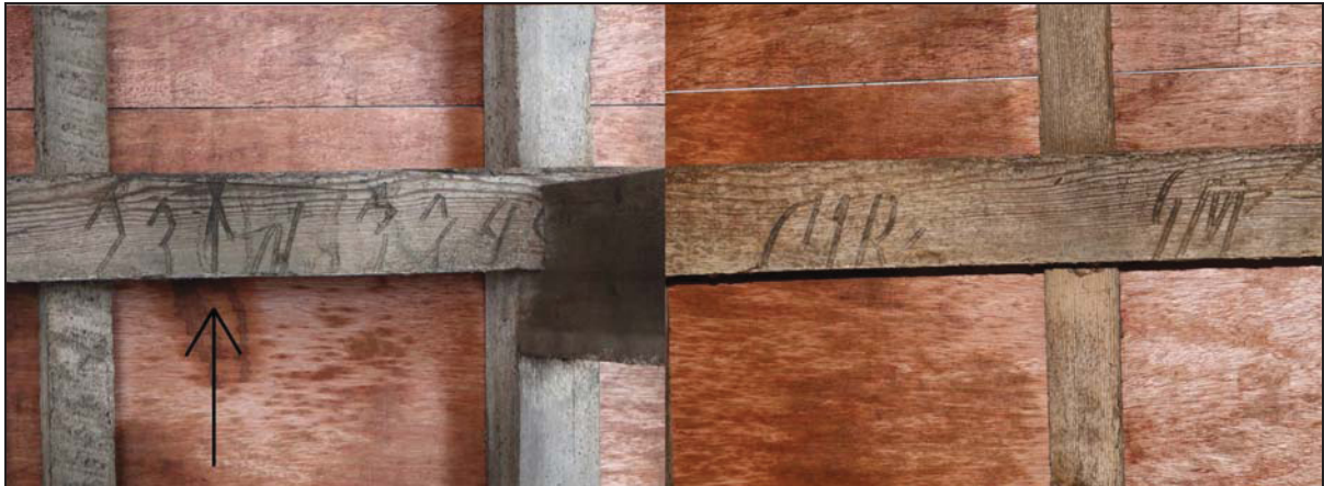
Plate 7 Composite image showing detail of the north purlin between Bays 1 and 2 (Building 1) showing Baltic bracking mark including the symbol for the port of Gdansk (indicated), taken from the south (DPs 33-34)
