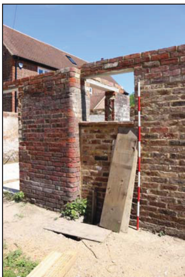
DP 17 West elevation of Building 2 at the junction between Unit 1 and 2, taken from the south-west
