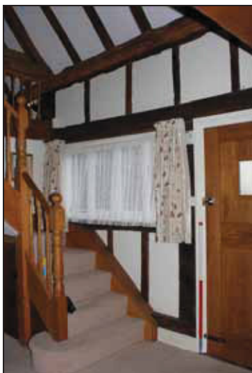
DP 29 North-west side of Bay 2 showing rebuilt fabric including the modern window that replaced an earlier 20 th century larger example in order to accommodate the staircase, taken from the east
