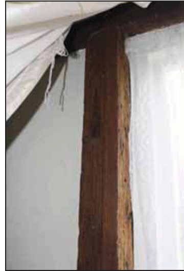
DP 26 North-west side of Bay 1 showing wattle notch, taken from the east
