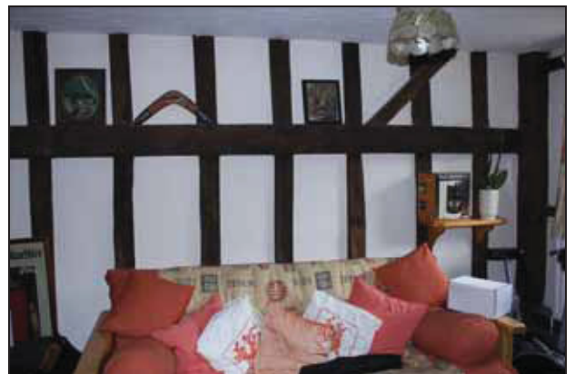
DP 18 South wall of Bay 3 showing mid-rail with upper and lower pegged studs with tension brace on the right, taken from the north-east
