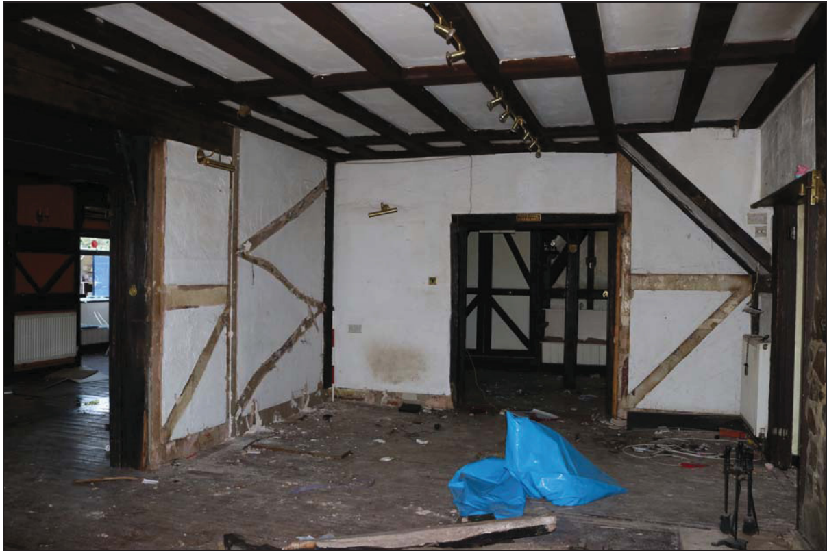
Plate 7 East end of Room GF03 showing fictive timber framing removed, taken from the south-west (DP 21)
