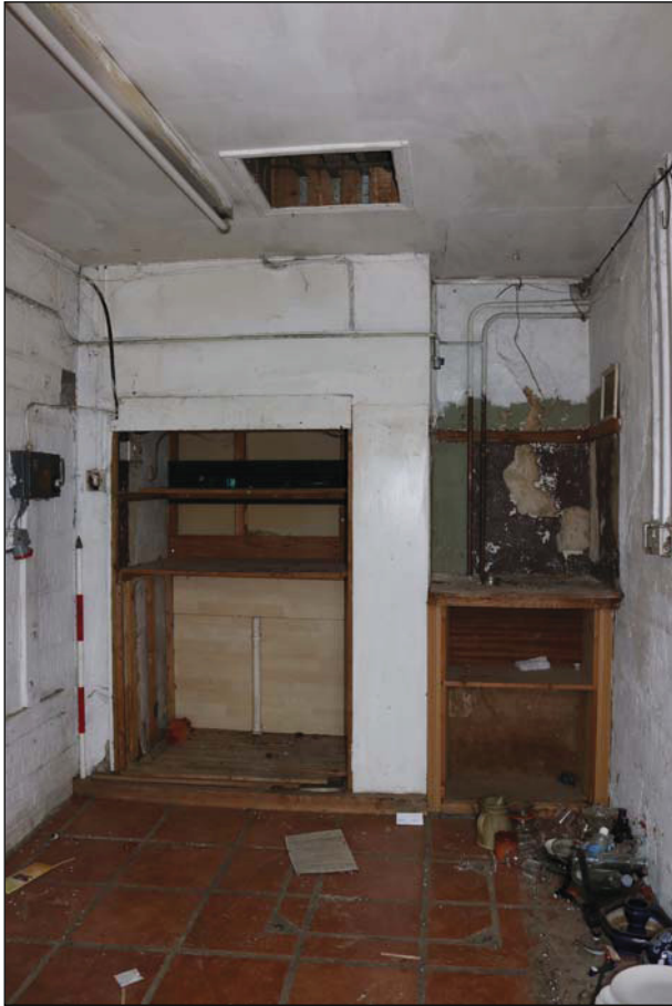
Plate 5 Former fireplace on the west side of Room GF06, taken from the east (DP 40)
