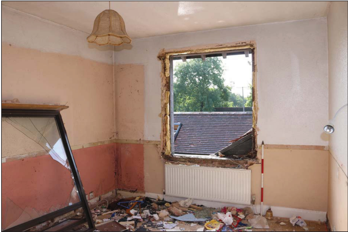
Plate 9 Room FF02 following removal of the window, taken from the north-west (DP 58)
