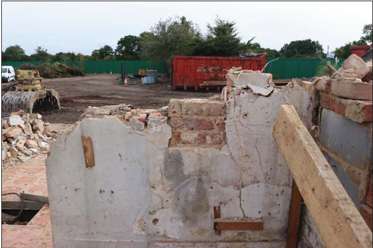
Plate 13 East side of the building during demolition showing rear of chimney stack with some earlier brickwork, taken from the west (DP 52)
