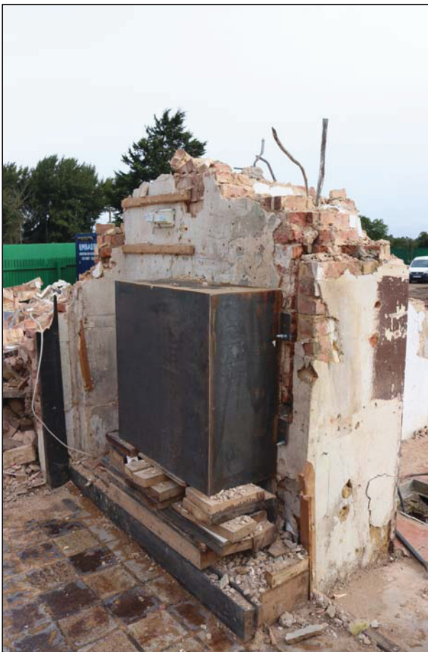
Plate 12 Eastern side of the building during demolition showing mix of Fletton brickwork with occasional earlier bricks, taken from the south-west (DP 51)
