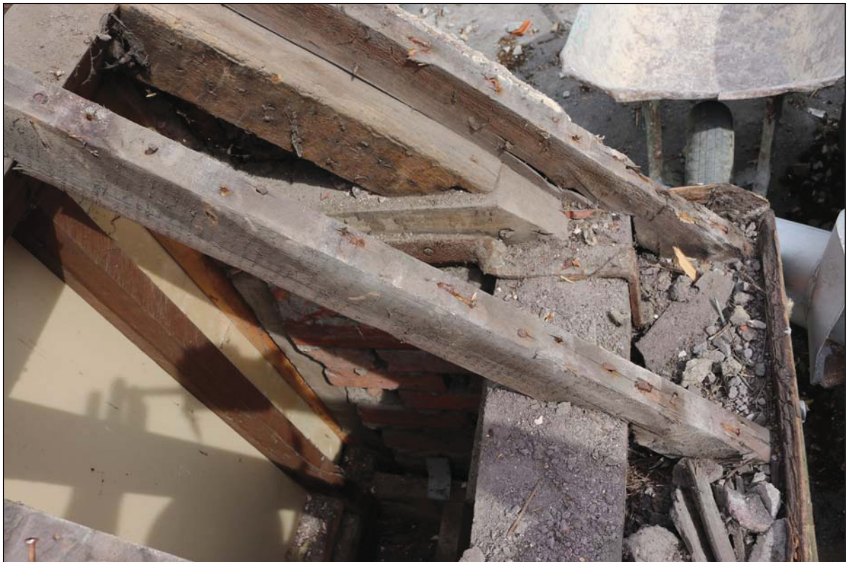
Plate 4 Detail of the east pitch (north-east range) after removal of the roof cladding showing iron-strapped wall-plate and tie-beam, taken from the east (DP 115)
