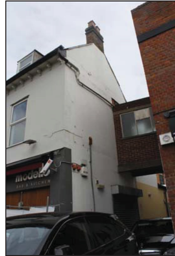
DP 8 East side of the main street front range, taken from the south-east
