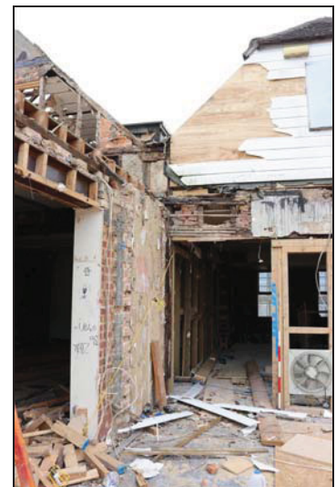
DP 122 North elevation of the north-west rear range following removal of the first floor extension, taken from the north
