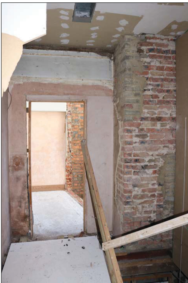
Plate 10 East end of FF01 showing inserted doorway in the east end following removal of the modern lift (main range), taken from the west (DP105)
