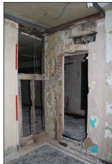
DP 72 North-east corner of FF03 (north-east range) showing truncated original mid-rails with studs above and below, taken from the south-west
