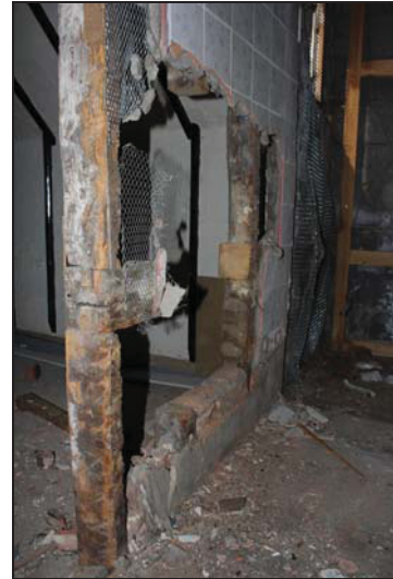
DP 26 Detail of the formerly external north gable end (north-east range) showing truncated timbers, taken from the north-east
