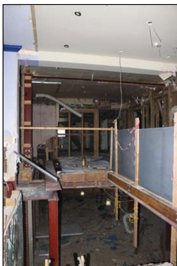
DP 103 FF02 (west range) following removal of the staircase, taken from the south
