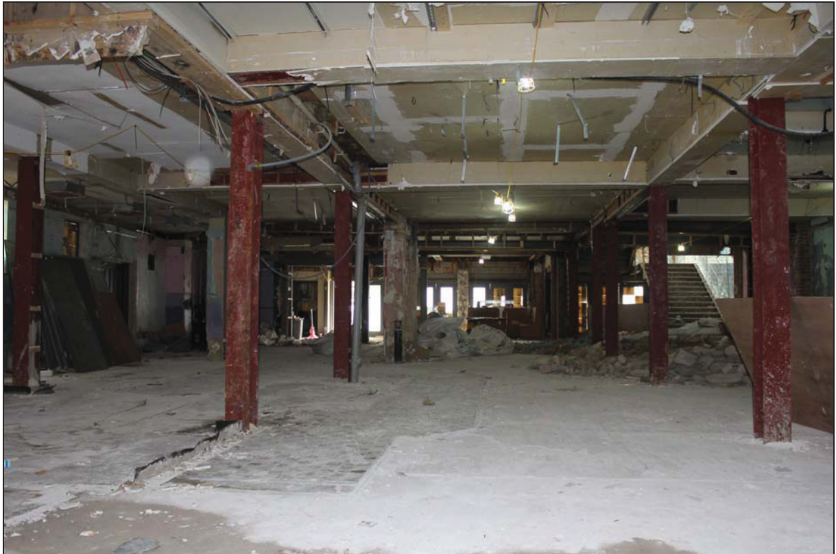
Plate 7 View at ground floor level from the rear extensions towards the street front, taken from the north (DP 92)
