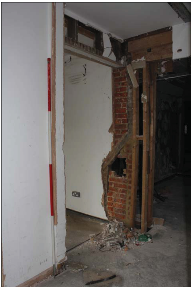
Plate 9 View of FF01 showing fragmentary surviving timber-framing and brickwork infill of the rear wall (main range), taken from the south (DP 60)
