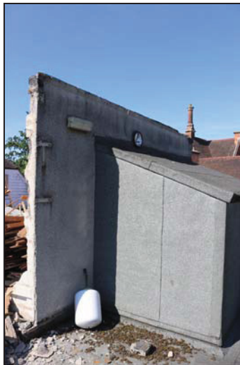
DP 101 South wall of the modern second floor extension during its removal, taken from the north-east
