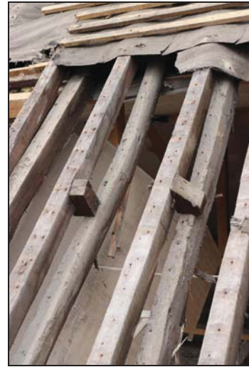
DP 118 View of the east pitch (north-west range) after removal of the roof cladding showing two phases of rafters, taken from the east
