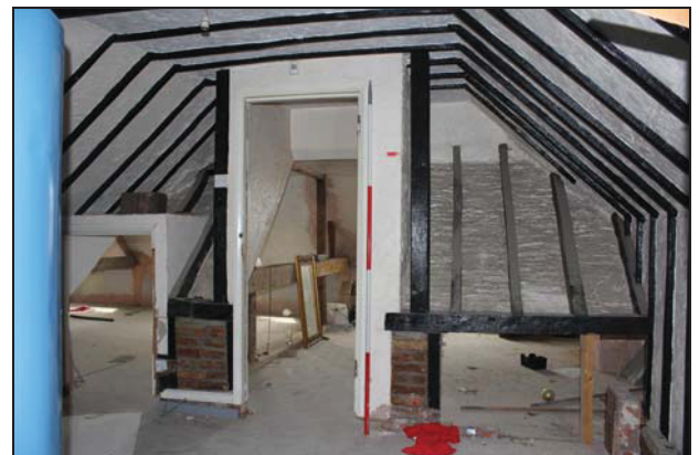
DP 30 South side of Room SF03 (north-east range) showing timber framing on the north side of the main range (east element), taken from the north
