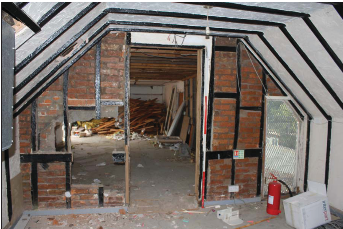
Plate 16 North wall of Room SF03 (north-east range) showing surviving timber infilled with brickwork, taken from the south (DP 29)
