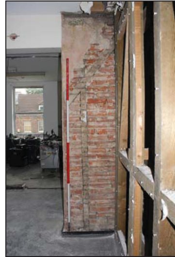
DP 68 Fragments of timber-framing surviving in the rear wall of the main range, taken from the north
