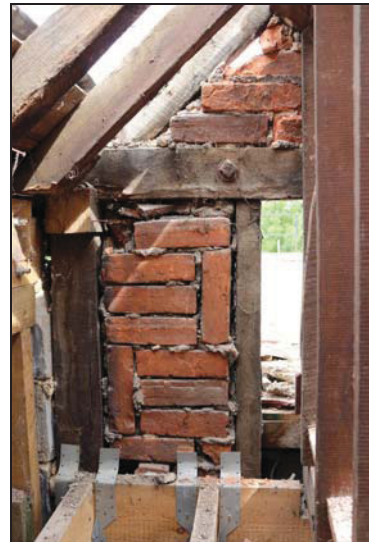
DP 120 Detail of the north-west corner (north-east range) showing bolted wall-plate with brick infill below, taken from the south
