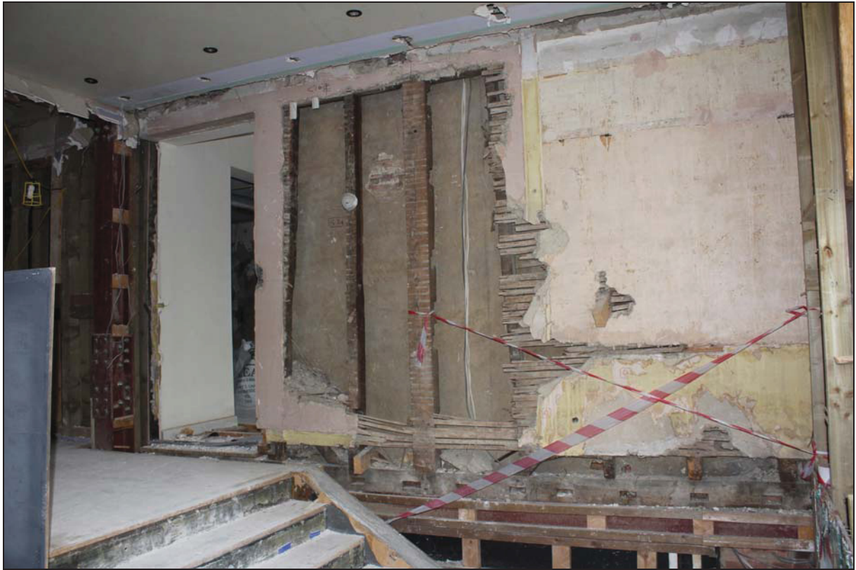
Plate 11 East wall of FF02 (west range) showing studwork constructed against pre-existing fabric, taken from the west (DP 51)
