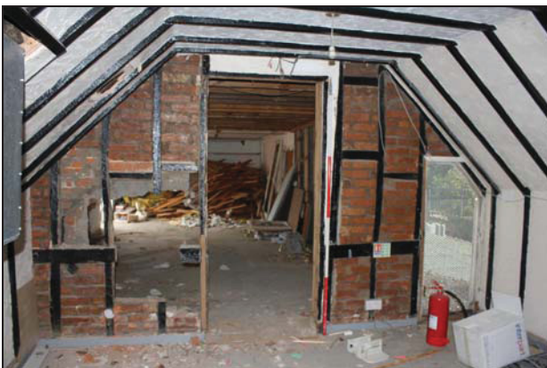
DP 29 North wall of Room SF03 (north-east range) showing surviving timber infilled with brickwork, taken from the south
