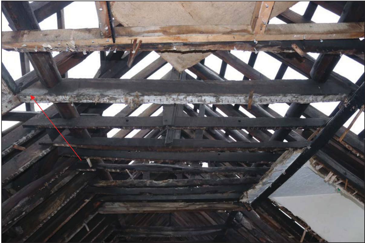
Plate 21 Roof structure over Bay 4 (SF02) showing intermediate pegged collar (indicated) and additional nailed collars, taken from the west (DP 148)
