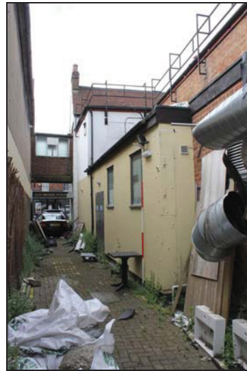
DP 10 East side of the building showing ranges extending to the rear, taken from the north
