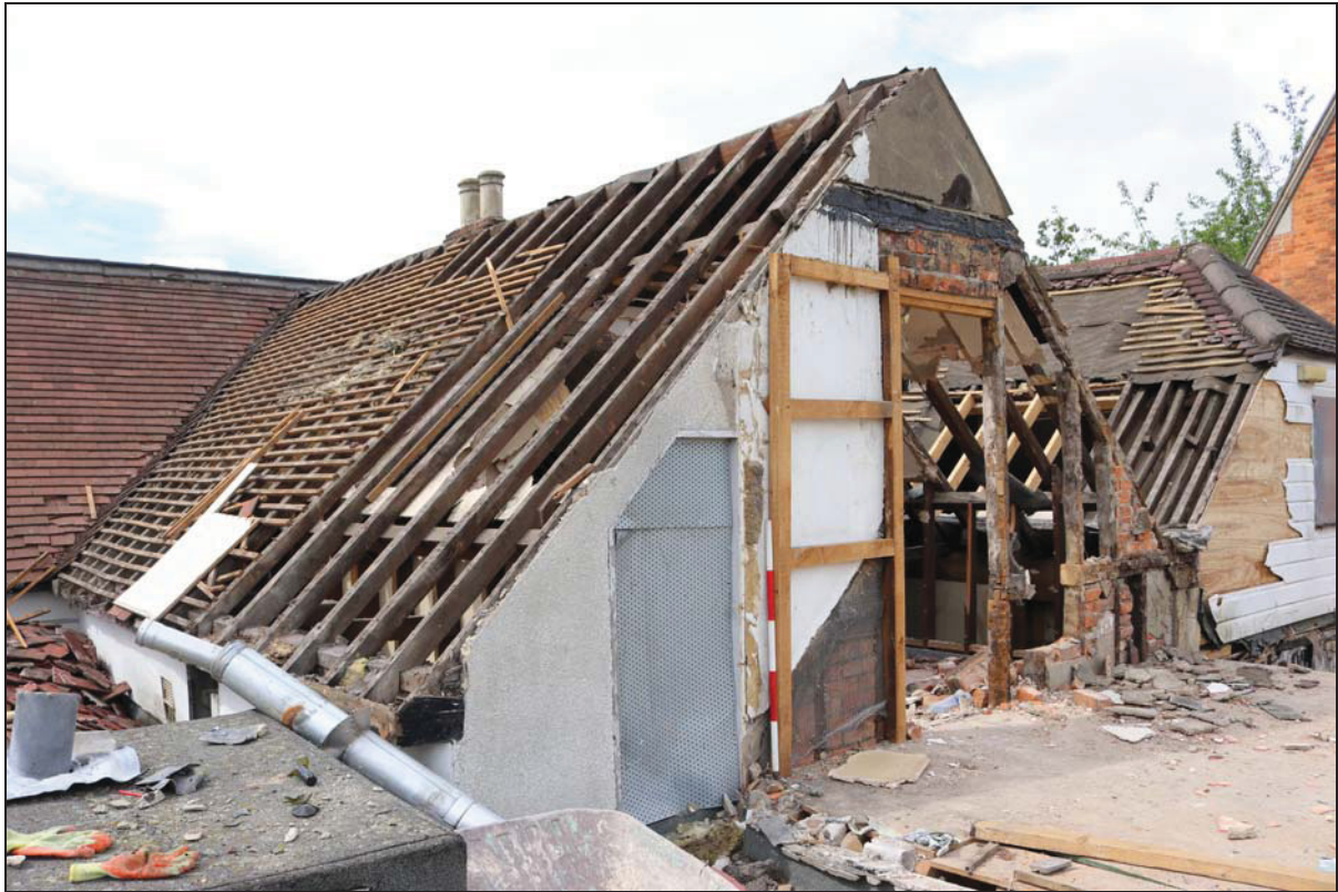
Plate 3 View of the north-east range after removal of the roof cladding, taken from the north-east (DP 112)
