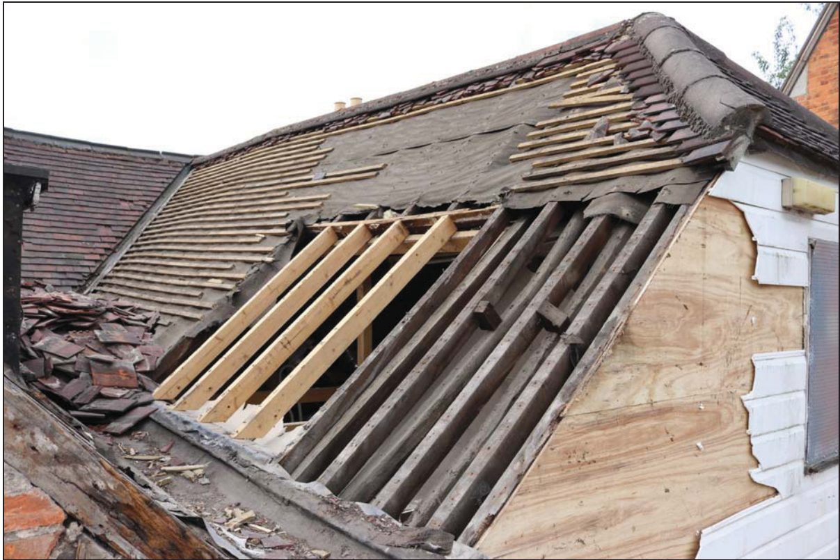
Plate 5 View of the north-west range after partial removal of the roof cladding, taken from the north-east (DP 117)
