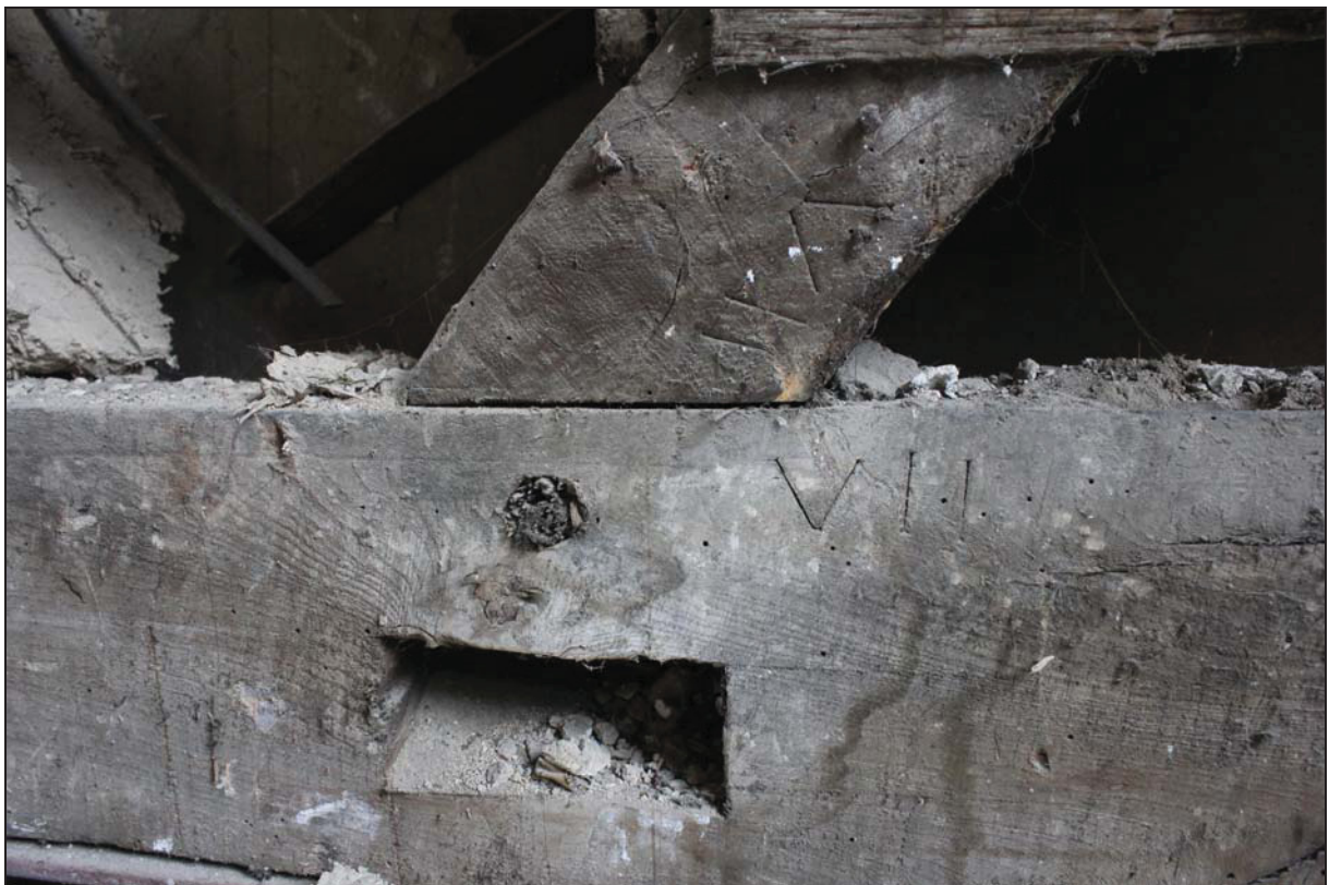
Plate 12 East side of FF02 (west range) showing assembly marks on the binding joist and primary brace, taken from the west (DP 54)
