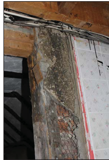
DP 28 Detail of the formerly external north gable end (north-east range) showing pebble-dashed render, taken from the north
