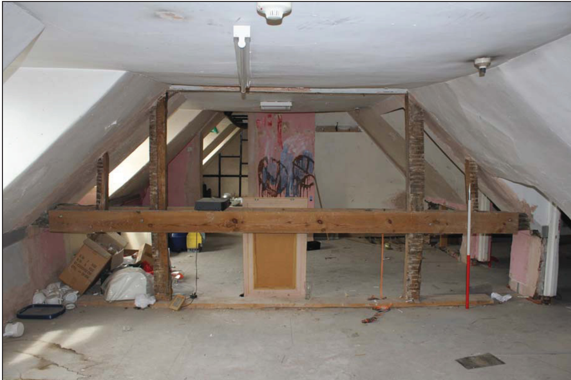
Plate 15 View of the attic space (SF01) over the main range, taken from the east (DP 38)
