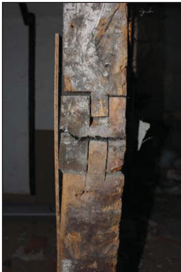
DP 27 Detail of the formerly external north gable end (north-east range) showing horizontal member truncated to expose the jointing of the upper and lower studs, taken from the east
