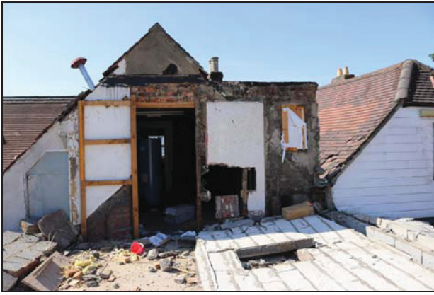
DP 99 View of north elevation of the north-east rear range following removal of the modern extension, taken from the north
