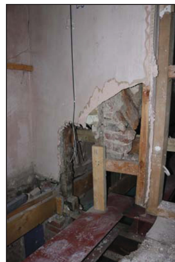
DP 104 North side of FF04 (north-west range) showing surviving timber elements exposed during the planned works, taken from the south
