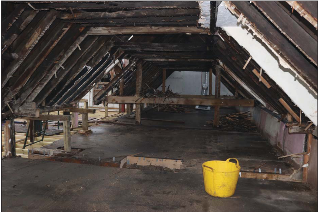
Plate 17 View of the attic space after the removal of lath and plasterwork and the studwork on the north, taken from the west (DP 147)
