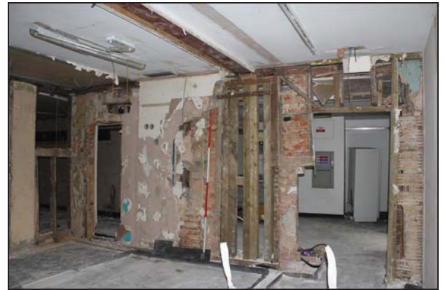
DP 70 East side of FF03 (north-east range) showing fragmentary survival of timber framing with much later replacement and removal, taken from the west
