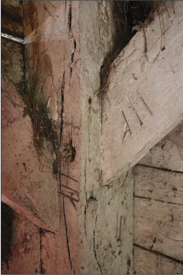
Plate 15 Detail of the north-west corner of Unit 4 showing assembly marks, taken from the south (DP 75)
