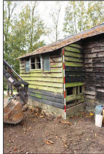
DP 14 Detail of the modern projection on the south-east side of Unit 6, taken from the east
