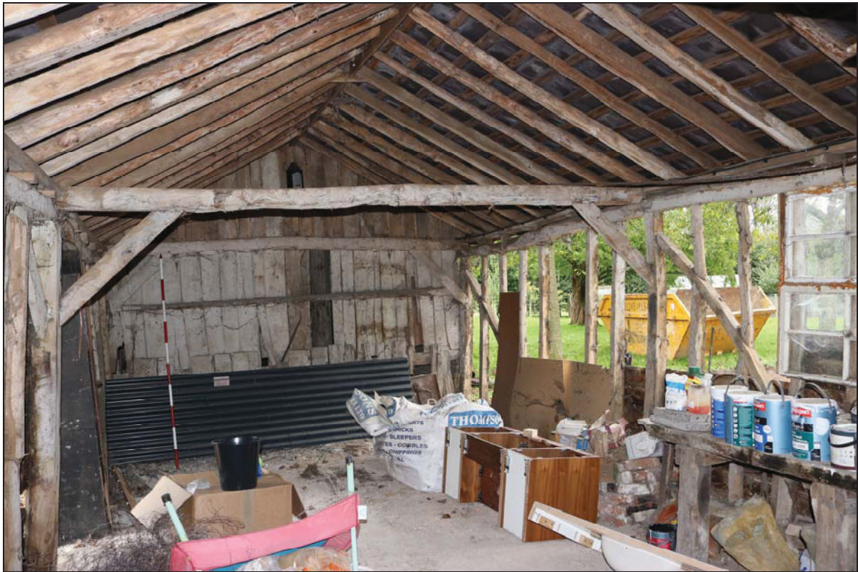
Plate 19 Interior of Unit 5 showing primary-braced framing on the right with the external weatherboarding removed, taken from the south-west (DP 79)
