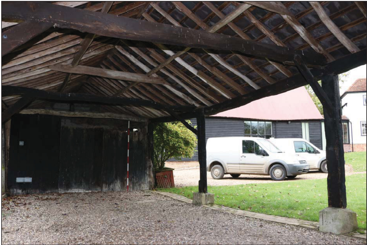
Plate 11 Open-fronted bays to the north-west of Unit 2, taken from the north-east (DP 43)
