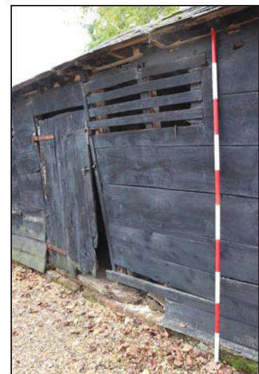
DP 18 North-west elevation (Unit 4) showing doorway with adjoining ventilation aperture and wide boarding, taken from the west
