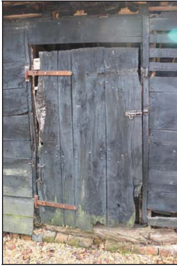
DP 19 North-west elevation (Unit 4) showing boarded door re-hung on the opposite side, taken from the north-west
