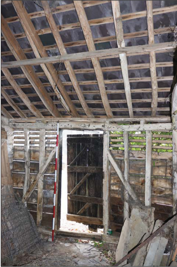
Plate 13 North-west wall of Unit 3 showing primary-braced framing with ledged and braced door and flanking ventilation apertures, taken from the south-east (DP 60)
