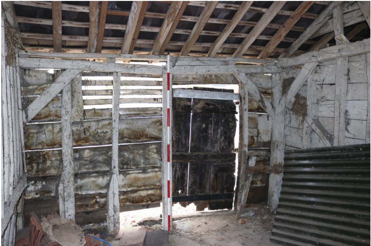
Plate 17 North-west side of Unit 4 showing lateral braces with infill studwork and door and ventilation aperture, taken from the south-east (DP 70)
