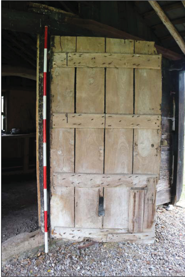
Plate 9 Rear face of the historic boarded and ledged door to Unit 1, taken from the south-west (DP 32)
