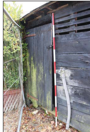
DP 16 North-west elevation (Unit 3) showing boarded door with later hinges, taken from the south-west
