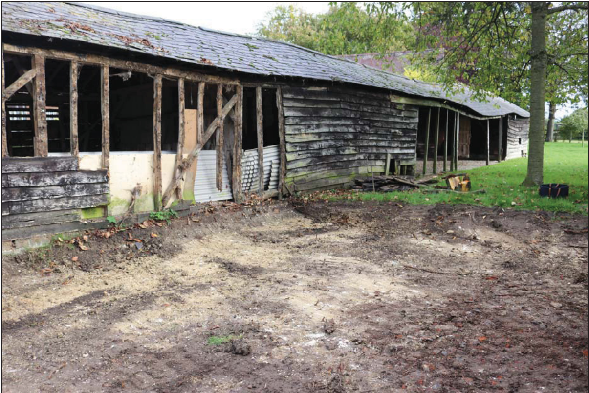
Plate 1 South-east elevation showing primary-braced framing (Unit 5) after removal of weatherboarding and open-fronted unit beyond (Unit 2), taken from the south (DP01)
