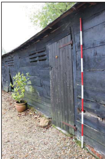
DP 23 North-west elevation of Units 4 and 5 showing fairly modern door set in the historic elevation, taken from the south-west
