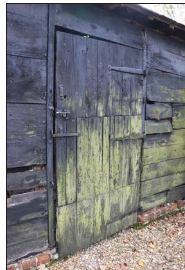
DP 24 North-west elevation of Unit 5 showing repaired and altered early boarded door, taken from the north
