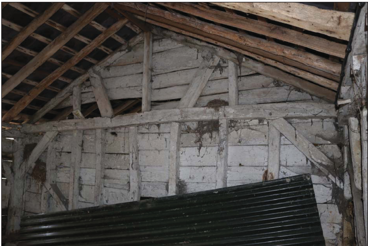
Plate 14 North-east side of Unit 4 showing studwork with horizontal boarding to the rear, taken from the south (DP 71)
