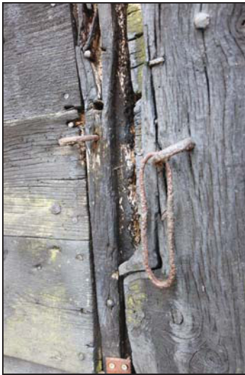
DP 21 Detail of the doorway on the north-west elevation (Unit 4) showing metal hasp and loop, taken from the north-west
