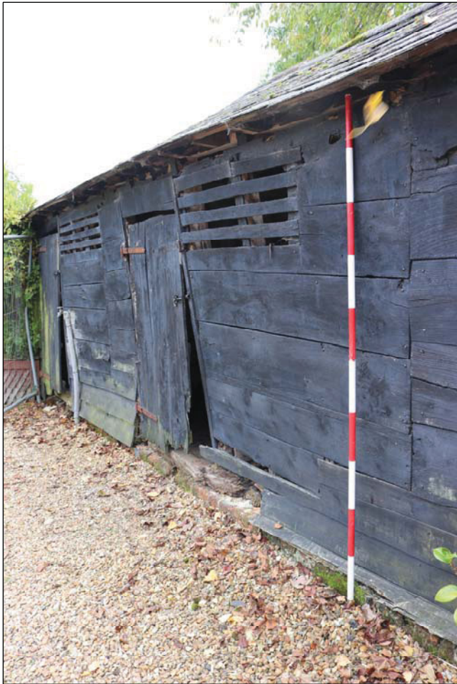
Plate 3 North-west elevation (Units 3 and 4) showing wide horizontal boarding with ventilation apertures, taken from the south-west (DP15)
