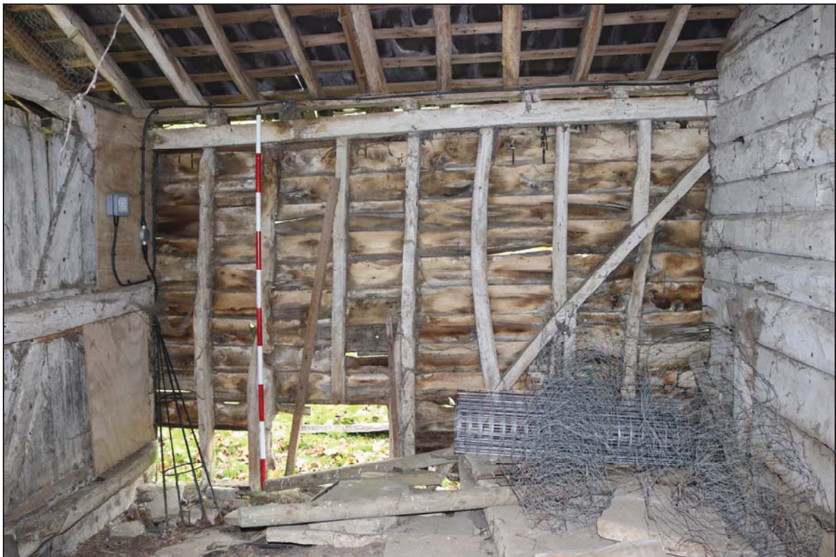
Plate 12 South-east wall of Unit 3 showing primary-braced framing, taken from the north-west (DP 57)
