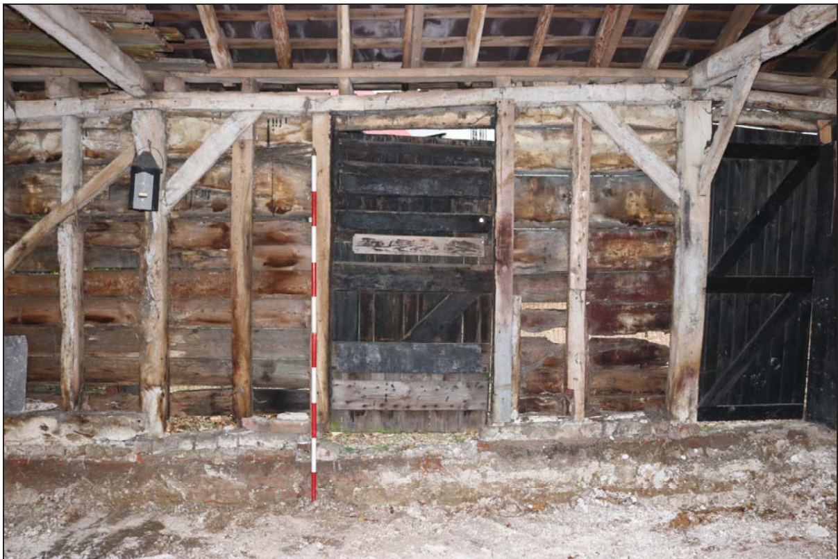
Plate 6 North-west wall of Unit 5 (central bay) after the lowering of the floor level, taken from the south-east (DP 116)
