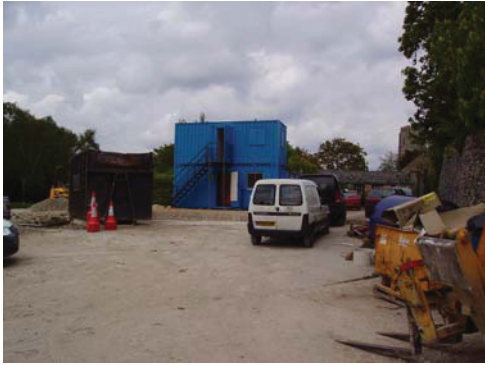
DP1 Eastern boundary of site and area of former hardstanding. From S.
