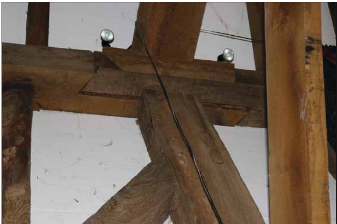
Plate 8 Scarf joint in the wall-plate at the bay divisions in Barn 1, taken from the south-east (DP 37)
