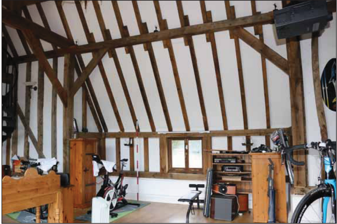
Plate 11 Outshut on the south-east side of bay 2 of Barn 1, taken from the west (DP 29)
