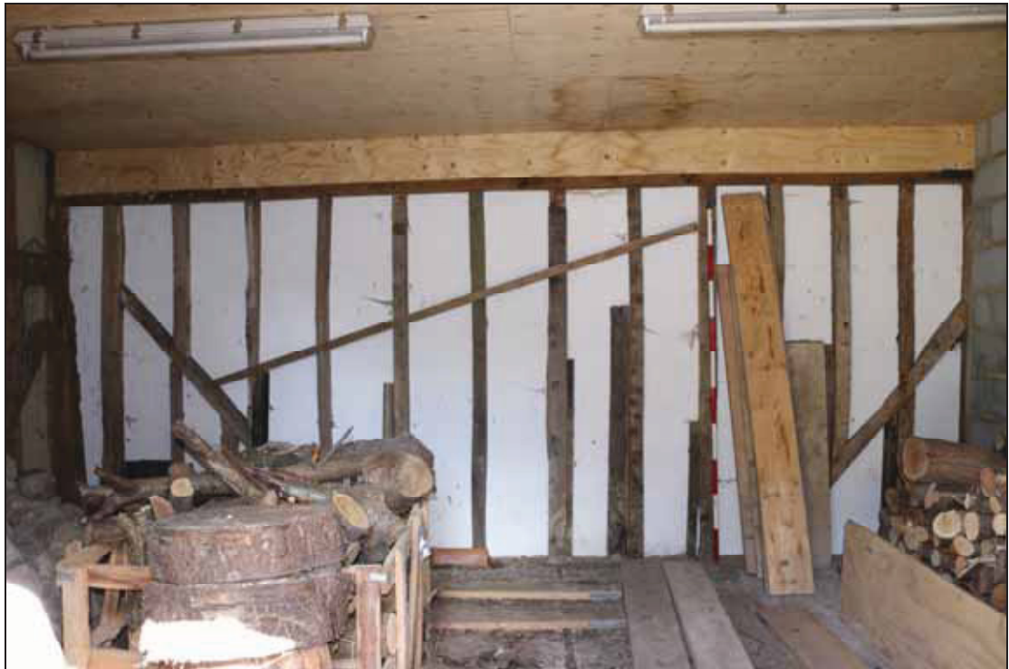
Plate 18 North wall of the west room of Barn 2's outbuildings, taken from the south (DP 16)
