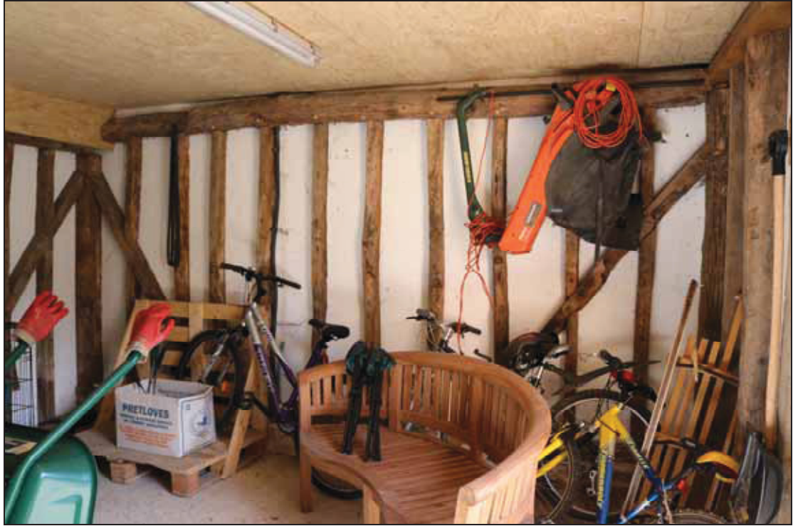
Plate 21 East wall of the east room of Barn 2's outbuildings, taken from the south (DP 24)
