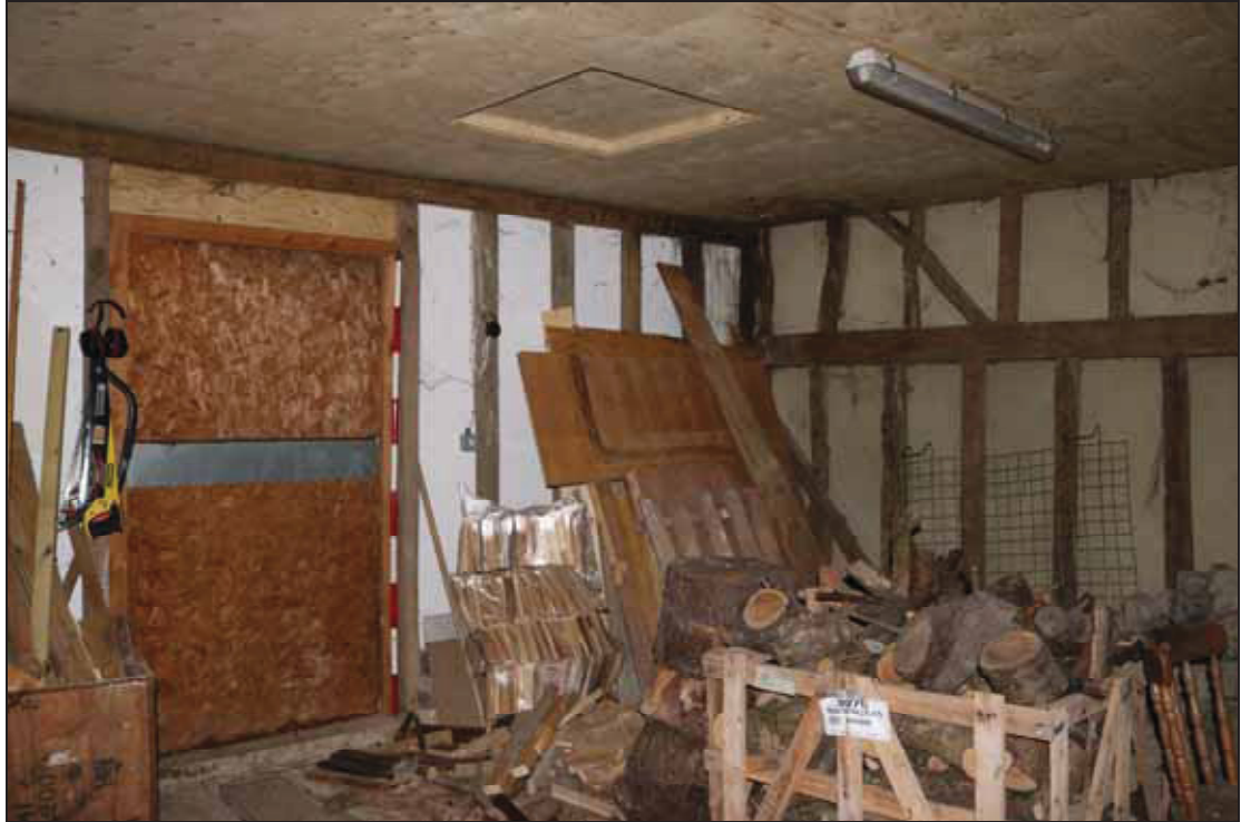
Plate 19 Interior of the west room of Barn 2's outbuildings, taken from the north (DP 19)
