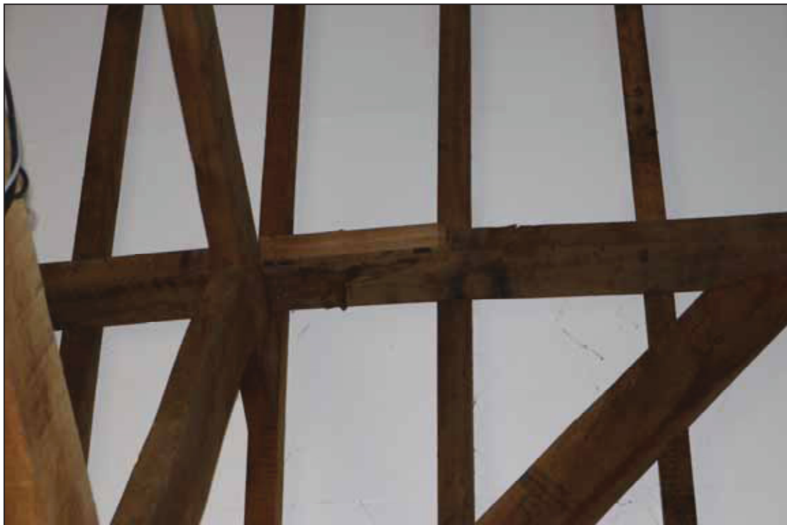
Plate 6 Scarf joint in the purlin at the bay division in Barn 1, taken from the west (DP 43)
