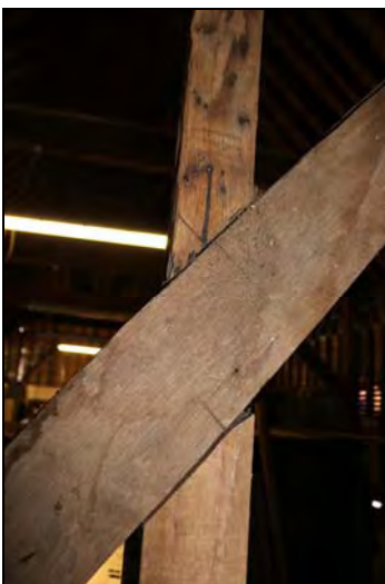
DP 104 South elevation showing primary brace and stud with chiselled assembly marks and setting out line, taken from the south
