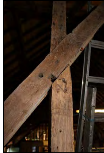
DP 101 South elevation showing primary brace and stud with chiselled assembly marks exposed during the monitoring, taken from the south
