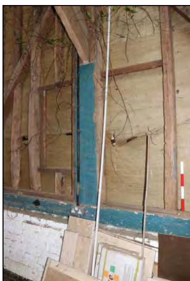
DP 65 Apertures inserted into the east side of Bays 4 and 5 (barn), taken from the west
