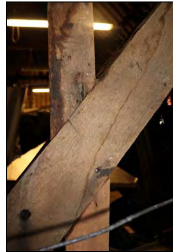
DP 103 South elevation showing primary brace and stud with chiselled assembly marks and setting out line, taken from the south
