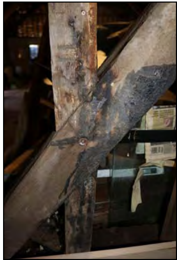
DP 102 South elevation showing primary brace and stud with chiselled assembly marks exposed during the monitoring, taken from the south
