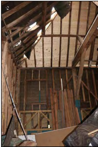
DP 61 West wall of Bay 5 (barn) showing inserted aperture, taken from the east
