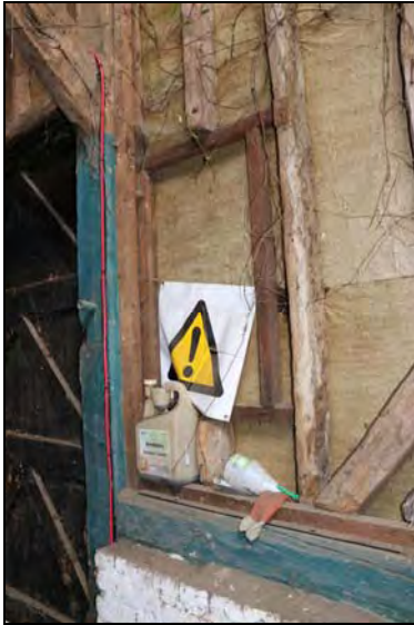
DP 55 Aperture inserted into the east side of Bay 4 (barn) framed in modern flimsy timbers, taken from the west
