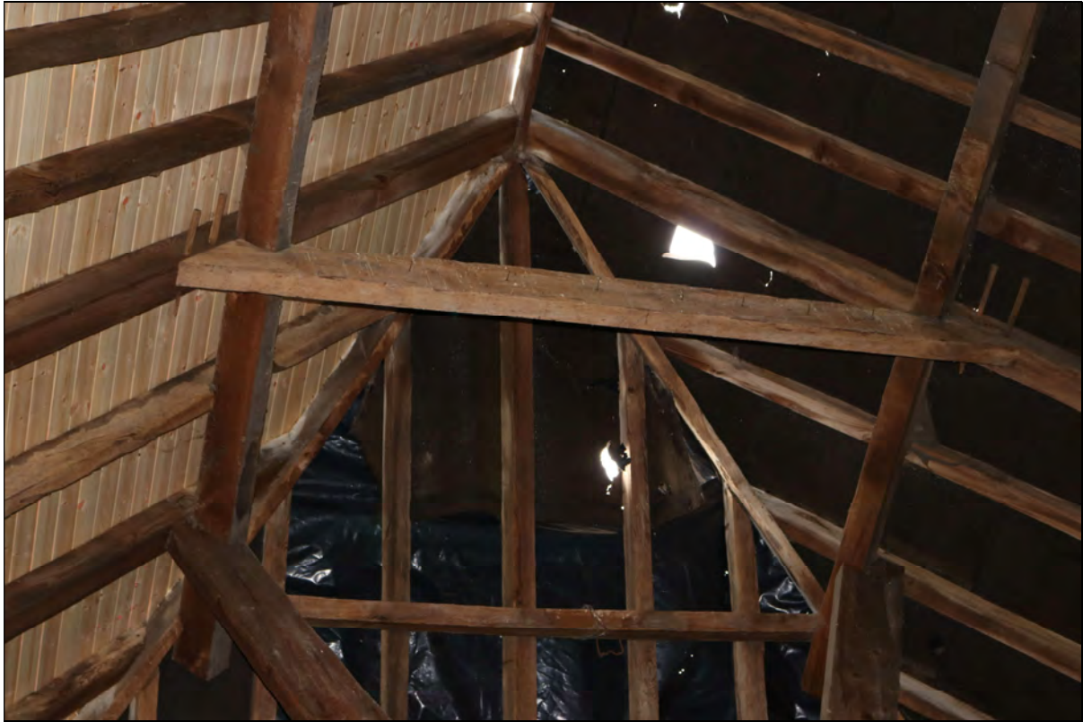
Plate 9 Detail of the north roof hip (barn) showing detail of the hip truss with pegged collar, taken from the south (DP 46)
