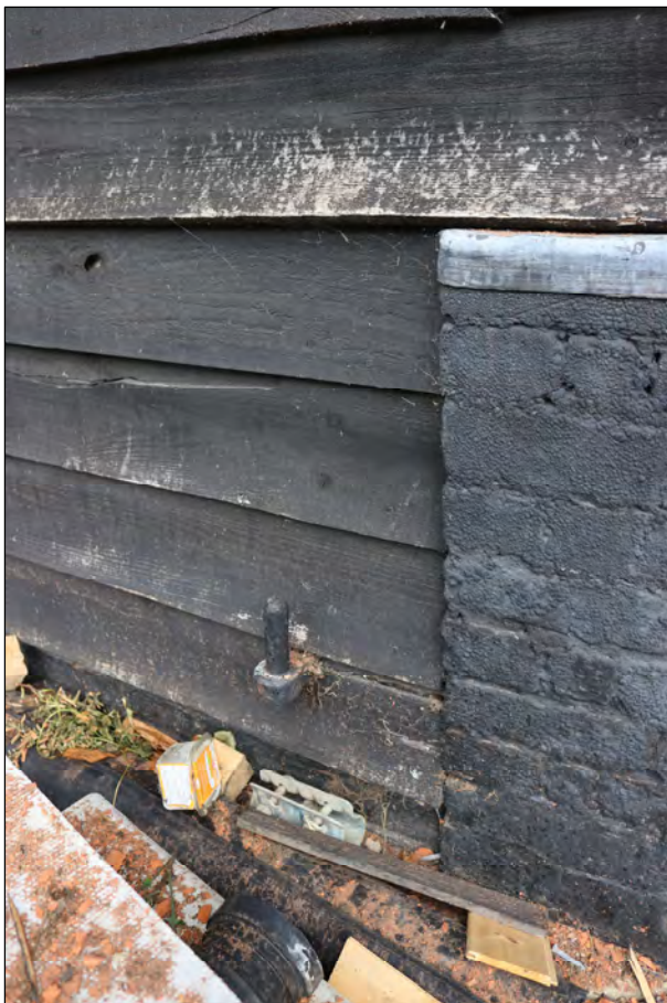
Plate 4 West side of the central bay (barn) showing pintle for former threshing door, taken from the south-west (DP 6)
