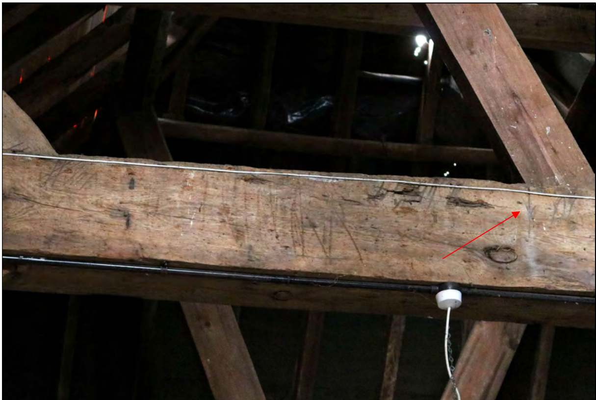
Plate 10 Edge of the tie-beam (barn: Truss 2) showing scribed Baltic timber marks including the mark for Gdansk (indicated), taken from the south (DP 71)
