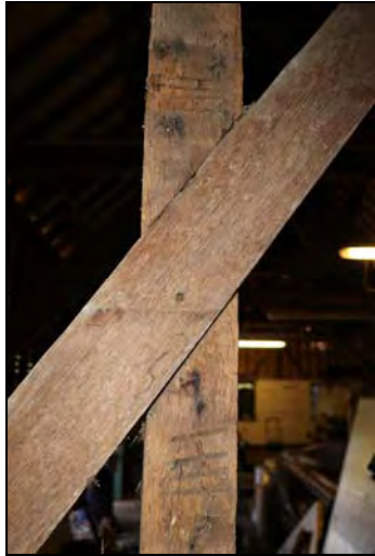
DP 100 South elevation showing primary brace and stud with chiselled assembly marks exposed during the monitoring, taken from the south
