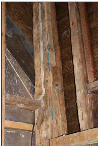
DP 63 Detail of the south-west corner post showing evidence for reuse, taken from the north-east
