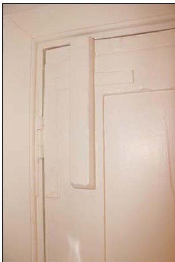
DP 35 Detail of the rear face of the historic door showing H-L hinges, taken from the south-east
