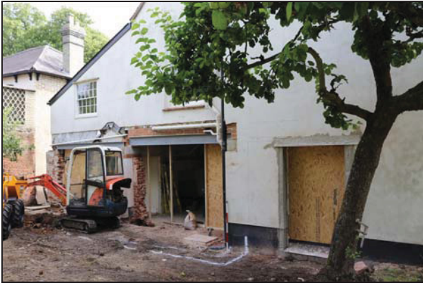
DP 1 West side of the building following removal of external walls at ground floor level, taken from the south-west
