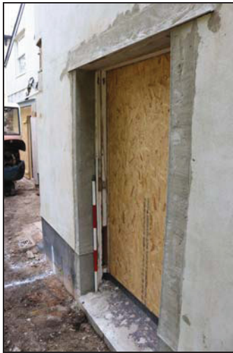
DP 3 Enlarged opening to take the reused eight-over-eight sash window, taken from the south-west
