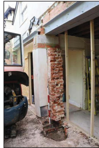
DP 4 West side of the central rear range following the removal of the external wall leaving a brick pier on the north, taken from the south-west
