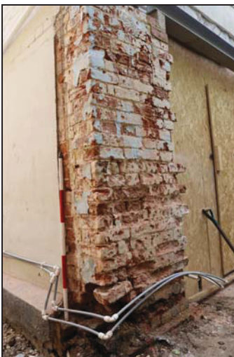
DP 5 North-west corner of the northern rear range showing exposed brickwork, taken from the north-west
