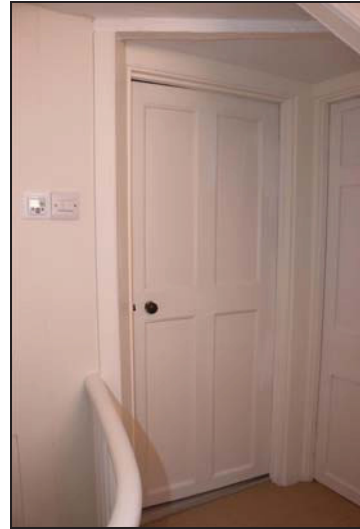
DP 32 Historic door at second floor level (southern range), taken from the north
