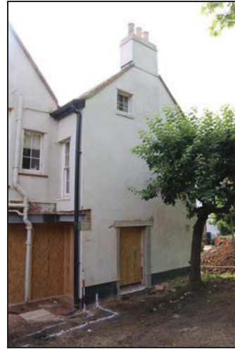
DP 2 West gable end of the southern rear range, taken from the north-west
